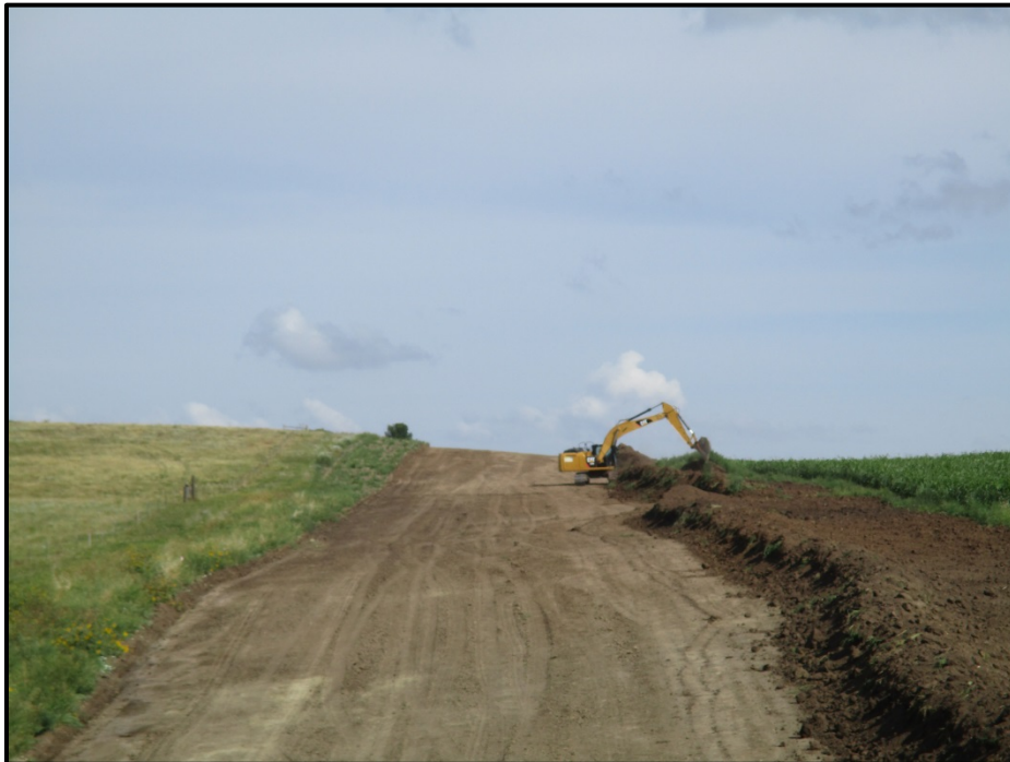
Photo 10. (GPS Point #454) – Excavator/hoe moving topsoil pile out from the edge so dozer can come through and spread topsoil on ROW. Direction: North.
