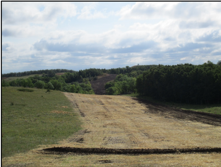
Photo 8. (GPS Point #453) – Water bar shown at the bottom of the photo. Travel lane still being used on the right side of the ROW to get to the hill in the background. The hill in the background was rocky and has not yet been seeded. Direction: East.
