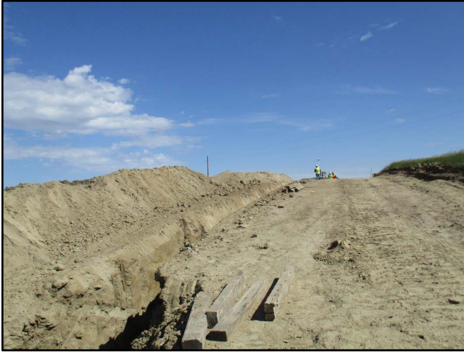
Photo 3. (GPS Point #434) – Survey crew (shown at top of hill) came in after pipe was laid to survey for the as-built (pipe welds and depths). Direction: North.
