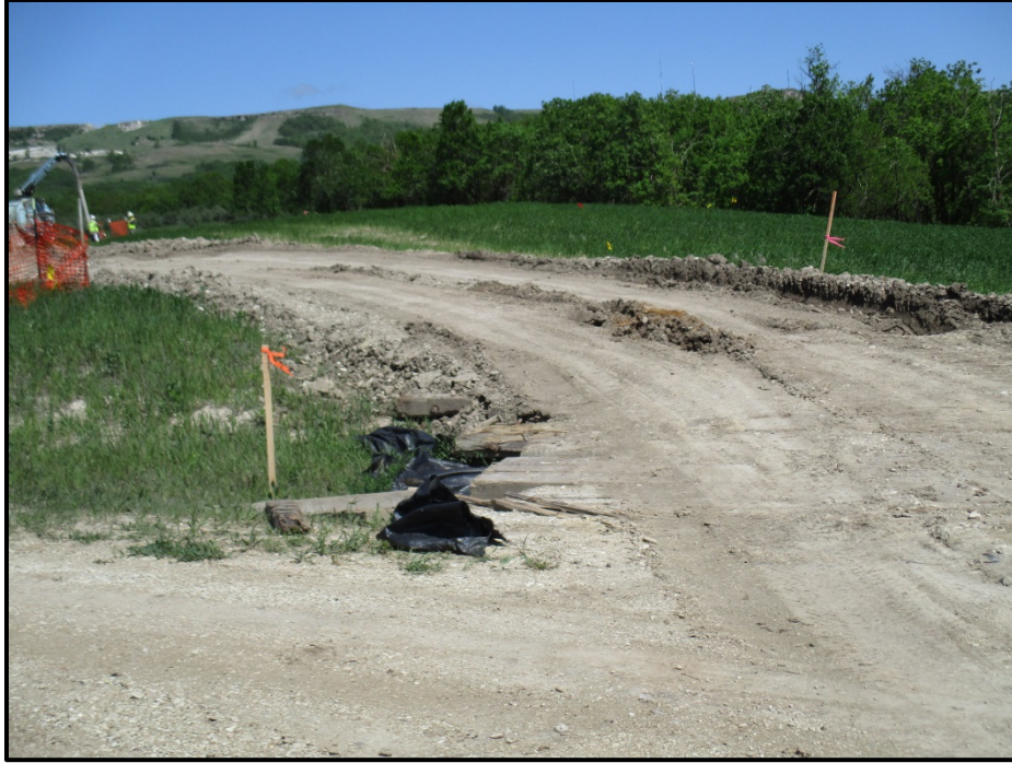
Photo 5. (Near GPS Point #435) – Many of the swamp mats on site were laid over a tarp, which prevents the mat from being buried when driven over.
