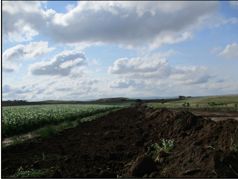
Photo 11. (GPS Point #454) – Topsoil pile moved from edge of ROW closer to the center of ROW. Direction: South.
