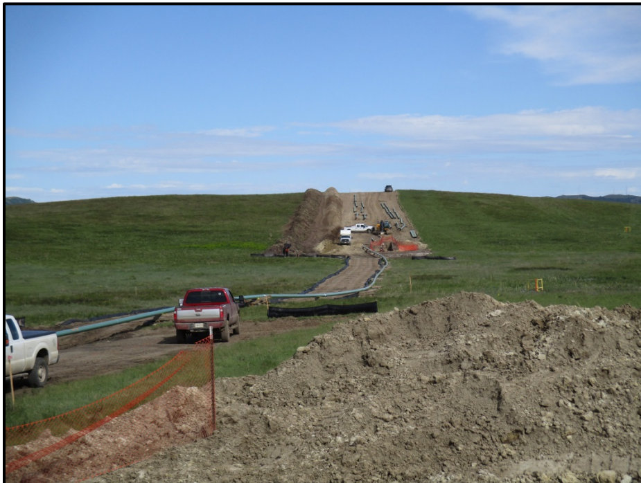
Photo 6. (GPS Point #432) – Near bore tie-in area showing fence along bell-holes. Swamp mats are visible in center of photo, used to cross low area/drainage. Silt fences were in place along edges of ROW in low areas. Contractors stated that the open trench was not open for more than 3 days.
