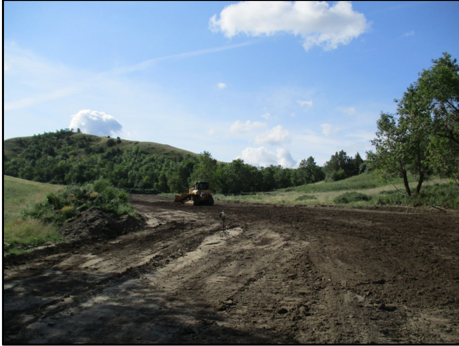
Photo 13. (GPS Point #455) – Dozer pushing sediment up the hill and smoothing out the area from a rain event. Pipe test lead with metal stake shown in the middle left of ROW. Direction: South.
