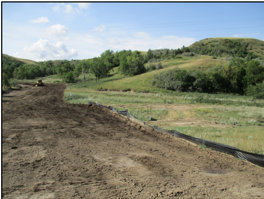
Photo 12. (GPS Point #455) – Rain event washed some sediment down the hill and was caught in silt fence. Dozer pushing some of the sediment back up the hill. Direction: South.
