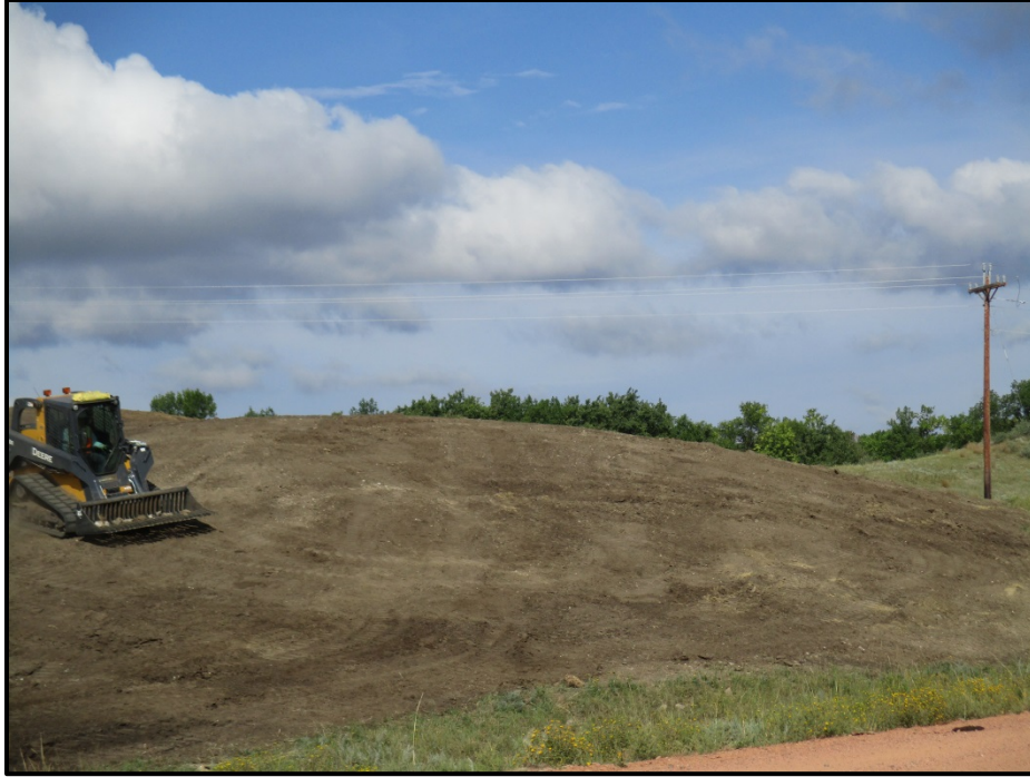
Photo 9. (GPS Point #453) – ROW still needs to be fine graded, seeded and crimped. Direction: West.
