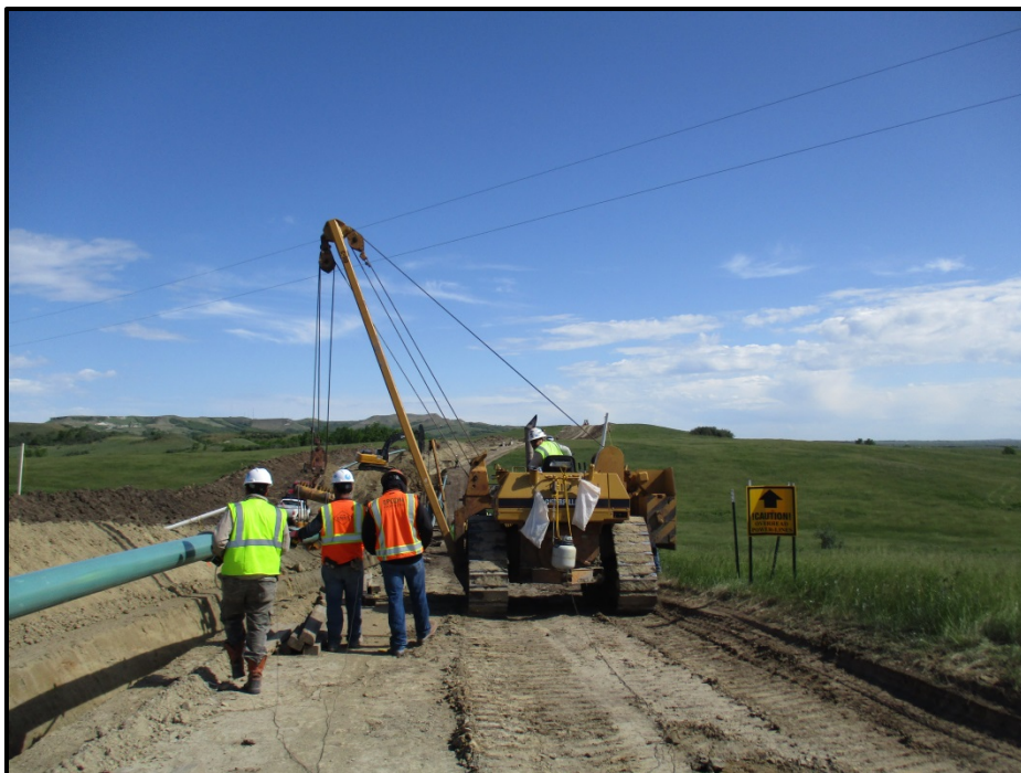
Photo 2. (GPS Point #434) – Contractor lowering pipe into trench. There is a “Caution Overhead Power-Lines” sign on the far right of the ROW. Direction: North.
