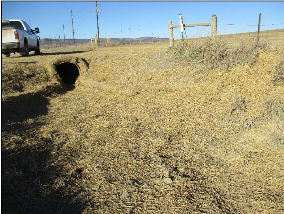
Photo 2. (GPS Point #495) – Approach to field/pipeline ROW from road. Area has fence with gate, pipeline marker, culvert, straw wattles, and mulch.
