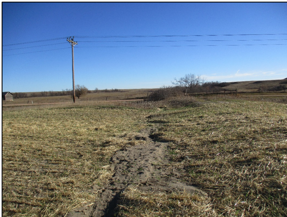
Photo 4. (GPS Point #497) – This area had some sedimentation and rills forming (erosional features) within the pipeline ROW. The area was sandy. While on-site the ONEOK representative called their reclamation team to come address the problem. Direction: East.
