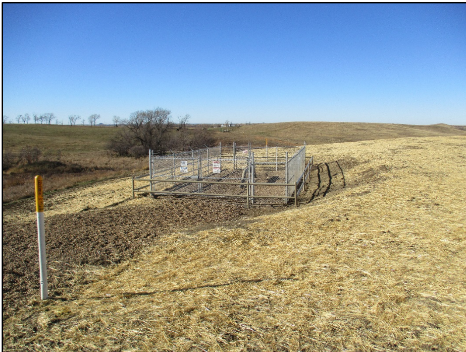
Photo 10. (GPS Point #502) – Pipeline ROW with fenced in block valve. Pipeline marker to the left of photo, area has been mulched and seeded. Direction: West.
