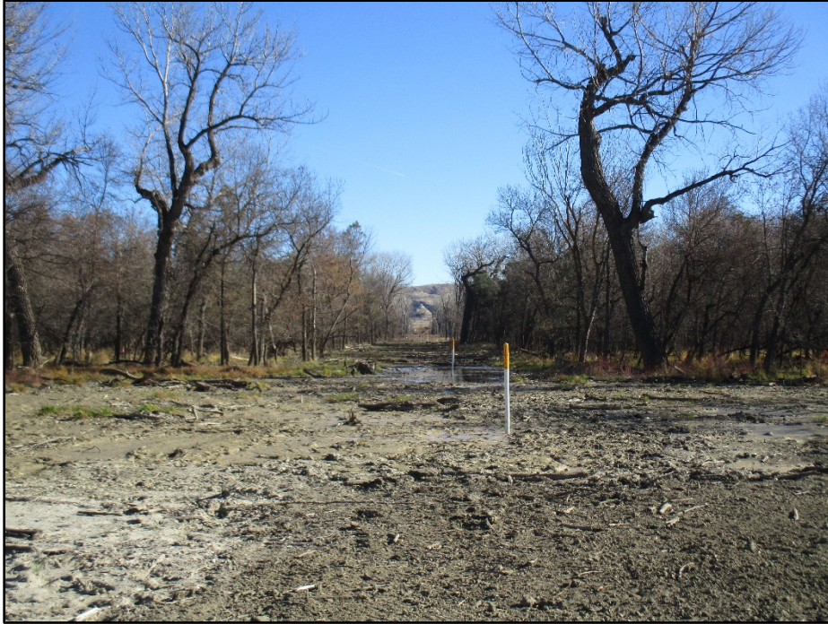
Photo 13. (GPS Point #503) – River bore location. Pipeline markers go through riparian area. Trees and shrubs were removed. Direction: East.
