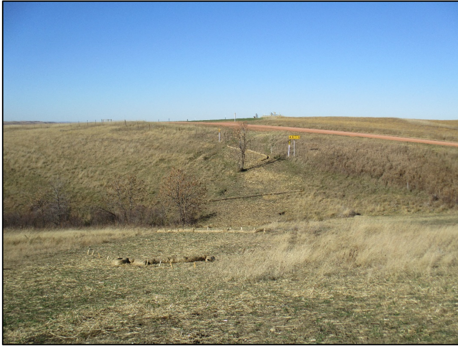
Photo 19. (GPS Point #505) – Pipeline ROW on state land with straw wattles for erosion control. Direction: Northwest.
