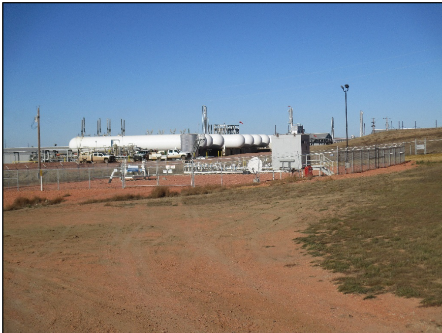
Photo 24. (GPS Point #507) – End of the pipeline, this is where it ties into the Targa NGL Pipeline. Direction: Northwest
