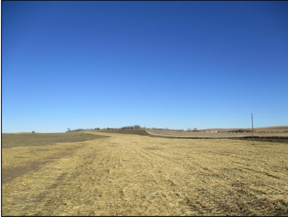
Photo 1. (near GPS Point #495) – Pipeline ROW, contours appear adequate. Area has been seeded and mulched. Direction: North.
