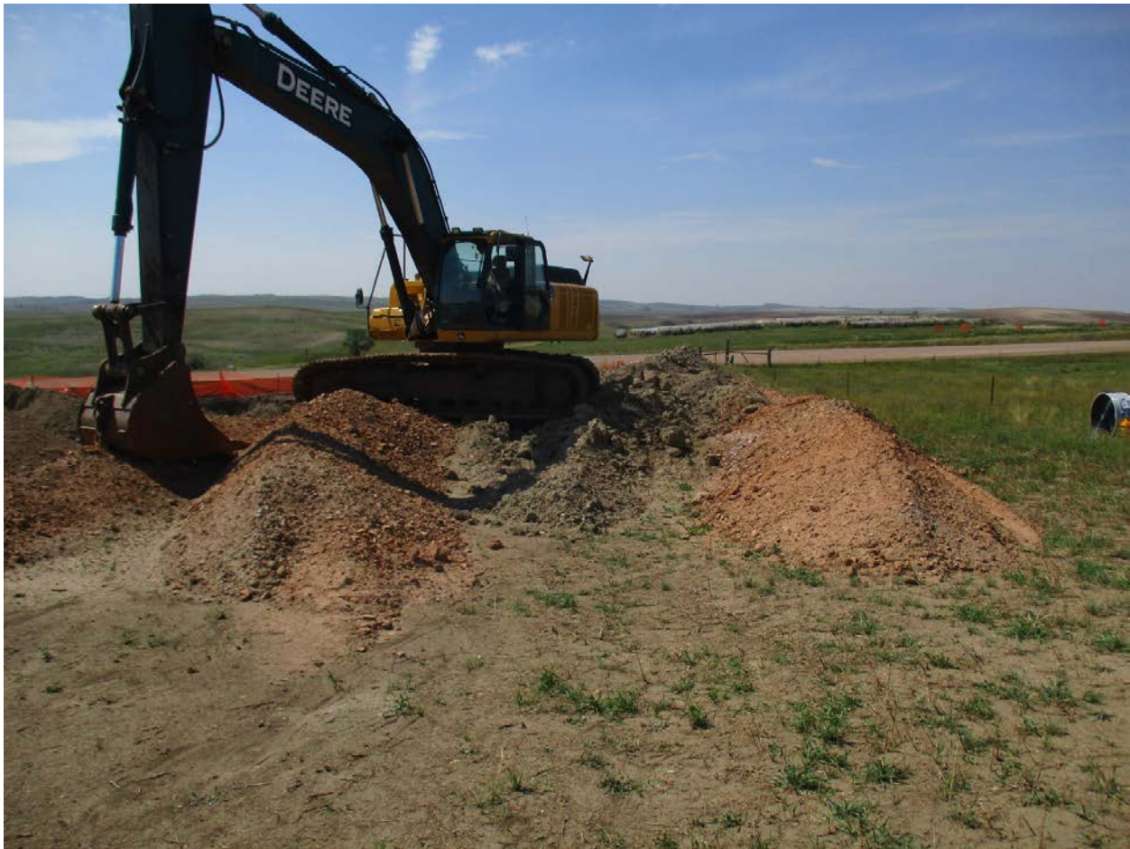
Photo 18. (Point 546) Facing: West. View of the equipment and spoil piles at the line strike site. The photo shows mixing of scoria piles with subsoils. This work was completed by a contractor for rural water, not ONEOK. No topsoil piles were visible in the area.
