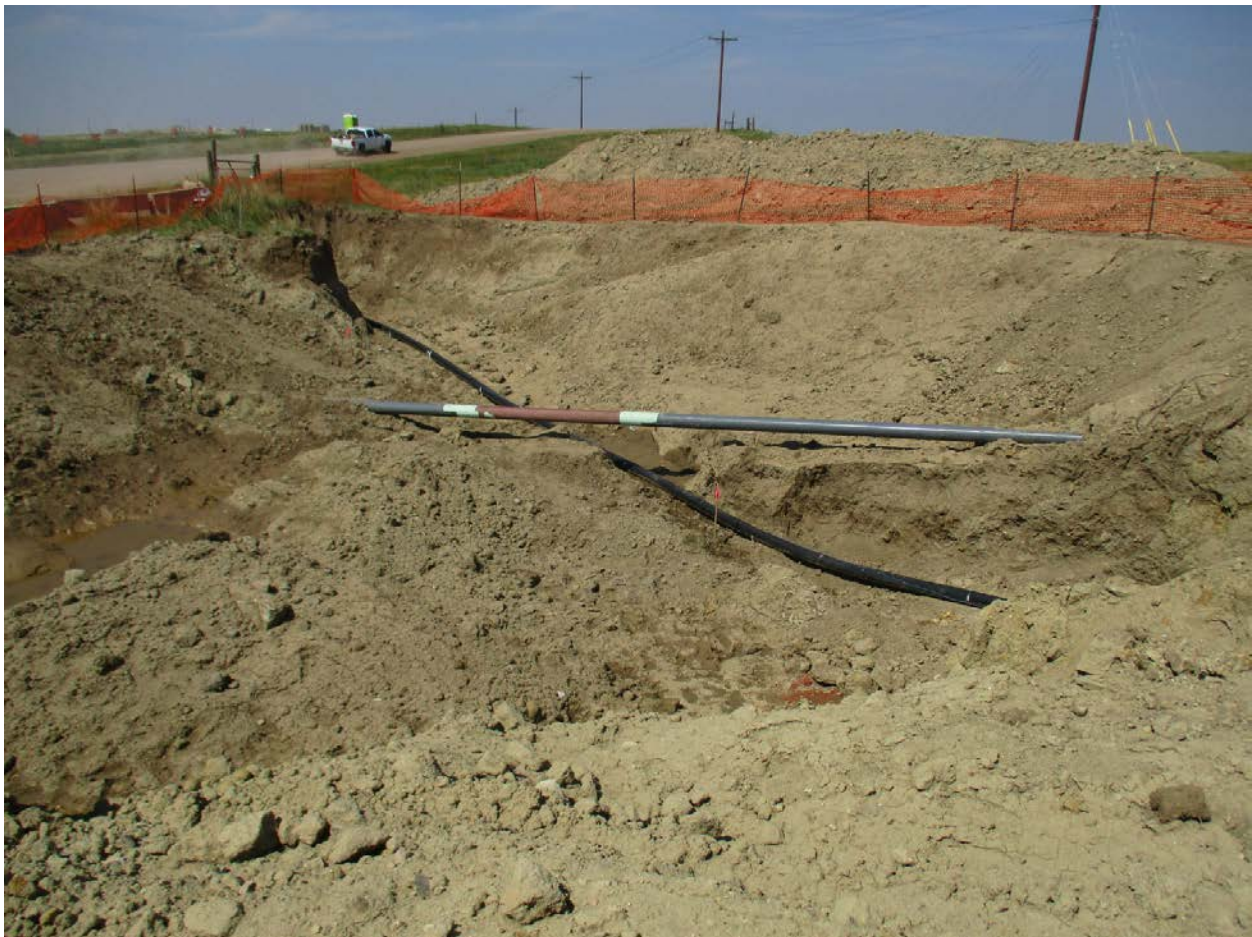
Photo 17. (Point 546) Facing: North. The area excavated to repair the recent line strike and remove contaminated soils. The Bear Creek NGL Line is the gray-colored steel line; the strike repair is the reddish brown portion bounded by white bands. The rural water line is the black polyline below the NGL line and at an angle in the photo.
