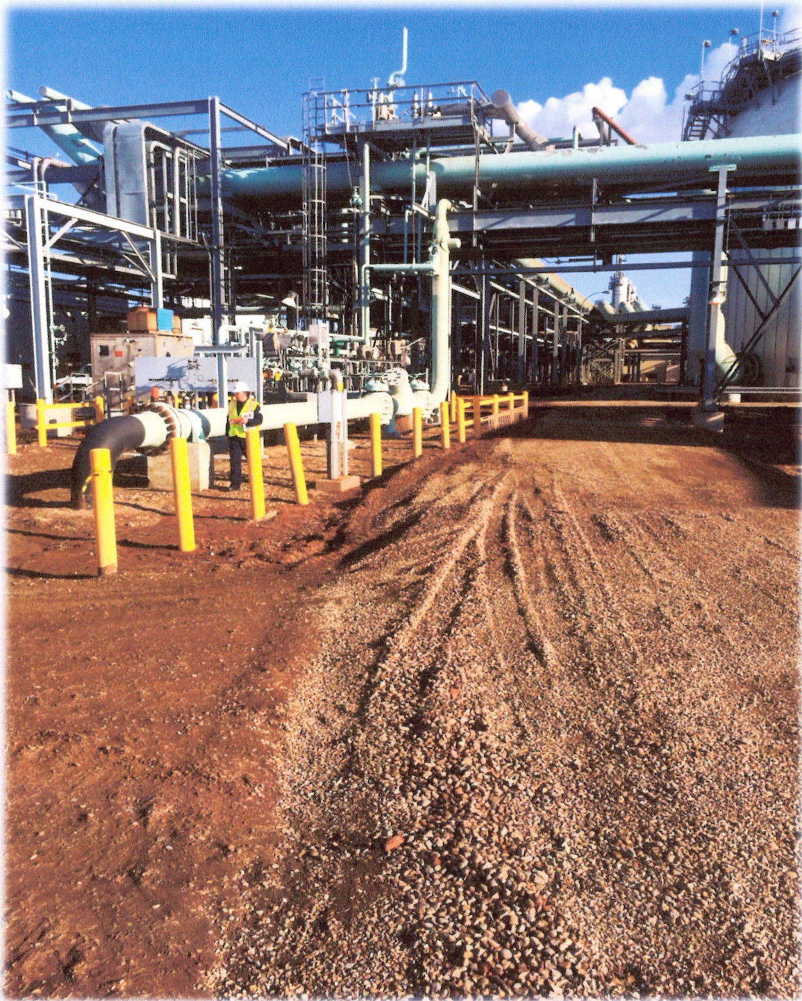
Figure 3: Section of the survey corridor located within the Plant. Note existing pipeline on the western side of the right-of-way. Photo taken from the center of the APE, view to the North.
