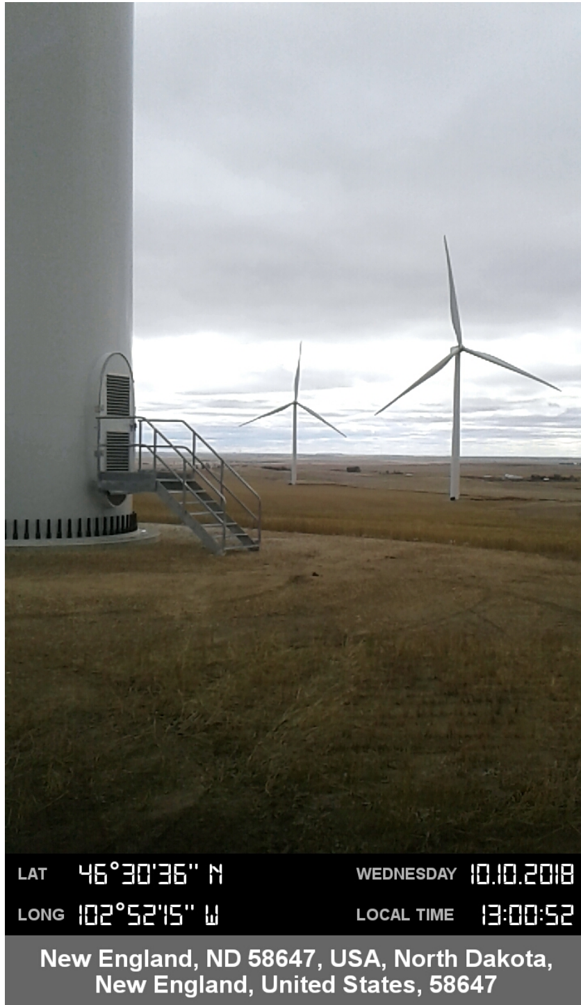
Report Photo #3: Overview of turbine construction block (T38) view to South Southwest.
