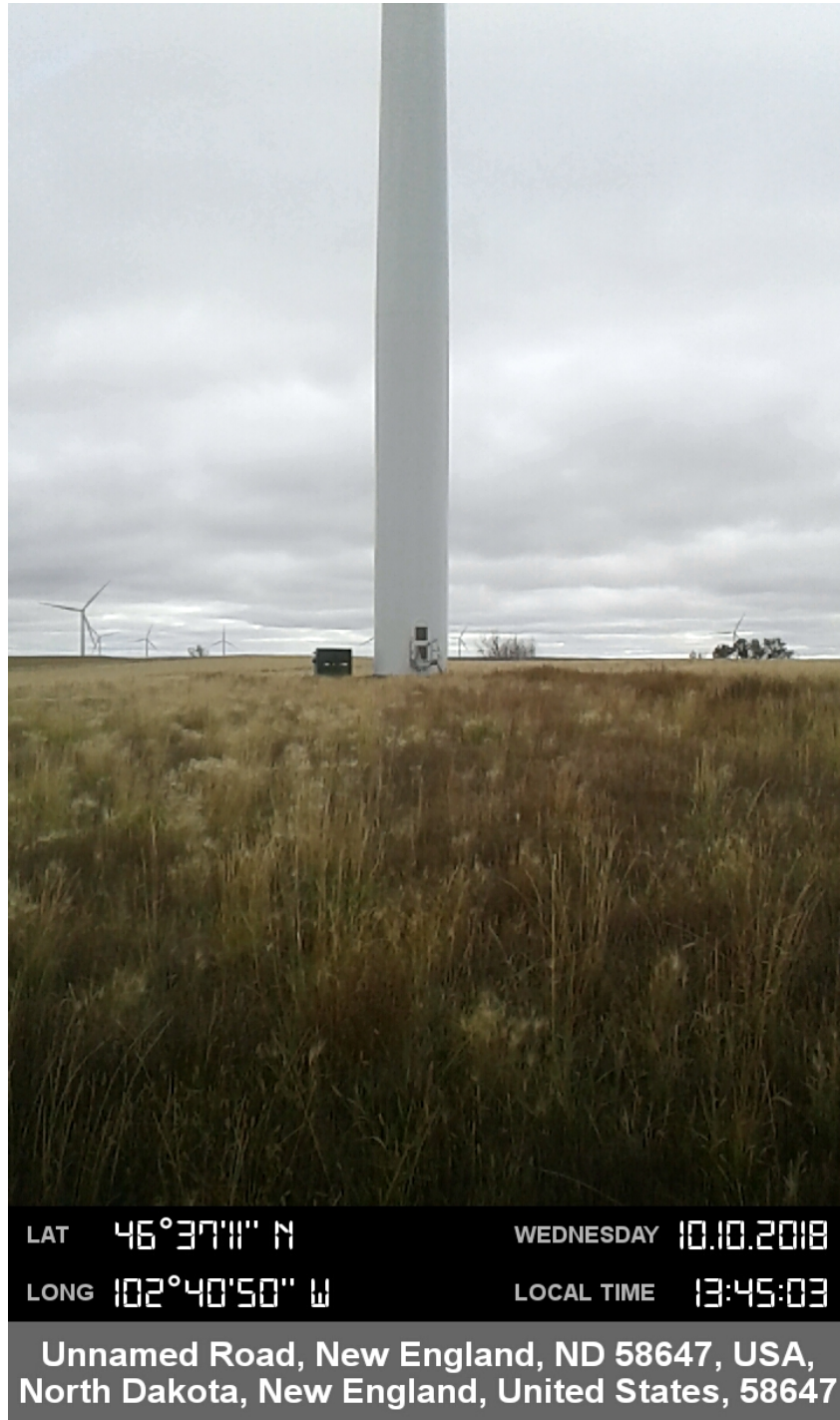
Report Photo #5: Overview of turbine construction block (T56) from North to South.
