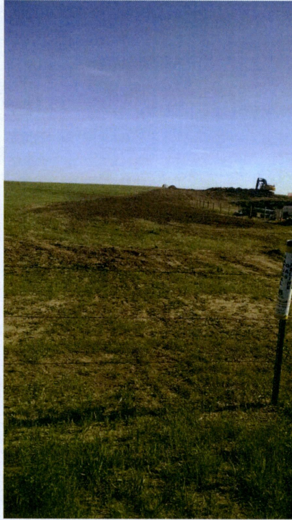
Photo 114: At 34th Street, looking South at completed right-of-way with fence back in place
