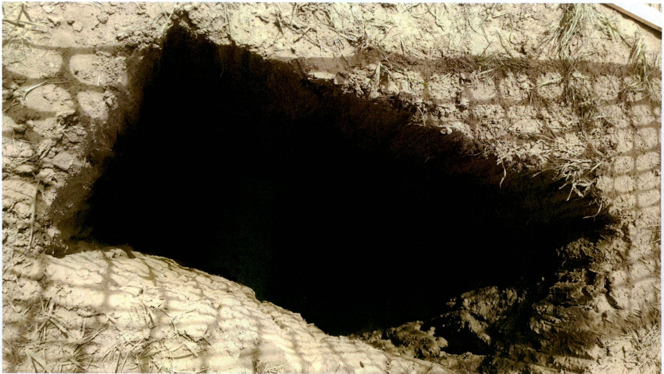
Photo 10: Station 1742+75.10, pot hole showing crude pipe with 59" cover
