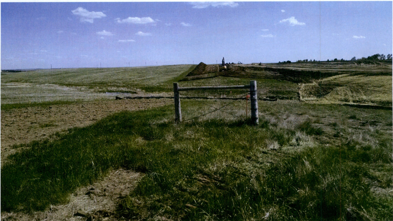
Photo 50: Station 1715+87.29, Looking South at stake by old fence, back hoe digging bell hole for end of bore in the distance
