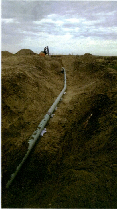
Photo III: Station 36+91.76, Looking North at tie-in from mainline to reroute, mainline dug out to lower pipe
