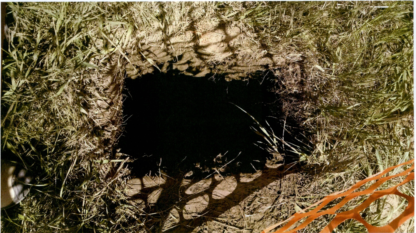
Photo 16: Station 4+00, pot hole showing 1/2\" consolidated cable with 26\" cover
