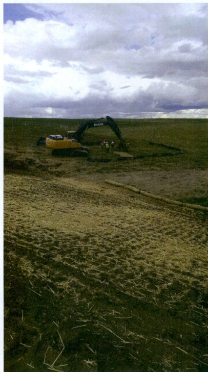
Photo 96: Station 8+91, frac out while drilling bore
