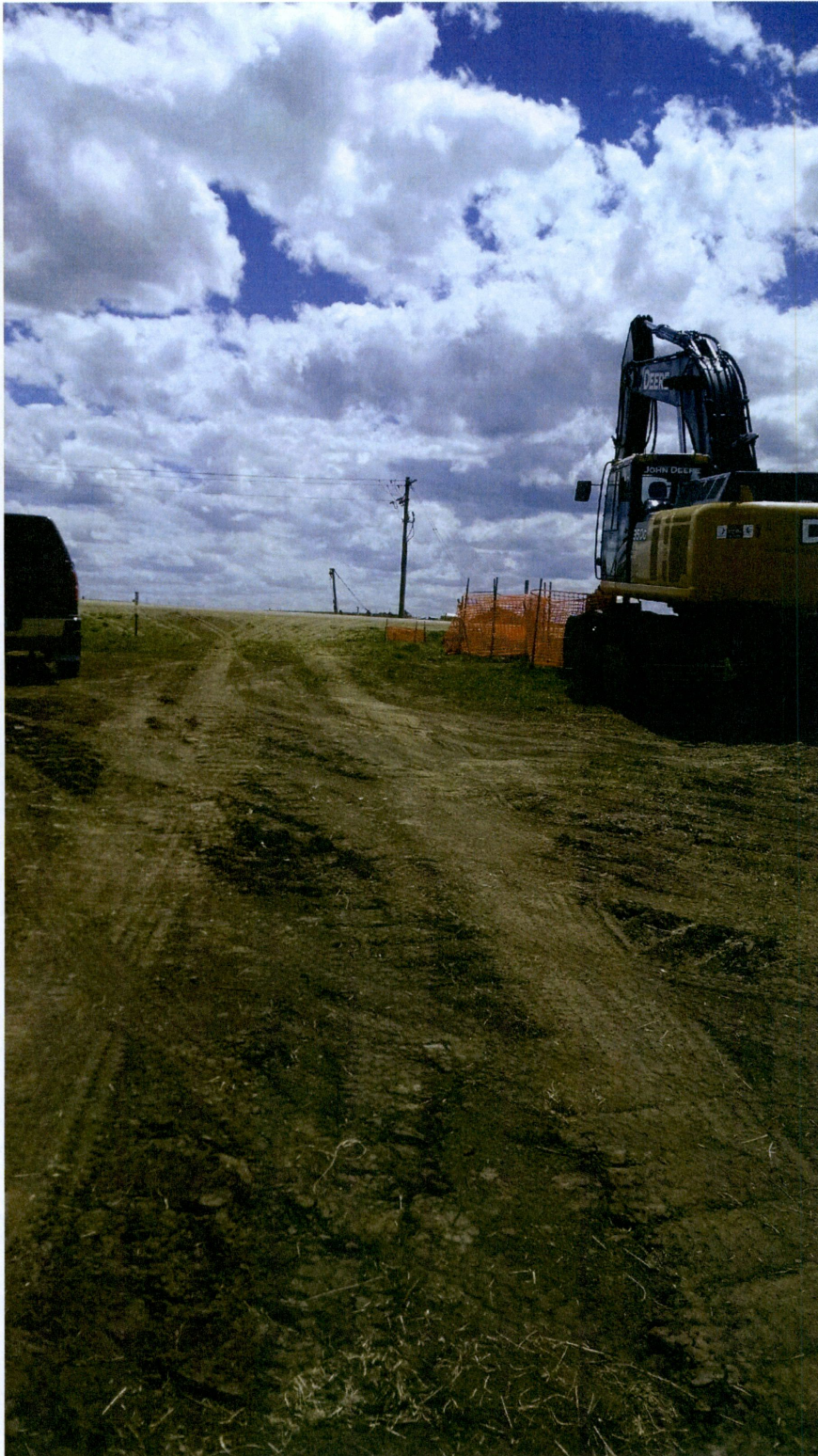
Photo 85: Station 7+94, 7+86, & 7+37, pot holes
