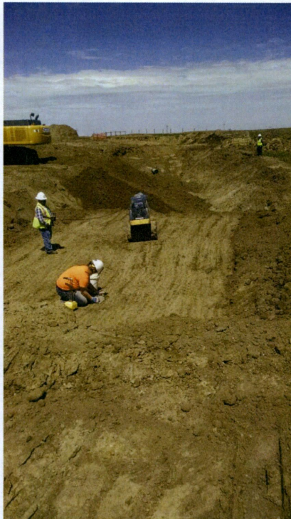
Photo II2: Station 36+91.76, Looking North at tie-in from mainline to tie-in, compacting soil and getting density checked to 90%
