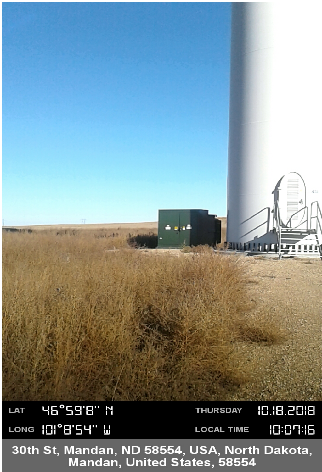
Report Photo #7: Overview of turbine construction block (T30) from South to North.
