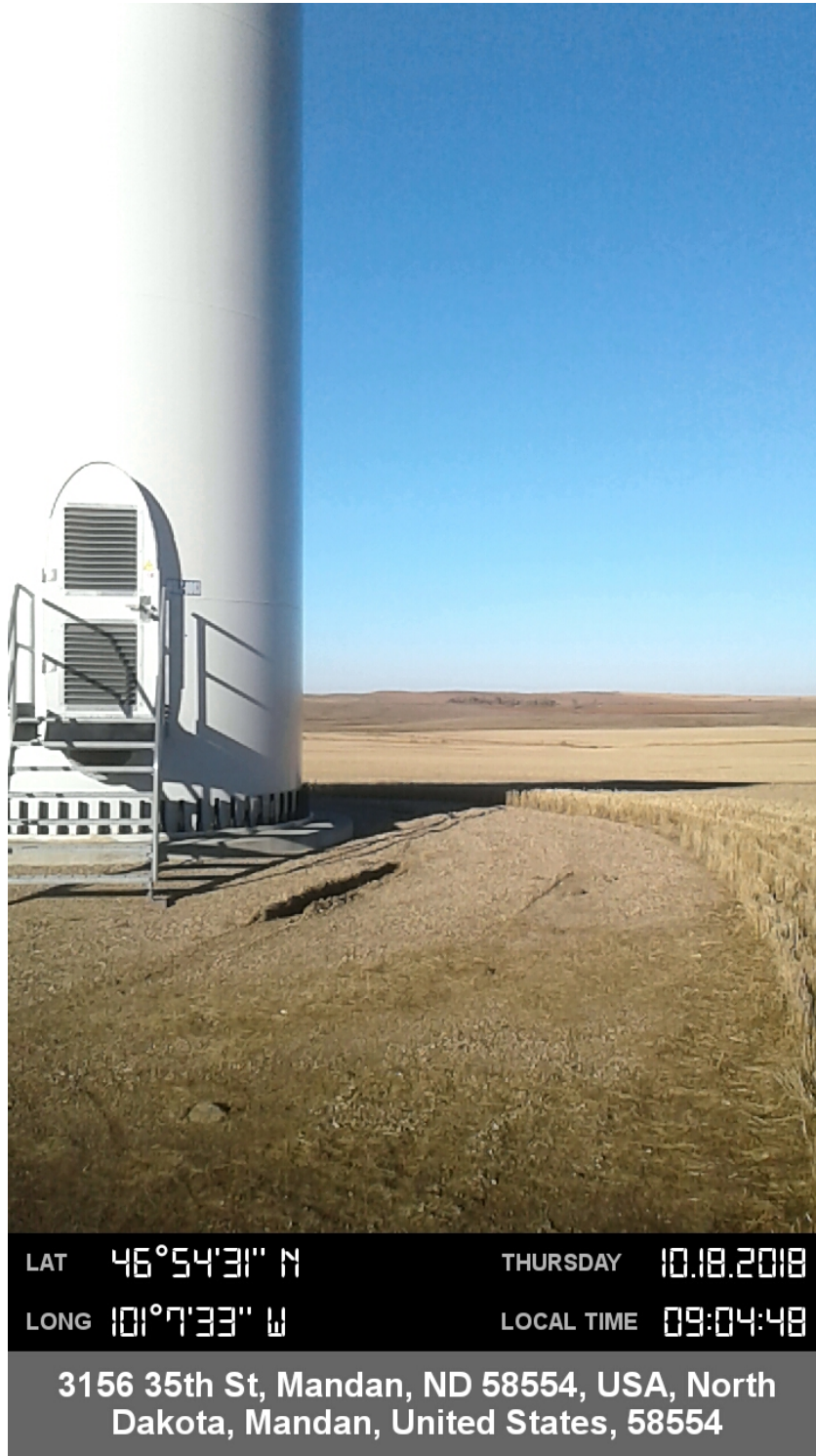
Report Photo #4: Overview of turbine construction block (T3) from South to North.
