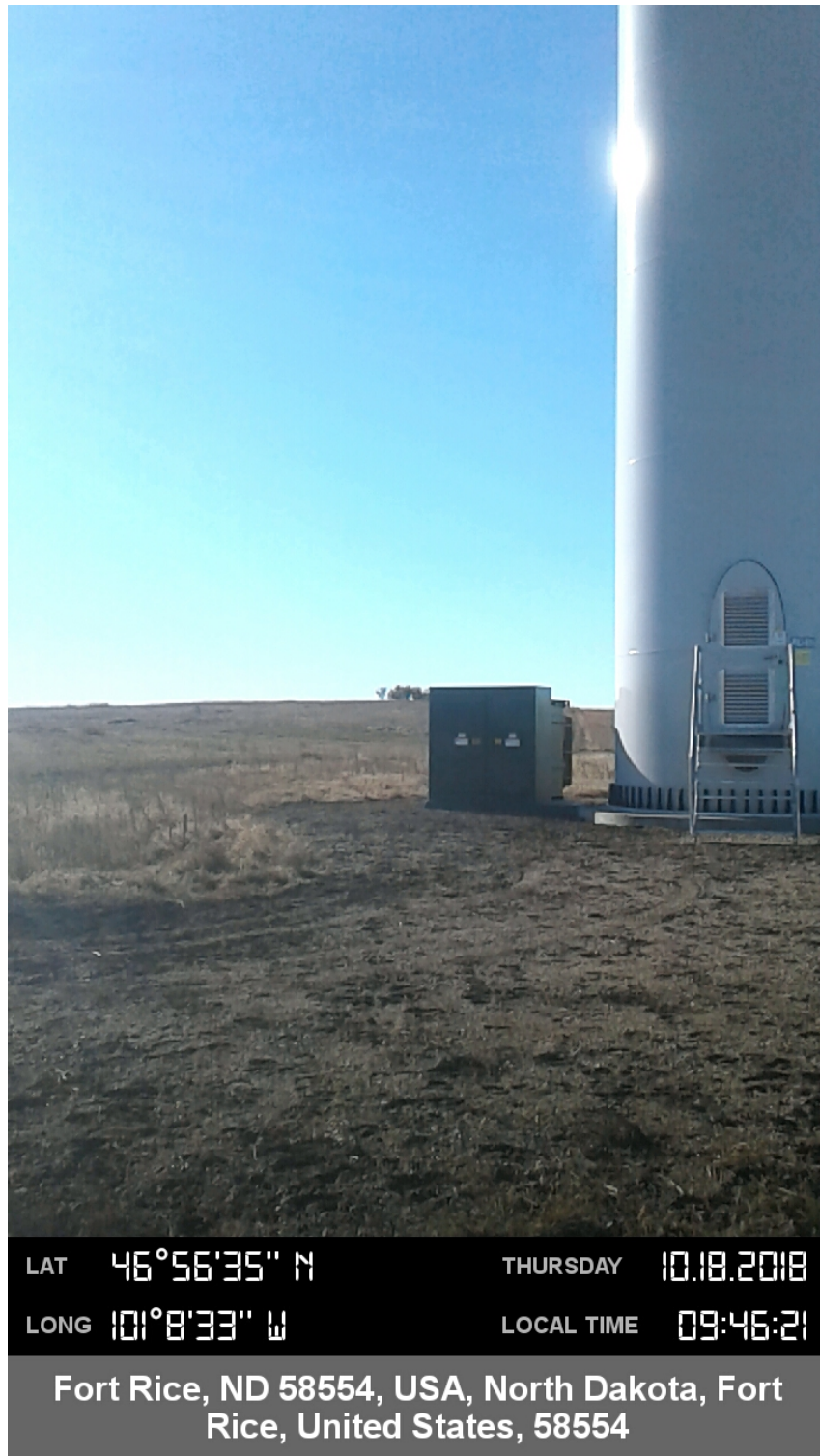
Report Photo #6: Overview of turbine construction block (T14) from South to North.
