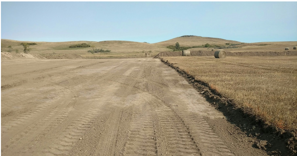
Photo 2: Located at station PI 2+60.02, showing Right of Way graded and heading west, then turning north. Photo showing stripped Right of Way at approximate depth of 12 inches. Topsoil is shown on edge of Right of Way beyond.
