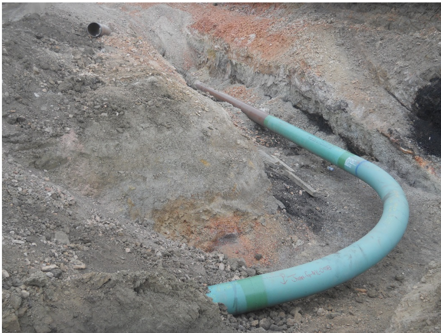
Photo 6: Located at station PI 25+09.66, looking west with pipe in trench and then turning south. Photo shows trench needs to be backfilled and regraded. Clean up across Right of Way needs to be done also.
