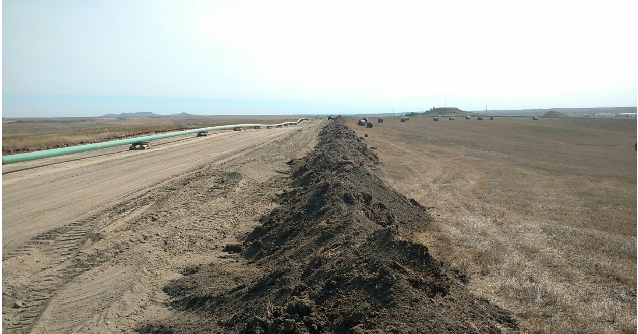
Photo 11: Located at station 54+00, looking west. Photo showing graded and stripped Right of Way. Topsoil is located on the right edge of Right of Way. Subsoil located on left side of topsoil. Both soil types are segregated and separated. Pipeline is welded and setting on skids ready for trenching.
