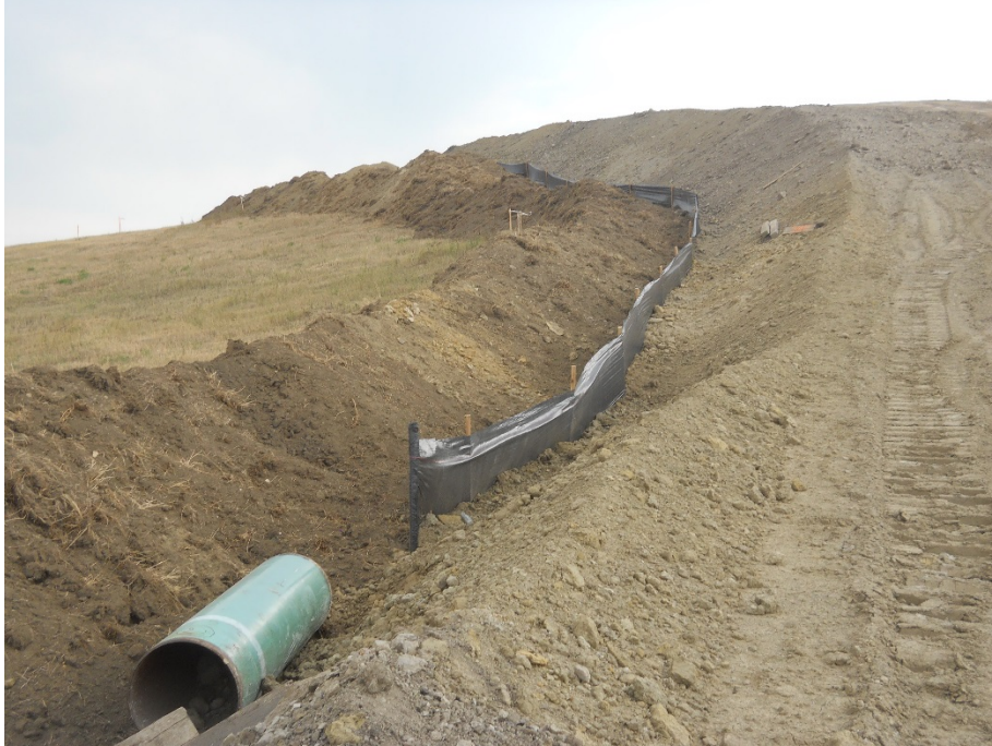
Photo 19: Located at station 69+00, looking southwest. Photo showing BMP silt fence placed between topsoil pile and subsoil pile. Clean up not done. Silt fence to prevent soil types from touching.
