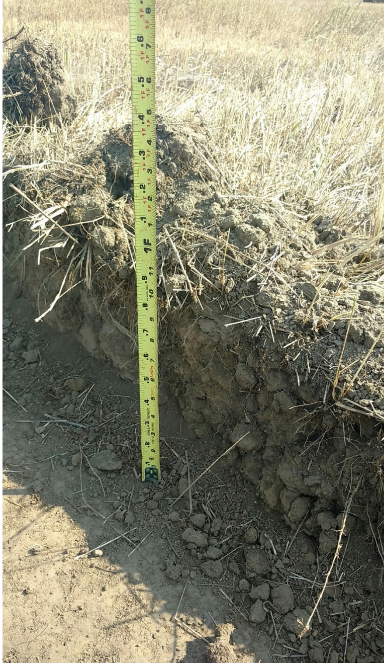
Photo 5: Located at station 21+00, photo showing stripped Right of Way at approximate topsoil depth of 12 inches. Photo is showing west side of Right of Way edge.
