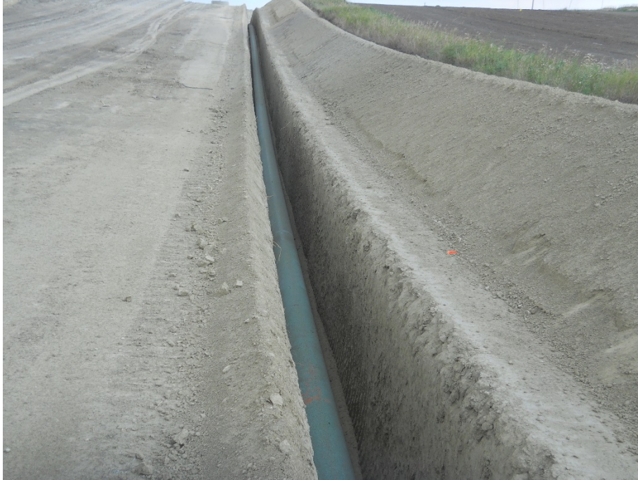
Photo 25: Located at station 96+00, looking west. Photo showing graded Right of Way graded with pipe installed in trench, ready to be backfilled as required.
