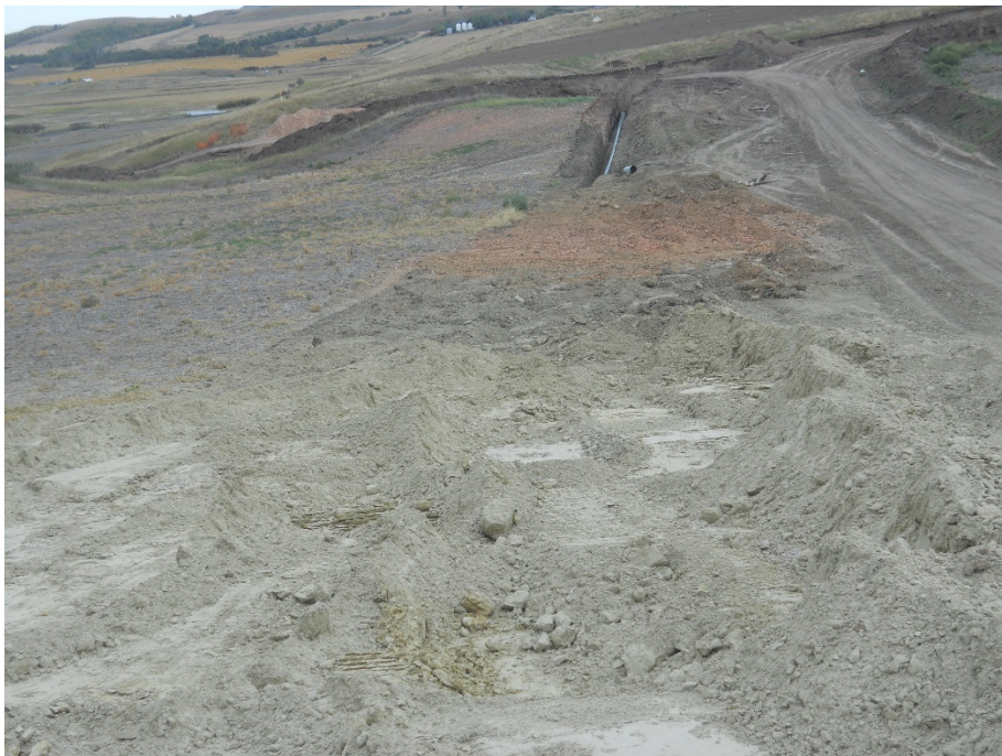
Photo 12: Located at station 38+00, looking west. Piping installed in trench with partial backfill complete. Regrading and leveling not completed.
