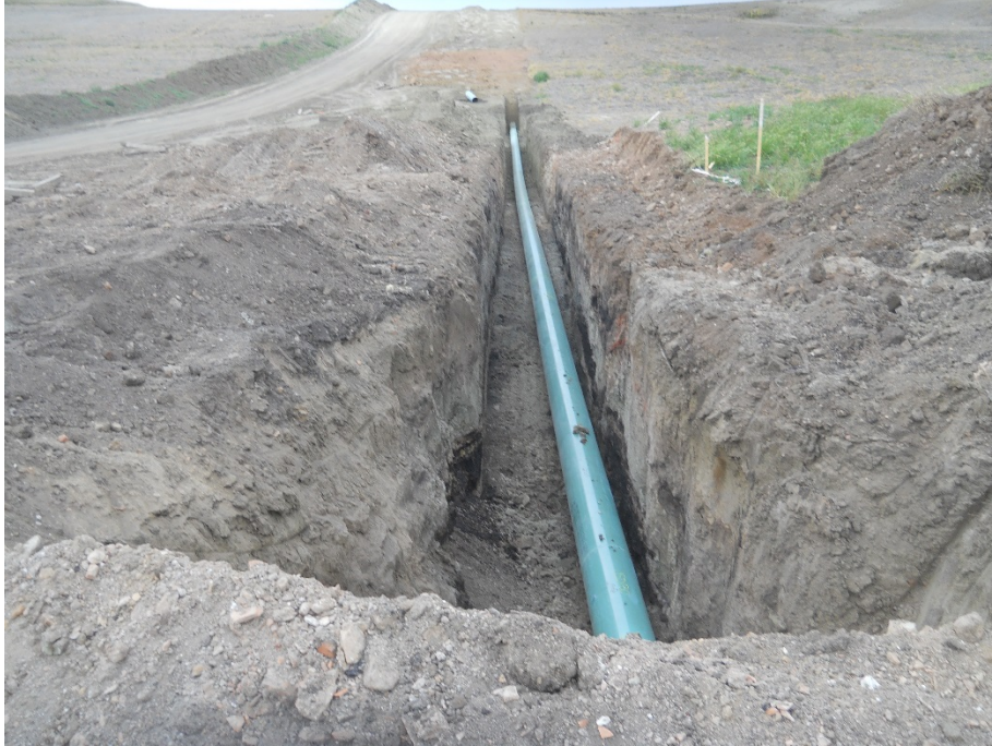
Photo 15: Located at station 51+00, looking west. Photo showing partial open trench with installed pipe ready to be backfilled. Topsoil shown placed on edge of Right of Way, in upper left corner of photo.
