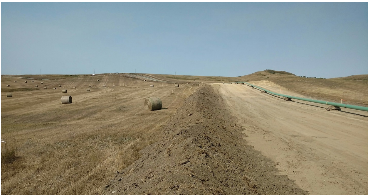
Photo 12: Located at station 57+00, looking west with Right of Way turning southwest. Photo showing graded and stripped Right of Way, topsoil located on left side Right of Way edge. Subsoil pile is located on right side of topsoil, but is segregated and separated. Pipeline is welded and setting on wood skids ready for trenching.
