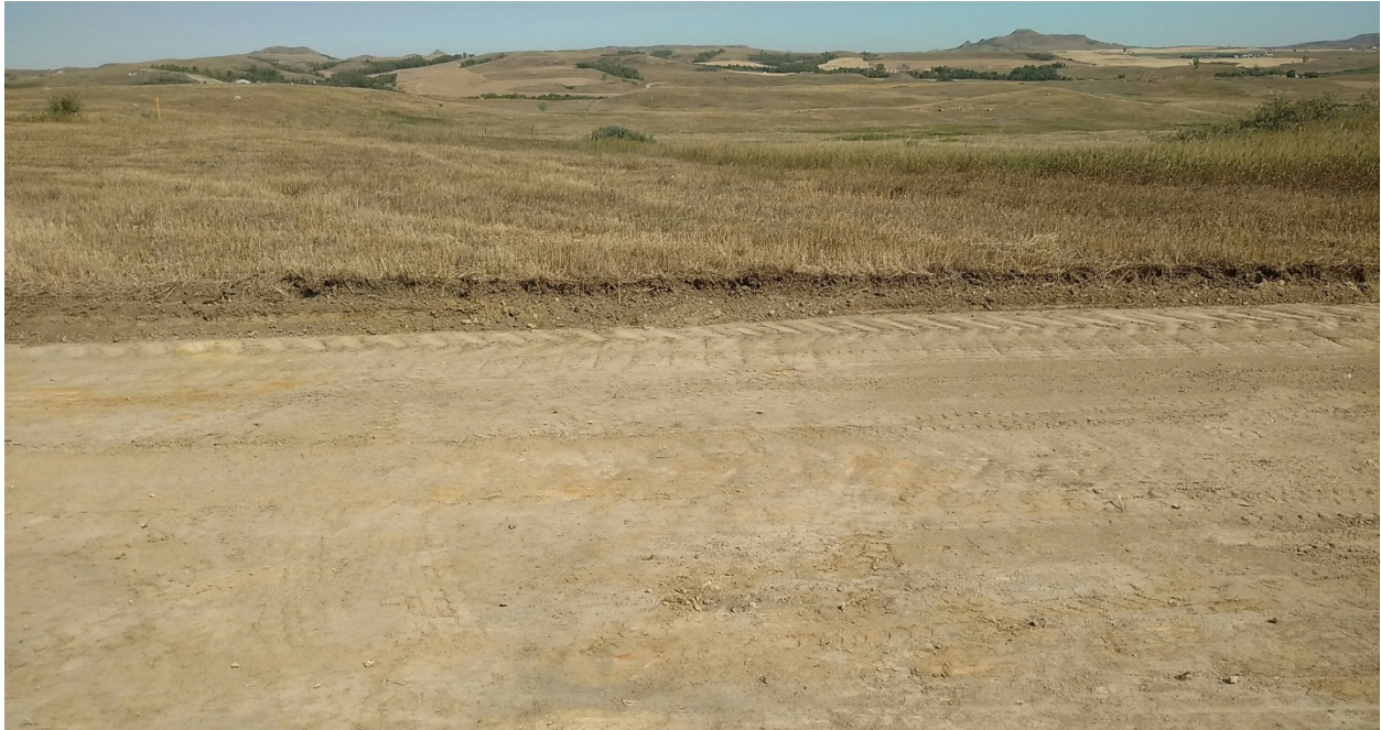
Photo 15: Located at station 75+00, showing stripped Right of Way at approximate topsoil depth of 12 inches. Soil depth is located on south side edge of Right of Way.
