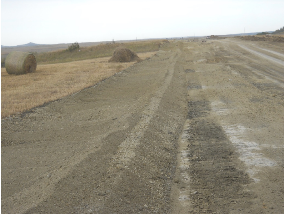
Photo 17: Located at station 57+00, looking west. Photo showing graded Right of Way, with topsoil pushed off on left side of Right of Way edge.
