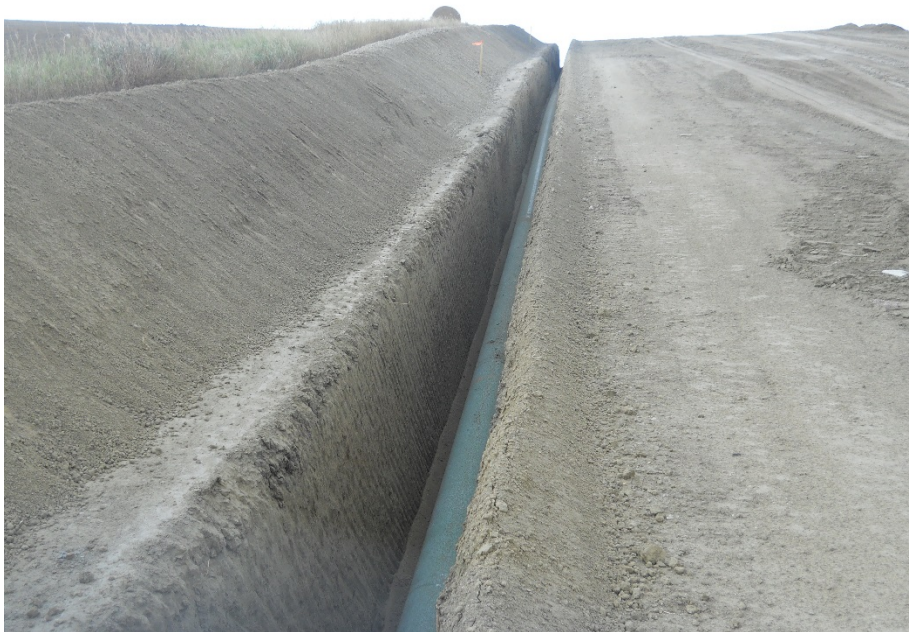
Photo 26: Located at station 105+00, looking south. Photo showing graded Right of Way with dug trench, showing pipeline installed in trench. Trench ready for backfilling as required.
