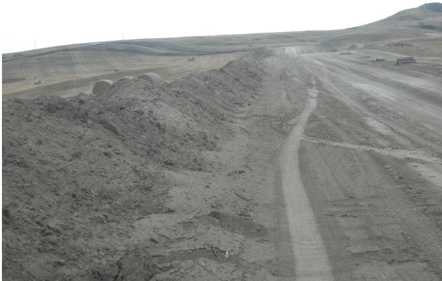
Photo 18: Located at station 63+00, looking west. Photo showing graded Right of Way with wood skids, ready to string out piping. Topsoil pile placed on left side edge on Right of Way.
