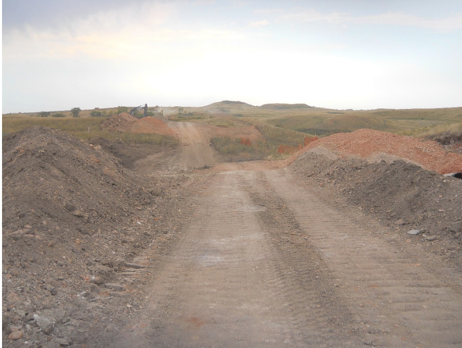
Photo 7: Located at station 27+00, looking west. Right of Way graded with topsoil placed on left side of Right of Way and subsoil on right side. Regrading and leveling are not complete.
