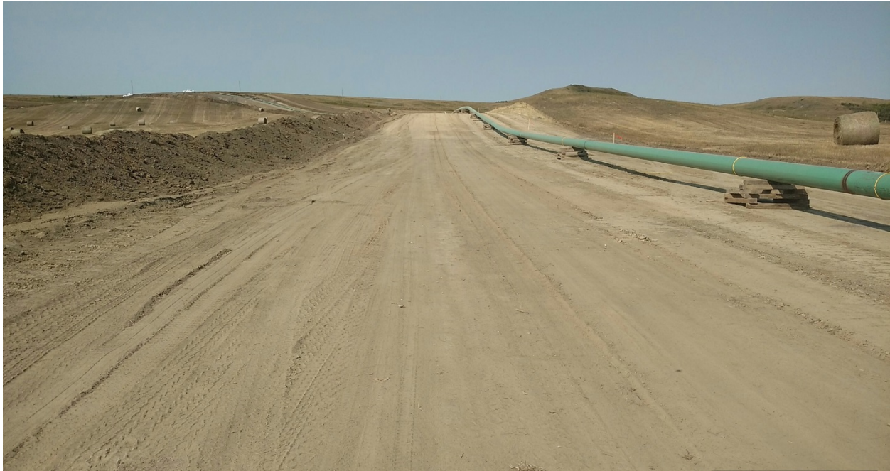
Photo 13: Located at station 63+00, looking west with Right of Way turning southwest. Photo showing graded and stripped Right of Way. Topsoil located on left side edge of Right of Way. Pipeline welded and setting on wood skids ready for trenching.
