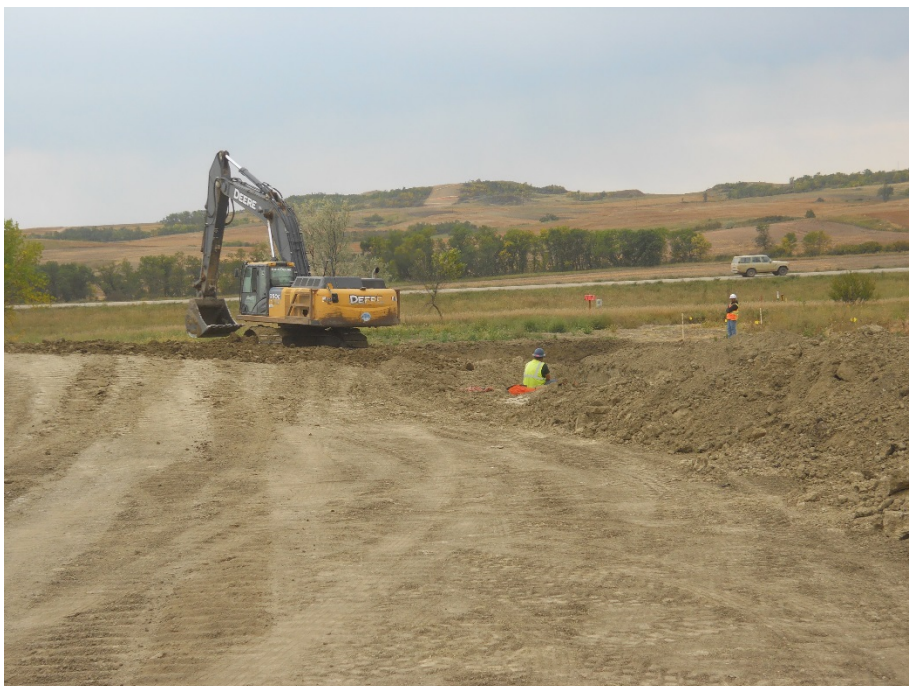
Photo 2: Located at station 6+00, looking south, workers on site backfilling trench and leveling topsoil placement.
