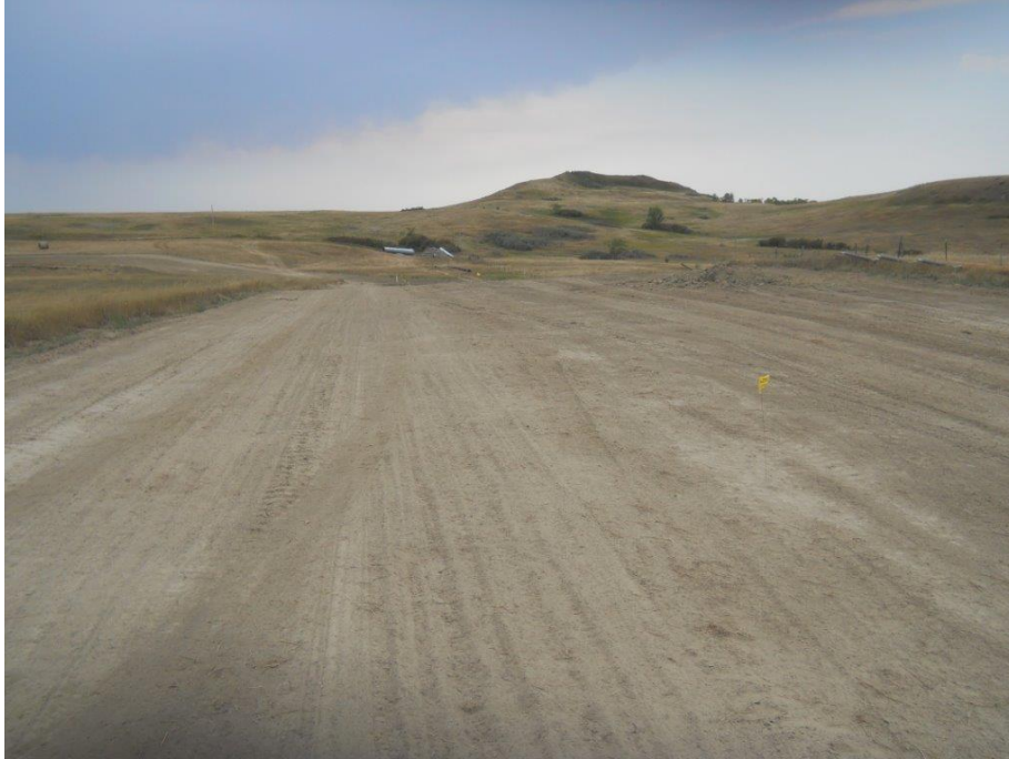
Photo 23: Located at station 84+00, looking west at graded Right of Way. Pipe installed in trench and backfilled. Right of Way topsoil needs to be finished level and cleaned up to original condition.
