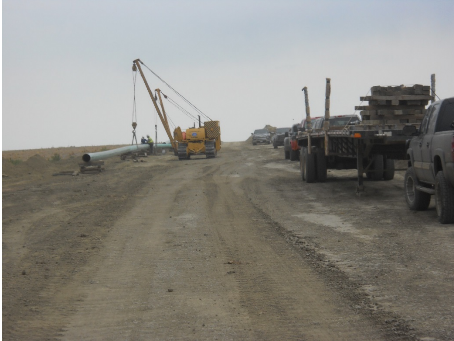
Photo 3: Located at station 12+00, looking north. Workers on site welding pipe. Right of Way graded and ready for trenching.
