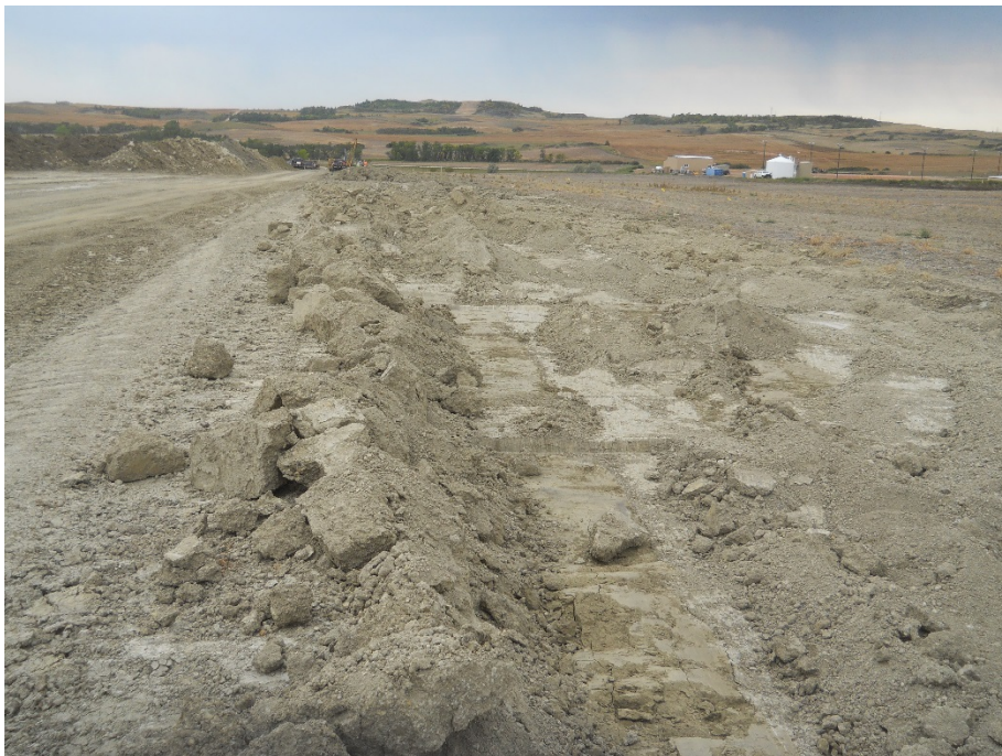
Photo 4: Located at station 15+00, looking south. Photo showing Right of Way backfilled with piping installed. No leveling or grading completed.
