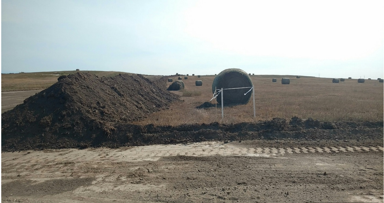
Photo 18: Located at station 81+00, coming from south direction and turning west. Photo showing stripped and graded Right of Way with approximate topsoil depth of 12 inches. Topsoil pile is pushed off on edge along Right of Way, located on north edge of Right of Way easement.
