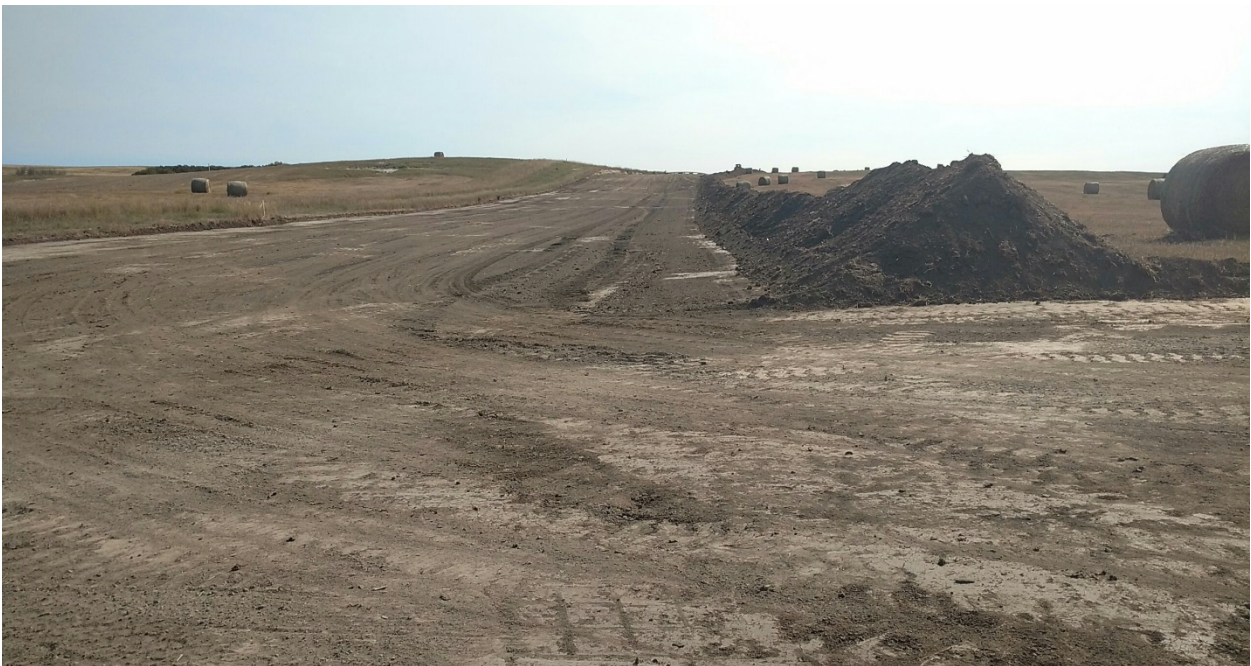
Photo 8: Located at station 27+00, photo showing graded and stripped Right of Way coming from the south, turning and heading west. 12 inch deep topsoil has been pushed off on edge of Right of Way easement.
