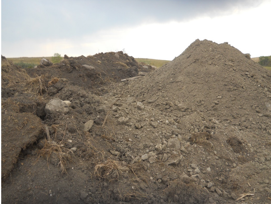
Photo 9: Located at station PI 30+26.19, looking west. Along Right of Way edge, subsoil pile is placed on left side edge of Right of Way. Topsoil pile is placed to the left of the subsoil pile. Both piles appear to be close enough that both soil types are touching.
