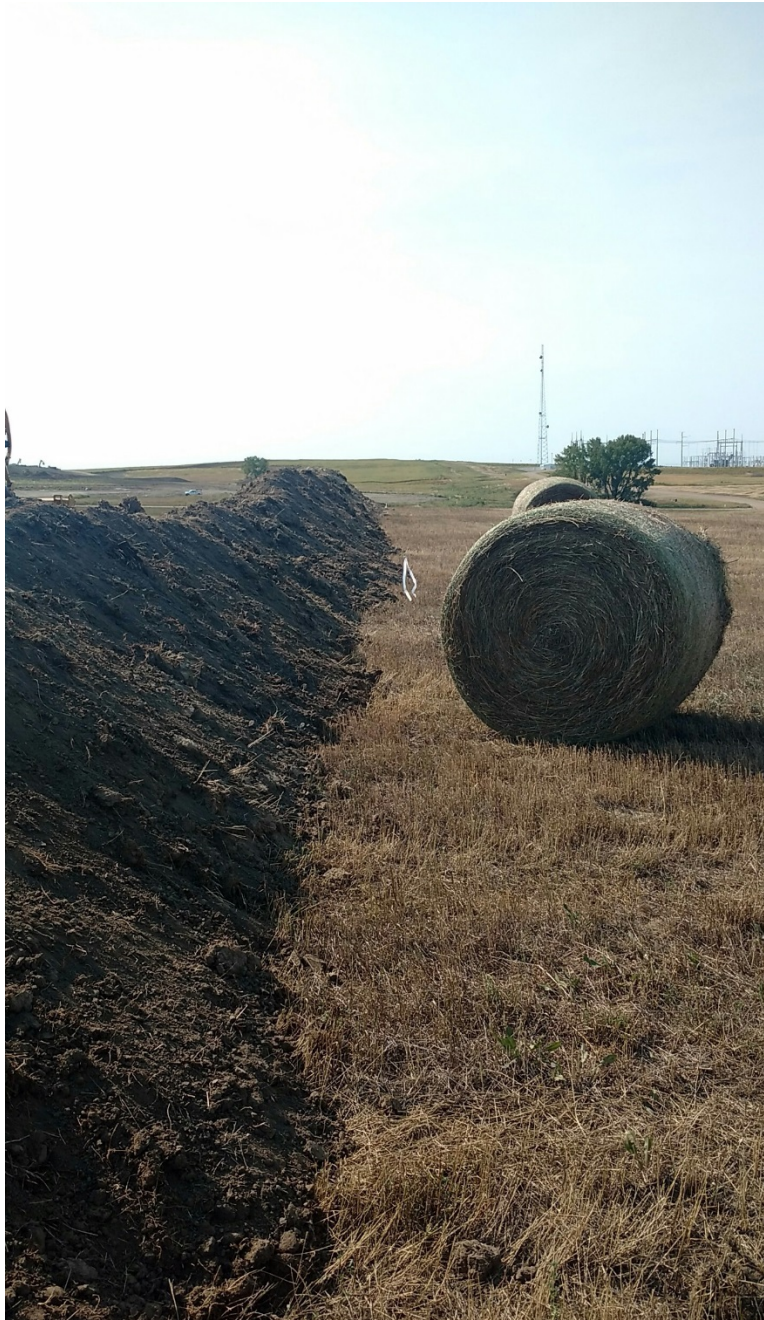
Photo 6: Located at station 18+00, photo showing graded Right of Way looking south, with topsoil pushed off on Right of Way easement edge.
