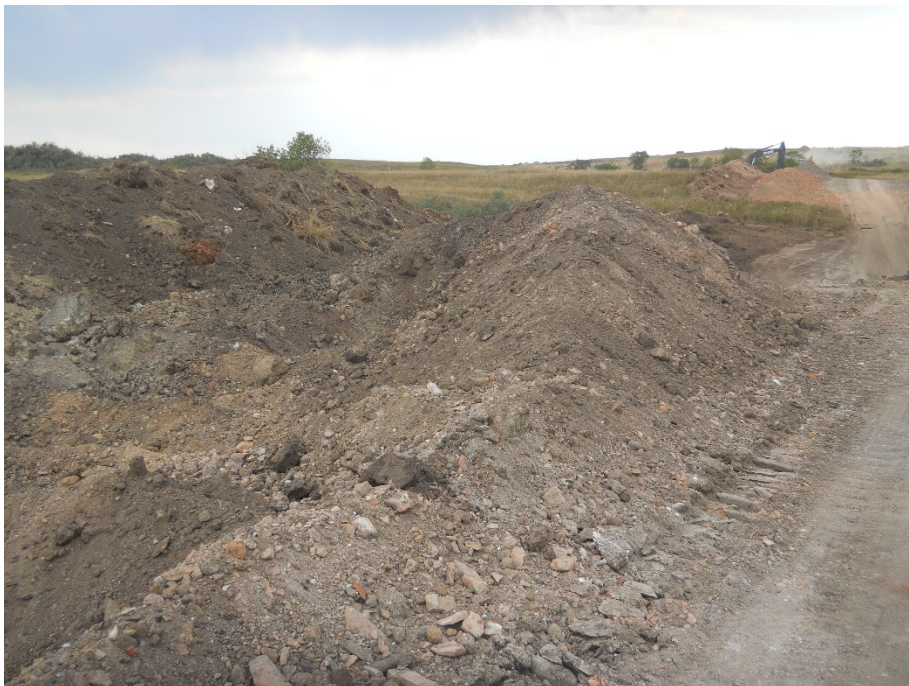
Photo 8: Located at station 29+00, looking west. Along Right of Way edge, subsoil is placed on left side edge of Right of Way. Topsoil pile placed on left side of subsoil pile. Both piles appear to be close enough that both soil types are touching.
