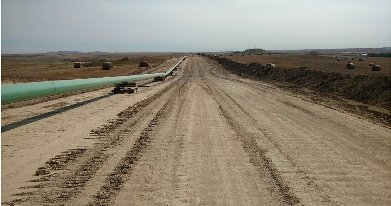
Photo 20: Located at station 87+00, looking west. Right of Way has been graded and stripped. Topsoil pile located on right edge along Right of Way. Pipeline is welded and setting on wood skids ready for trenching.
