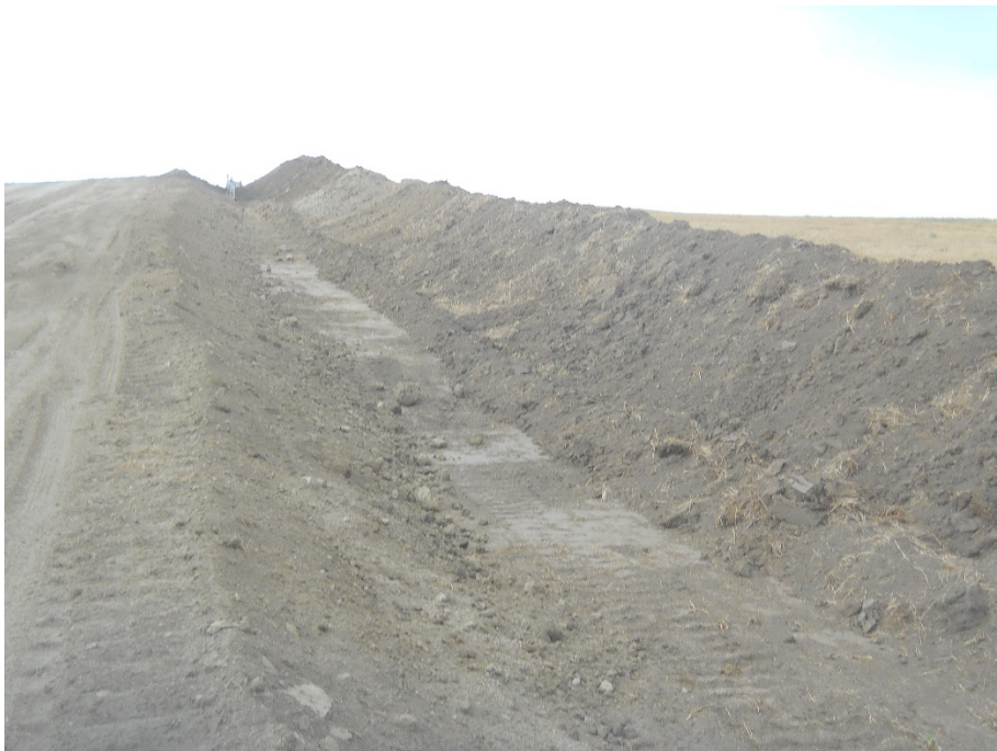
Photo 20: Located at station 75+00, looking south. Photo showing graded Right of Way, showing subsoil pile on left side of photo, on Right of Way edge. Topsoil pile shown on right side of photo, pushed on right edge of Right of Way. BMP silt fence shown on top of photo to keep soil segregated.
