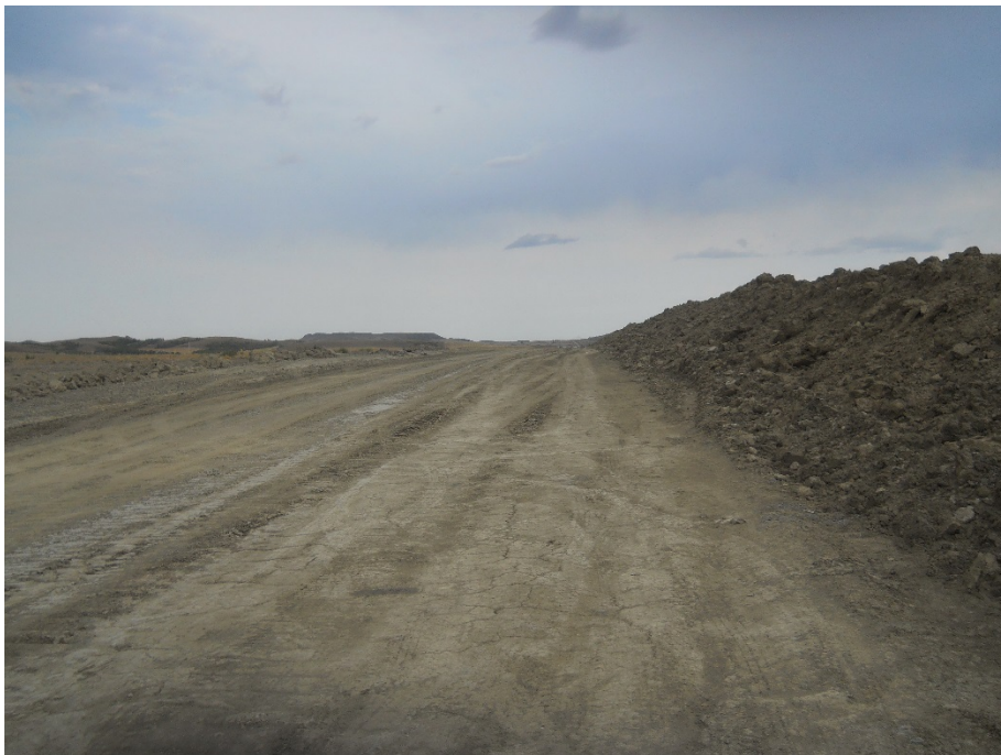
Photo 16: Located at station 54+00, looking west. Photo showing graded Right of Way with topsoil pile pushed off edge and placed on right side of photo. Right of Way nearly ready for trenching and pipe.
