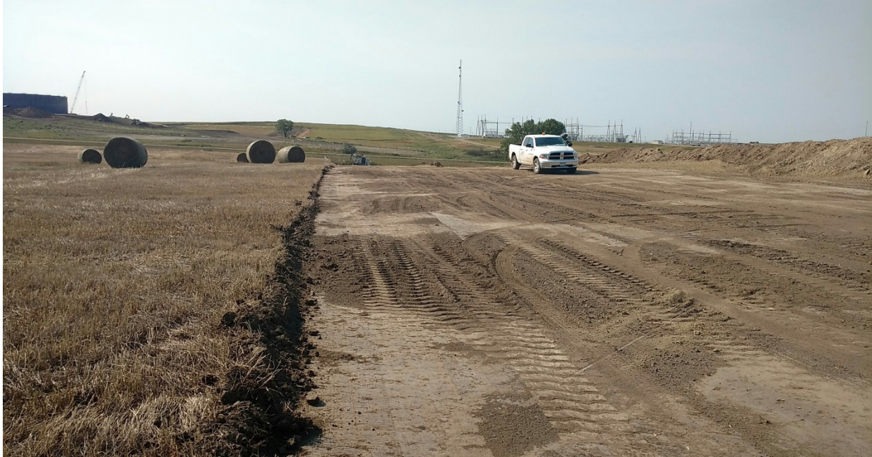
Photo 1: Located at station 0+00, showing Right of Way, beginning point of pipeline at Johnson's Corner. Right of Way has been graded with topsoil pushed off on edge of easement Right of Way. Photo looking northwest and taken on north side of Hwy 73.
