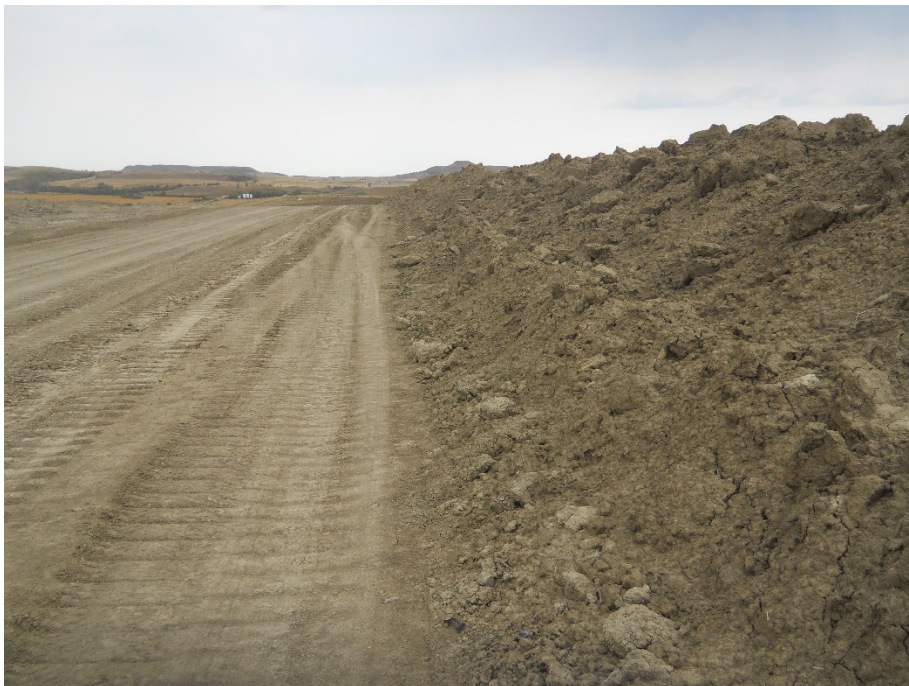
Photo 28: Located at station 111+00, looking south showing graded Right of Way. Piping placed in trench and backfilled. Topsoil pushed off Right of Way and placed on right edge of easement.
