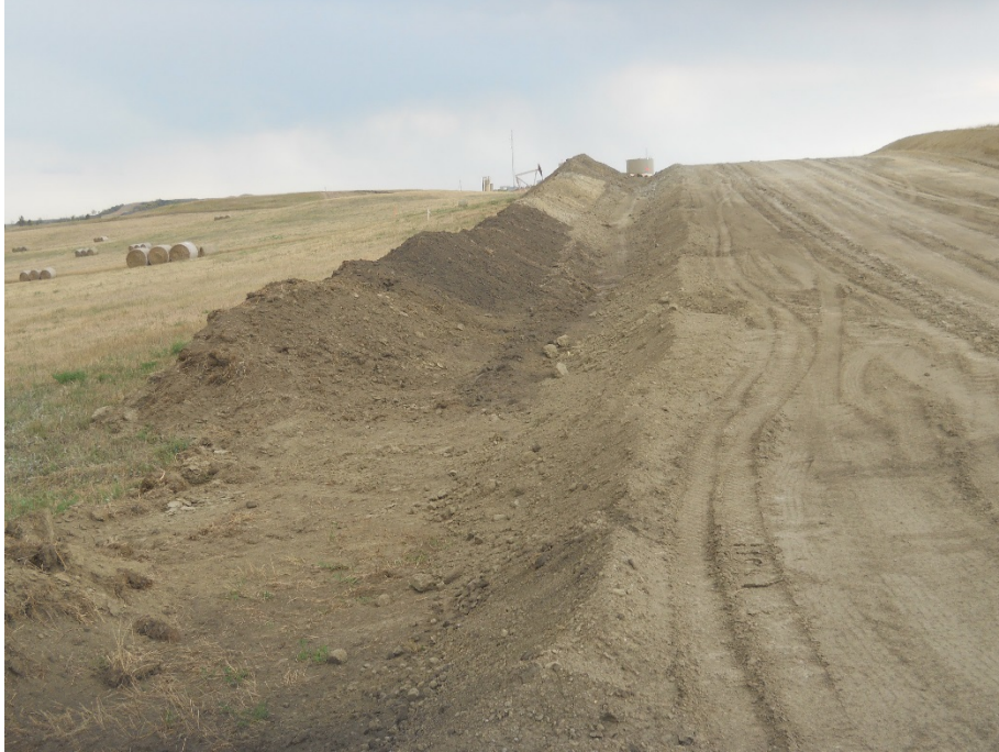
Photo 21: Located at station 78+00, looking south. Photo showing graded Right of Way, with pipe installed in trench and backfilled. Right of Way has two toning slope with subsoil shown on left side of Right of Way and topsoil pile to left of subsoil. Soil types do not appear to be touching or connected.
