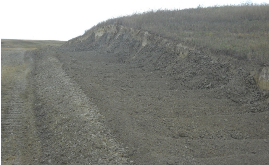
Photo 24: Located at station 87+00, looking north. Photo showing Right of Way with two toning slope with topsoil pile shown on left side of photo.
