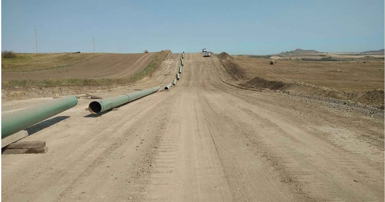
Photo 9: Located at station 39+00, Photo looking east, showing graded and stripped Right of Way. Topsoil pushed off right side edge on Right of Way. Pipe has been strung out, setting of wood skids ready for welding.
