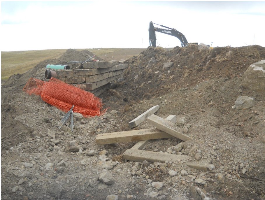
Photo 10: Located at station PI 37+41.66, looking west. Photo showing topsoil and subsoil piles touching and piled together. Wood skids and other pipeline materials shown in photo. No clean up done.
