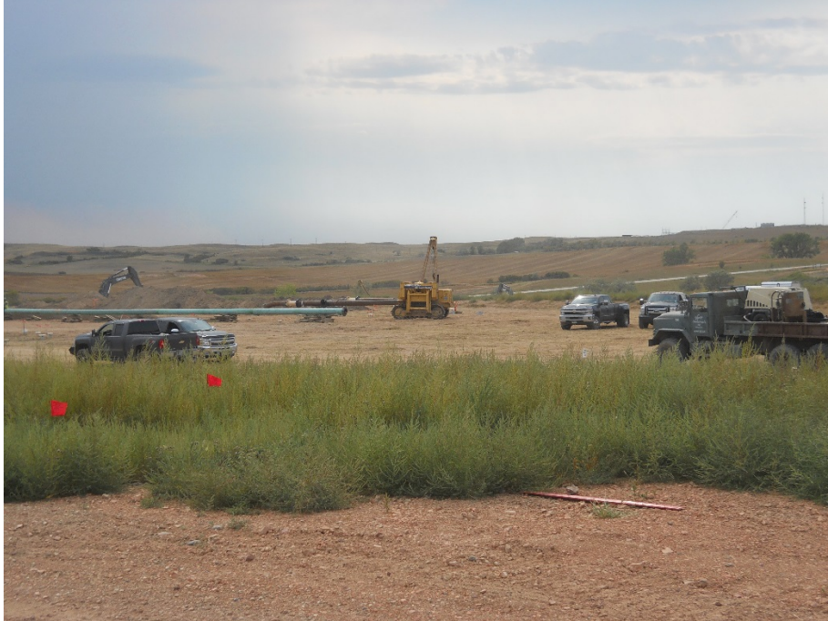
Photo 1: Located at station 0+00, beginning of pipeline at Johnsons Corner surface site. Photo looking west with valve launcher/receiver beyond.
