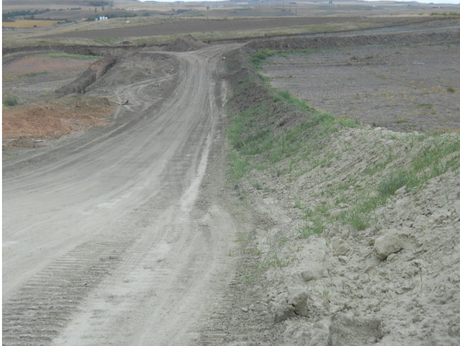
Photo 11: Located at station 36+00, looking west. Photo showing graded Right of Way with open trench having pipe installed in trench. Trench not completely backfilled. Topsoil pile shown on right side of Right of Way.
