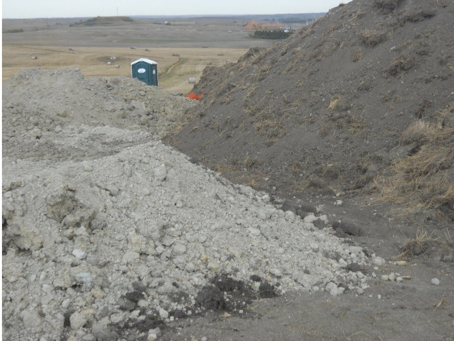
Photo 27: Located at station 108+00, looking south on Right of Way. Photo showing topsoil pile located on right side of photo and subsoil pile on left side of photo. Soil types appear to be touching.
