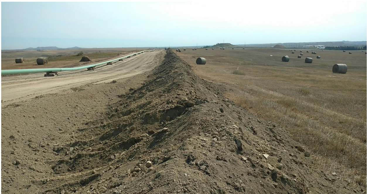
Photo 16: Located at station 76+00, looking south. Photo showing graded and stripped Right of Way. Topsoil pile is located far right on Right of Way edge. Subsoil pile is located on left side of topsoil location. Both soil types are segregated and separated. Pipeline is welded and setting on skids ready for trenching.
