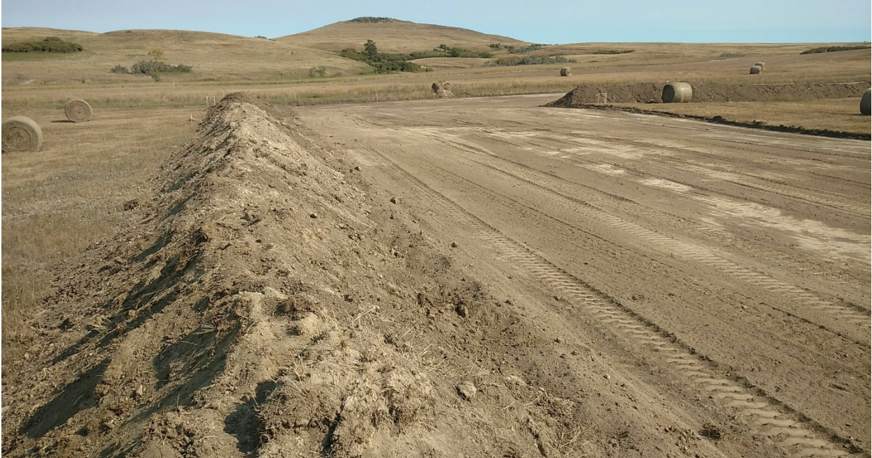
Photo 7: Located at station PI 25+09.66, showing Right of Way direction looking east then heading south. Photo showing stripped topsoil pushed to edge of Right of Way and 12 inch deep cut of Right of Way on right side of photo.
