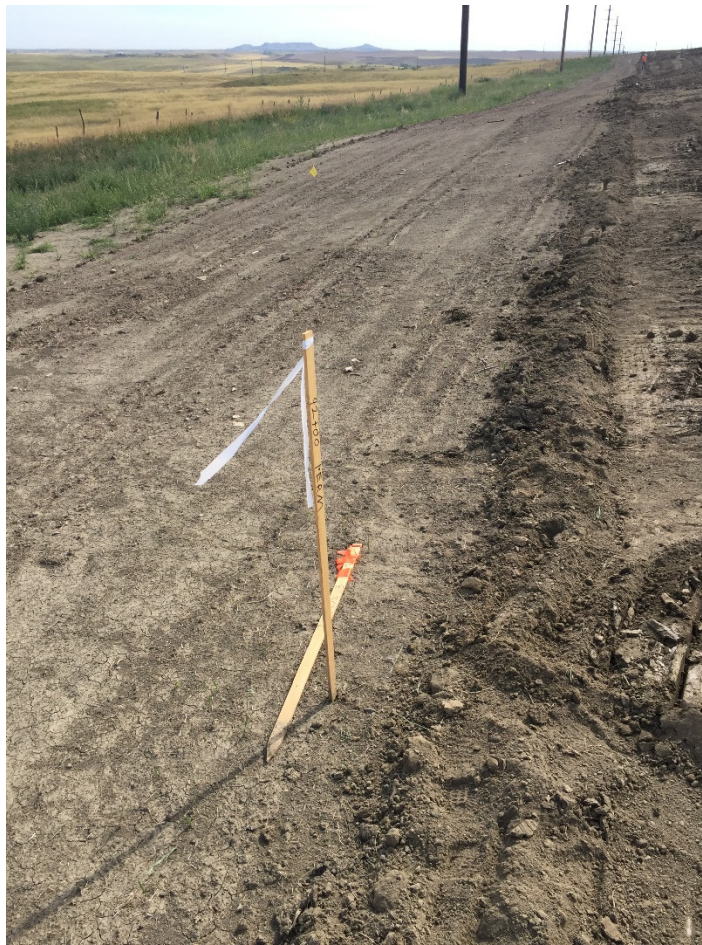
Photo 14: Sta. 92+00 showing back side of topsoil pile along R/W. The previous pipe installation is visible to the north or left with no vegetation.
