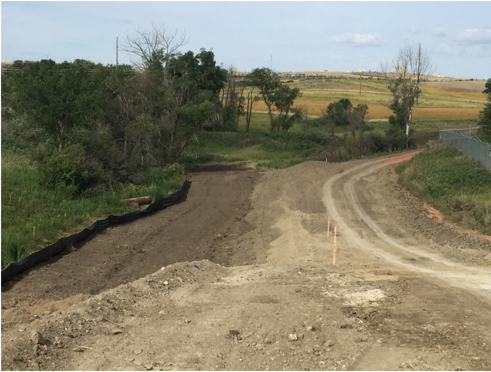
Photo 10: Sta. 7+00 looking west at the channel with topsoil removed to safe location and silt fence installed as previously committed to on site.
