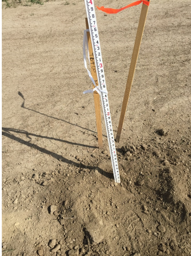
Photo 18: Sta. 92+00 showing 4-5 inches topsoil removal. Notice soil is same from previous pipe installation on the left outside of R/W.
