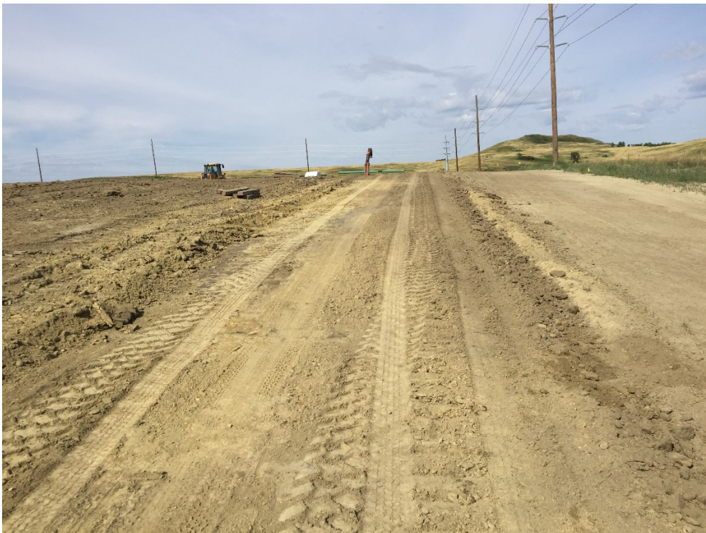
Photo 19: Facing west, Sta. 100+00. Area to right is previously installed pipeline. Area on the left side is the current project.
