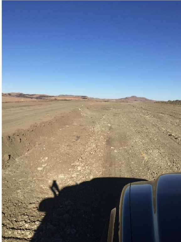
Picture 18: Grading in progress, looking north. Beginning to spread topsoil from berm
