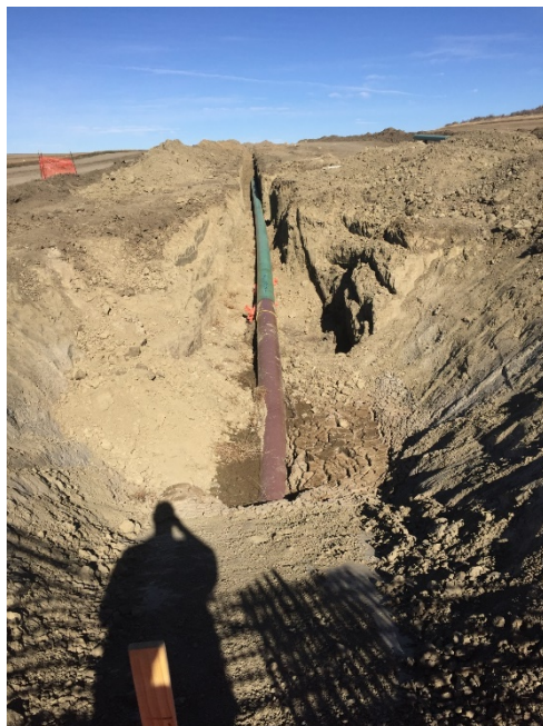
Picture 2: Pipe bore/trench. Depths checked at 4 feet or greater cover in trench.
