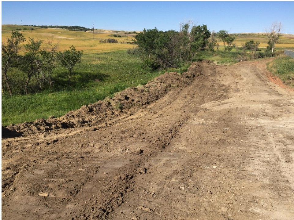
Photo 6: Sta. 5+50 looking west showing top soil pile along drainage area. See photo 10 on August 8 showing replacement of topsoil stockpile with silt fence.
