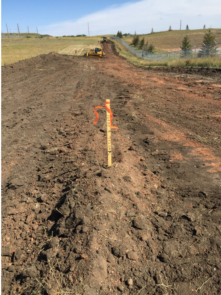
Photo 9: Sta. 12+00 looking north showing an old road under the stripping of limited top soil
