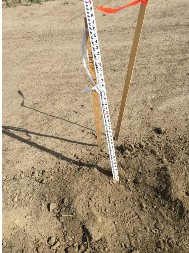
Photo 18: Sta. 92+00 showing 4-5 inches topsoil removal. Notice soil is same from previous pipe installation on the left outside of R/W.
