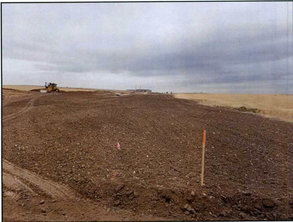
Figure 4. A portion of the pipeline runs parallel with the Dakota Access Pipeline (reclaimed area).
