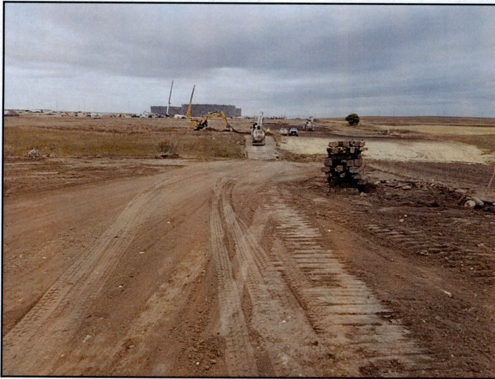
Figure 6. Photo showing the end of topsoil stripping on the north/east end of corridor.
