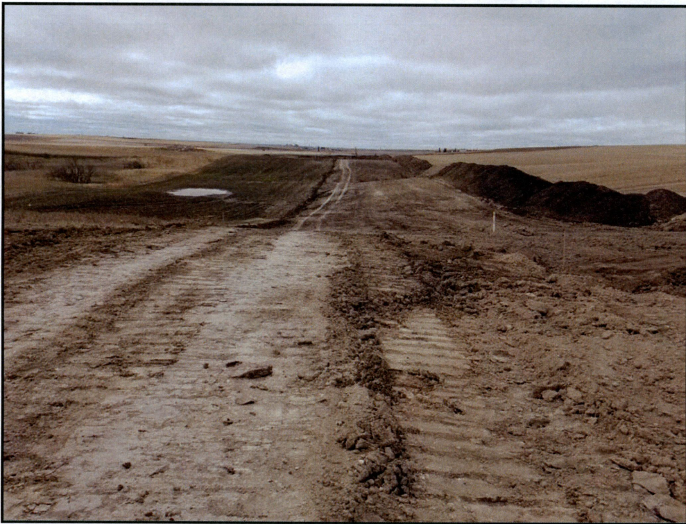
Figure 7. Photo taken looking west down the pipeline corridor. Pipeline has been installed and backfilled. Topsoil has not been re-spread.
