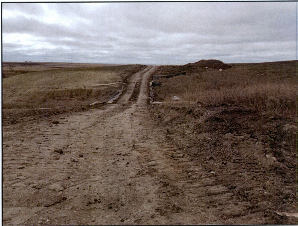
Figure 8. Photo taken looking west across matting installed in upland drain. Silt fence and straw waddles are properly installed and functioning.
