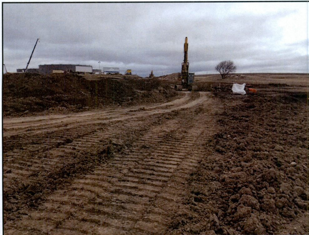
Figure 9. Photo taken, facing east, of construction corridor at dogleg near ETP facility.
