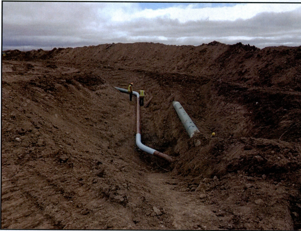
Figure 10. Photo of ETP Pipeline crossing under Dakota Access Pipeline. Pipeline construction is currently underway from this point to the ETP Facility.
