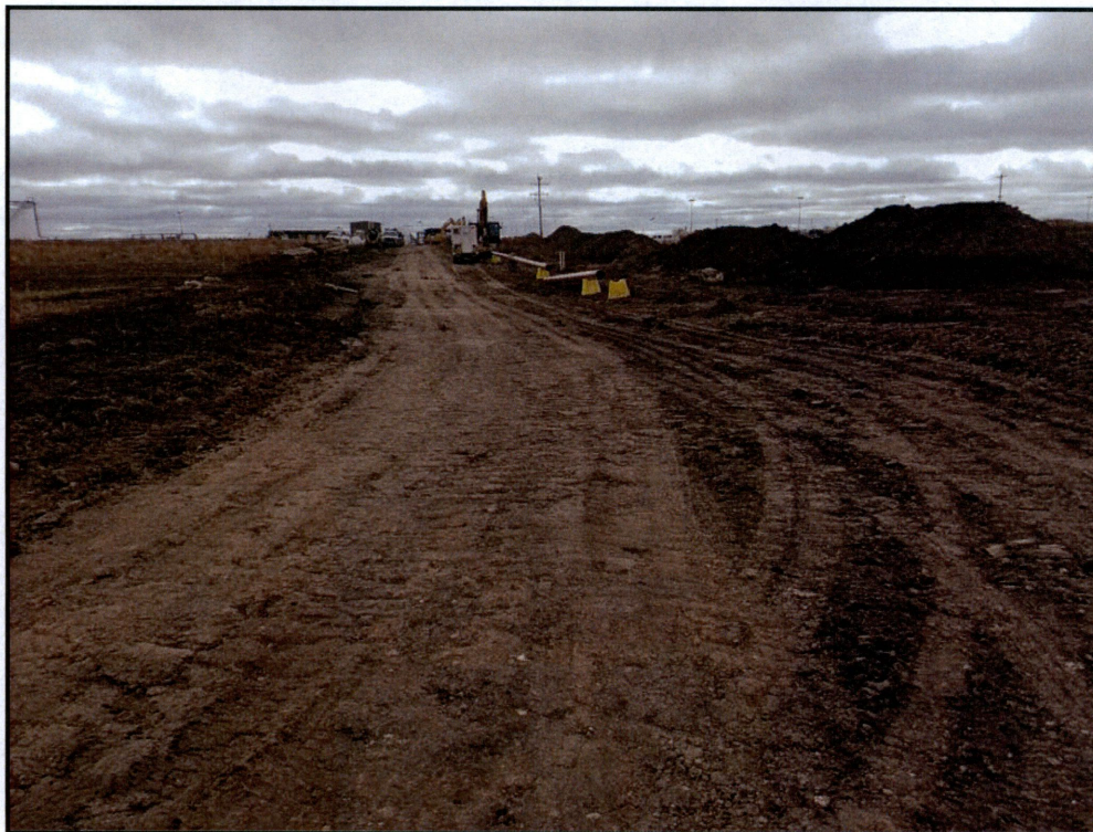
Figure 3. Photo taken looking north. Pipeline has been installed and trench filled. Pipe strung in photo is for the RFT tie-in.
