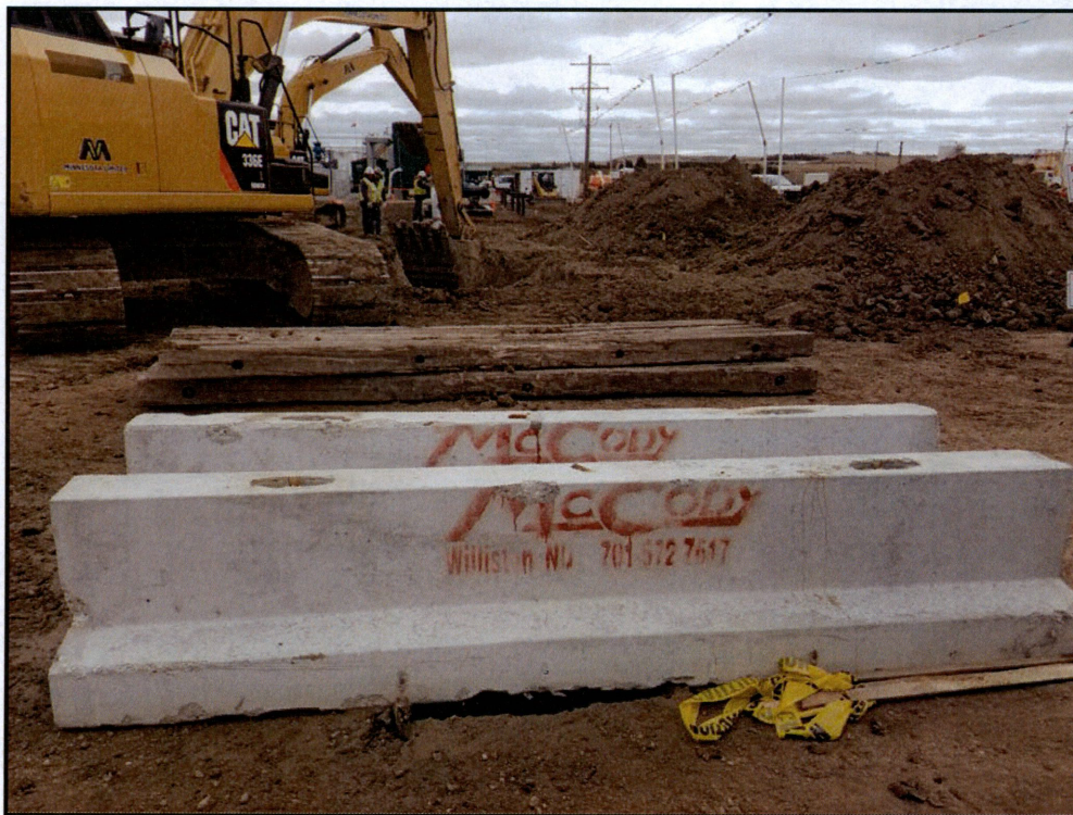
Figure 2. Photo taken facing south from the RFT access road. Construction of ditch to the RFT facility was underway.
