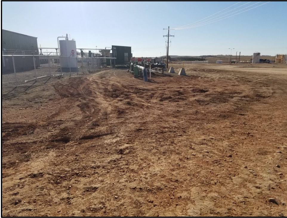
Figure 2. Pipeline valve connection at the Ramberg Truck Facility.
