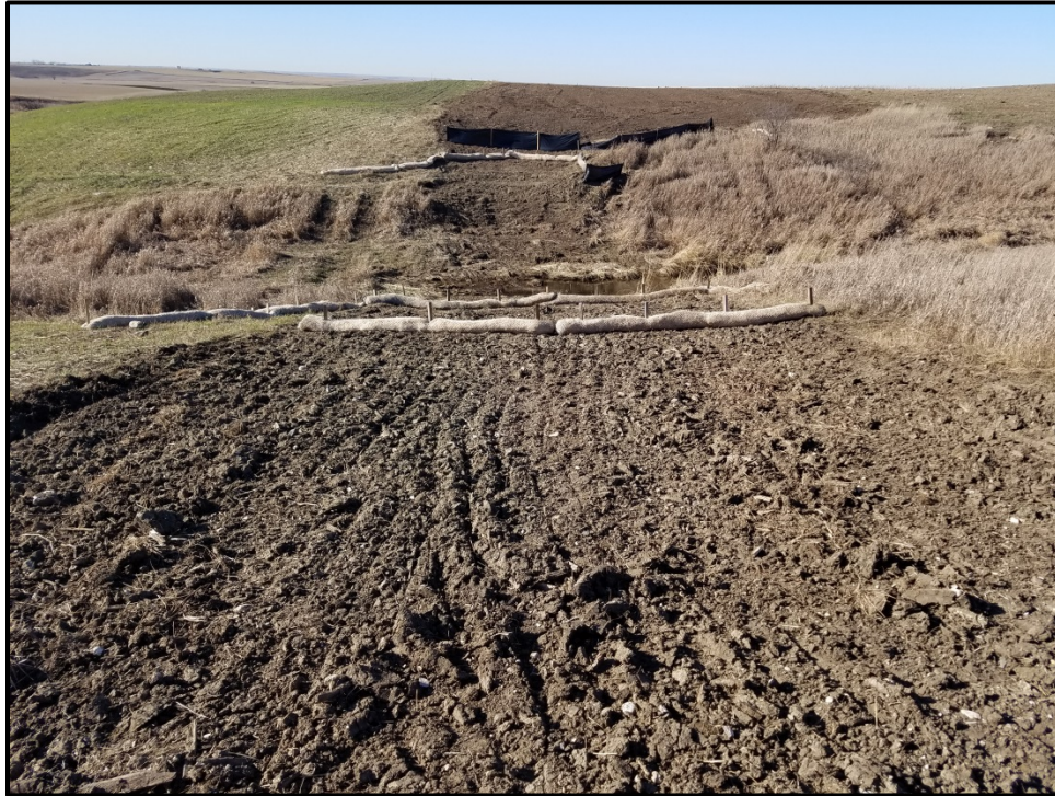
Figure 4. Silt fence and straw waddles were installed in appropriate areas. The ROW width was reduced at the waterbody crossing to minimum disturbance.
