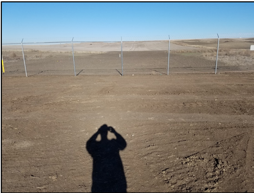
Figure 3. Photo looking north from Ramberg Truck Facility. Pipeline is 100% installed, fencing in place, land has been re-contoured, and disced.
