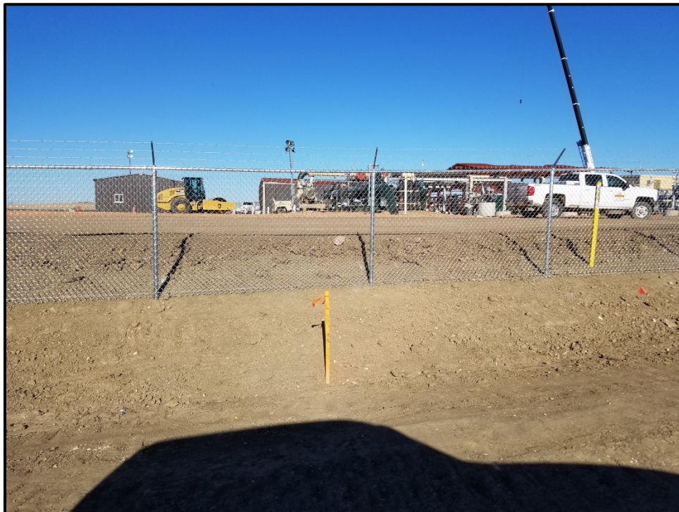
Figure 5. Photo of valve connection to the ETP Facility.
