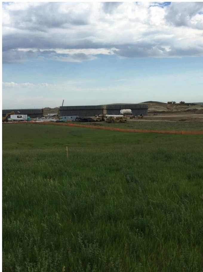
Proposed tie-in point at DAPL Watford City Terminal (under construction at time of photo, July 8 th , 2016)
