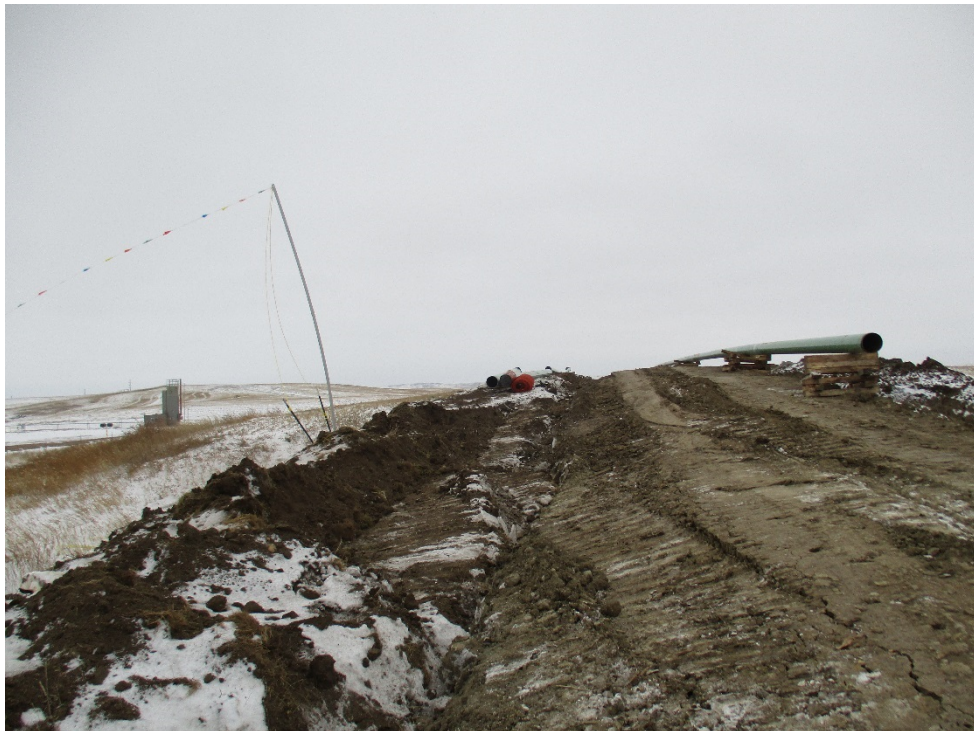
Below: Photo 10 (pt. 1) – Topsoil and subsoil piles in contact with each other. Near road bore. Same area as photo #9. Direction: South.
