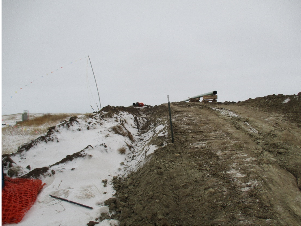
Above: Photo 9 (pt. 1) – Topsoil pile to the far left. Topsoil and subsoil piles touching/too close to each other. Possible subsoil on top of topsoil. Trench to the far right of photo. Near road bore. Area was two-toned/side-sloped. Direction: South.
