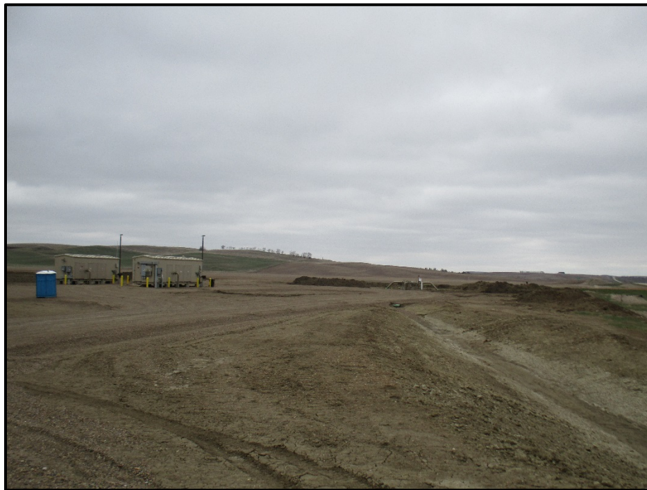
Photo 18. (GPS Point #518) – View of North Load-In Facility. Area will be fenced and gated. Direction: West.
