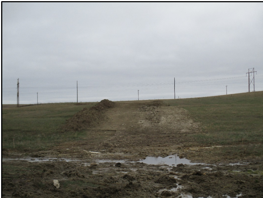
Photo 6. (GPS Point #510) – This is a wetland area that was double ditched (same area as photo #6). Caliber stated at this wetland location they will be installing wattles, Curlex erosion control blanket, and silt fences as needed and will make additions as needed. Direction: East.
