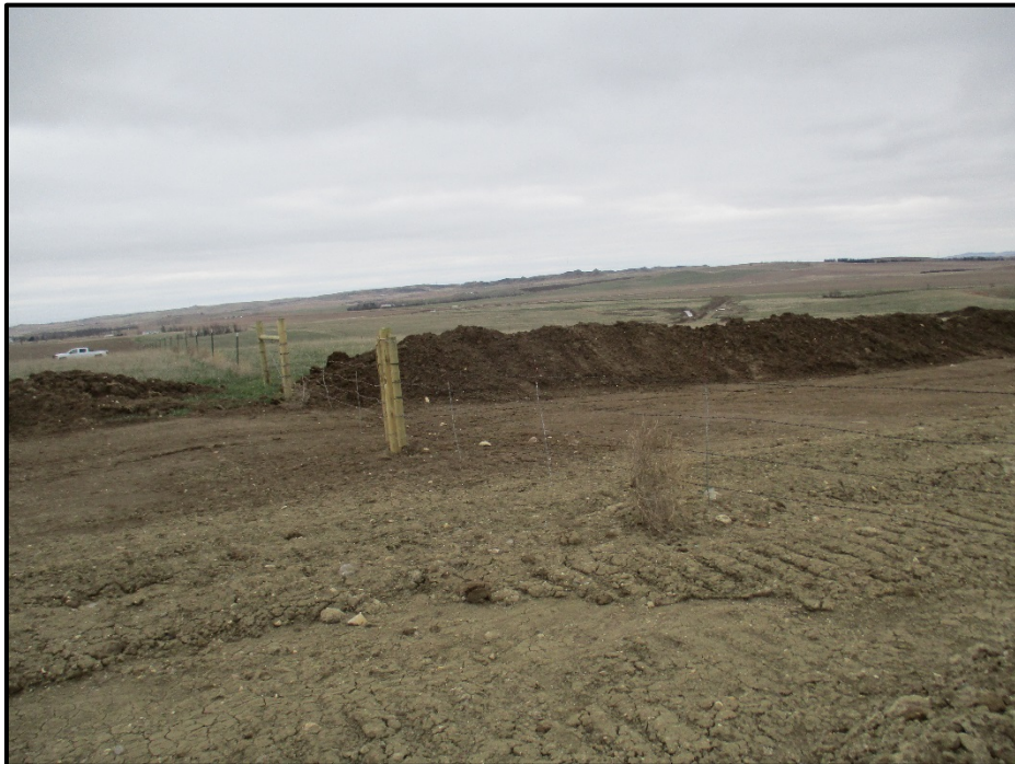
Photo 12. (GPS Point #514) – Gate and fence installed by Caliber, it currently has two gates on it but will be re-done to only have one gate when construction is finished. Direction: South.
