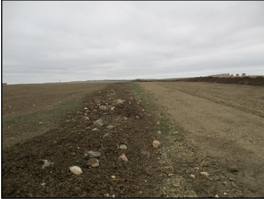
Photo 9. (GPS Point #514) – Area shows rocks that have been picked from the ROW they will be piled up, per landowner request. Topsoil (to the right of photo) has not been replaced along the ROW. Dakota Access Pipeline (DAPL) ROW is to the left of photo. Direction: East.
