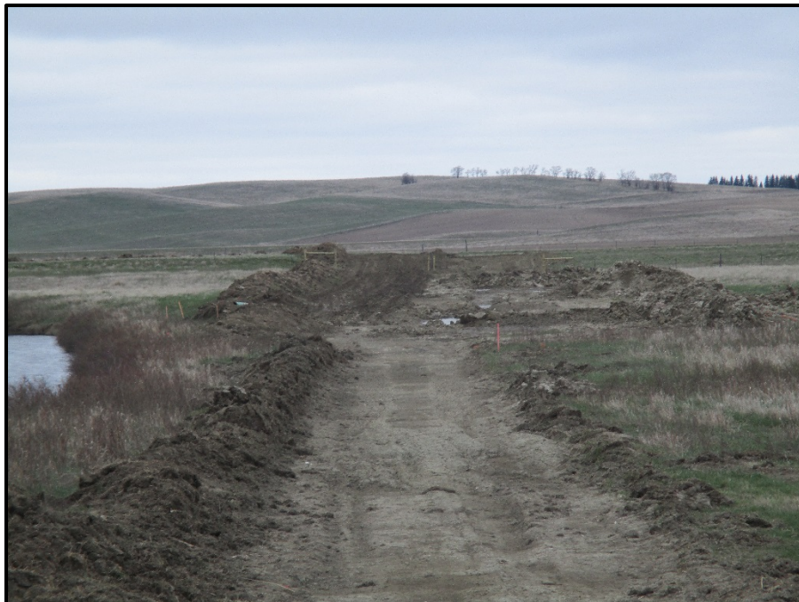
Photo 16. (GPS Point #517) – Bore location for stream crossing (on south side of stream). Area in the lower portion of the photo was used as a travel lane, topsoil was removed for temporary road. The area in upper portion of the photo is the bore location with the extended ROW (for the bore). Direction: Southwest.
