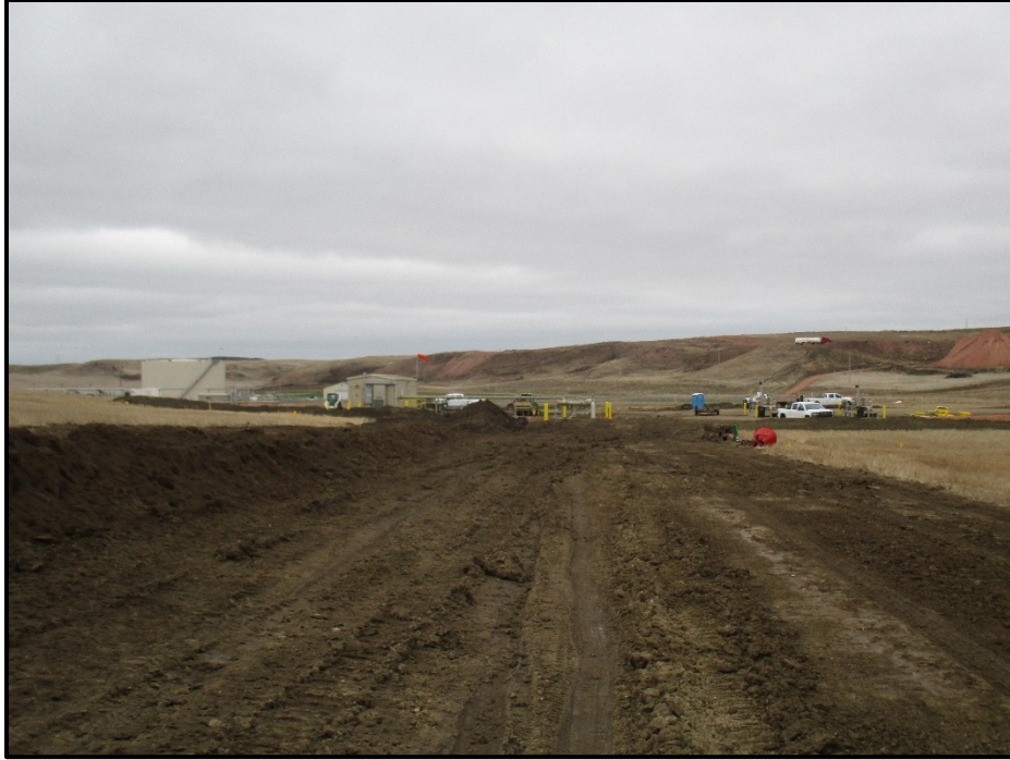
Photo 1. (GPS Point #508) – This area along the ROW had a small amount of soil subsidence, it was bladed and re-contoured. Topsoil pile to the left of the photo. The ROW connects to the South Loadout Facility. Direction: South.
