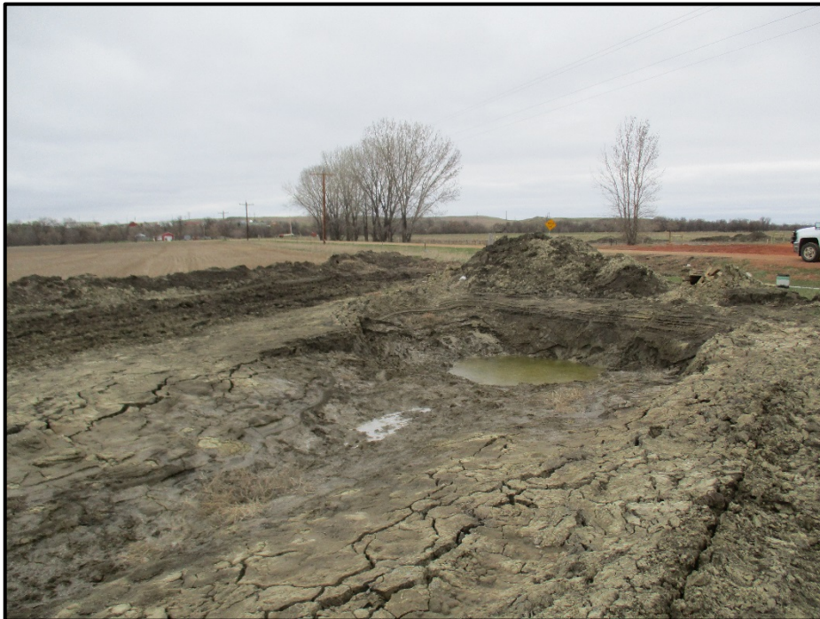
Photo 8. (GPS Point #512) – Sunken bell hole and trench, due to extensive snow in the area and the backfill material. This will be rectified during reclamation work. Direction: South.
