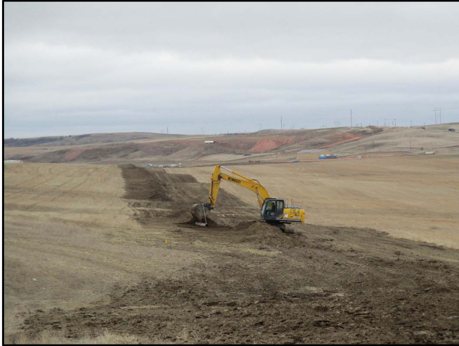
Photo 3. (GPS Point #509) – Equipment shown pulling back topsoil, notice the claws on the bucket are not being used. Topsoil is pulled to center of ROW so dozer can easily spread it over the ROW. Direction: South.
