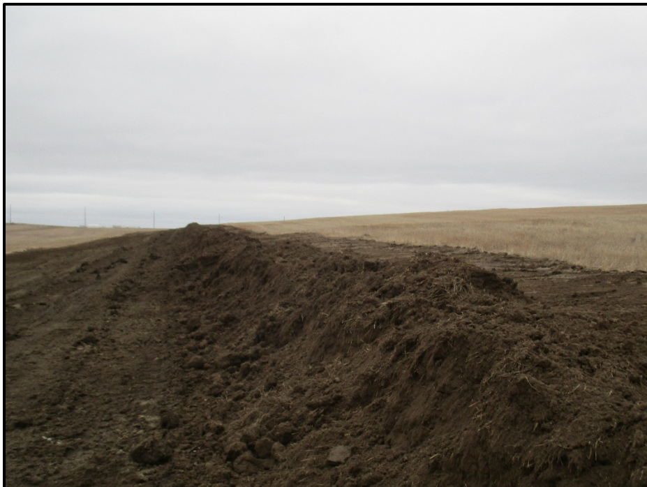
Photo 2. (GPS Point #508) – Topsoil pile has been pushed into the center of the ROW and is no longer along the edge. This gives the dozer access to spread out the topsoil pile. Direction: North.
