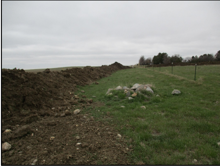
Photo 11. (GPS Point #515) – Topsoil pile along edge of ROW, with untouched rock pile on adjacent land, one of a few in the area. Direction: North.
