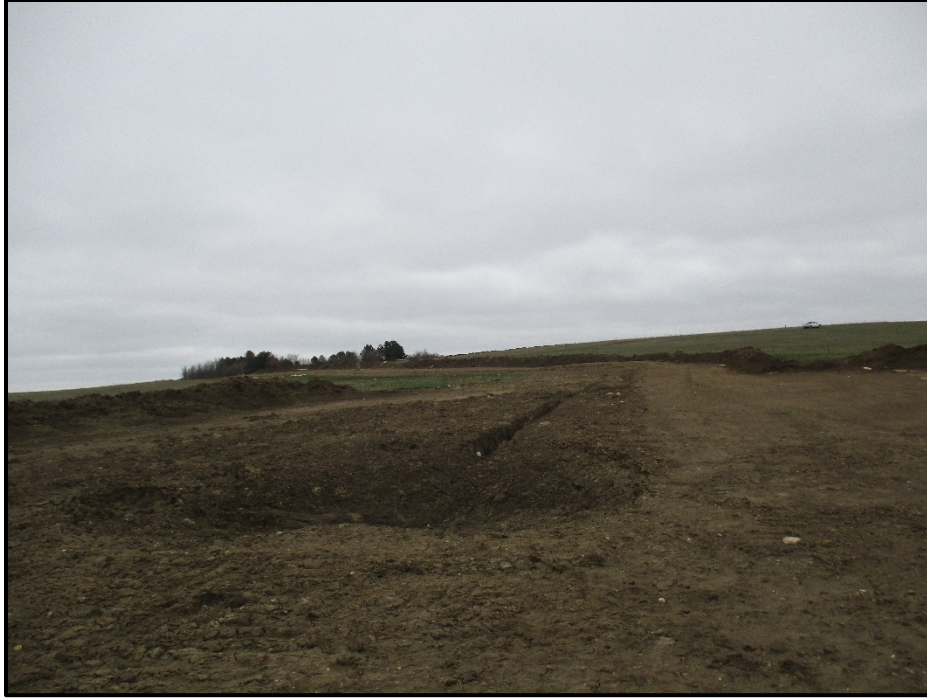
Photo 17. (GPS Point #516) – Bore location for stream crossing (on north side of stream). There is soil subsidence along the trench and bell hole area. Area will be re-contoured and likely ripped before topsoil is replaced. Direction: Northwest.
