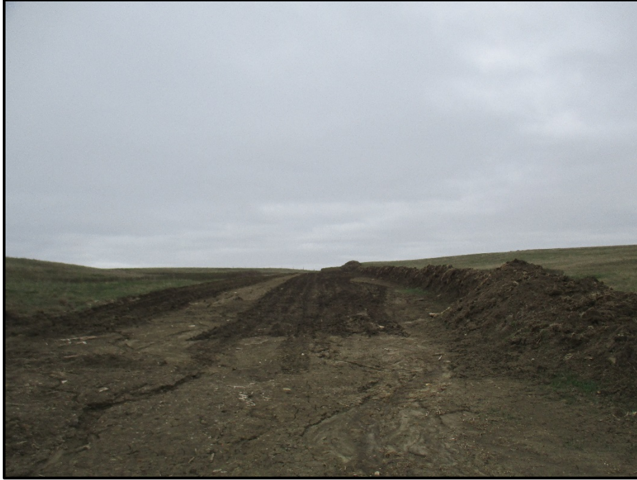
Photo 7. (GPS Point #510) – This area along the ROW has been ripped with the exception of the centerline where the trench was. Direction: West.
