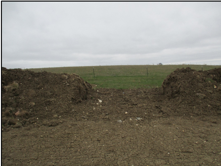
Photo 14. (GPS Point #515) – Open space along piled topsoil. Space was left open for drainage.
