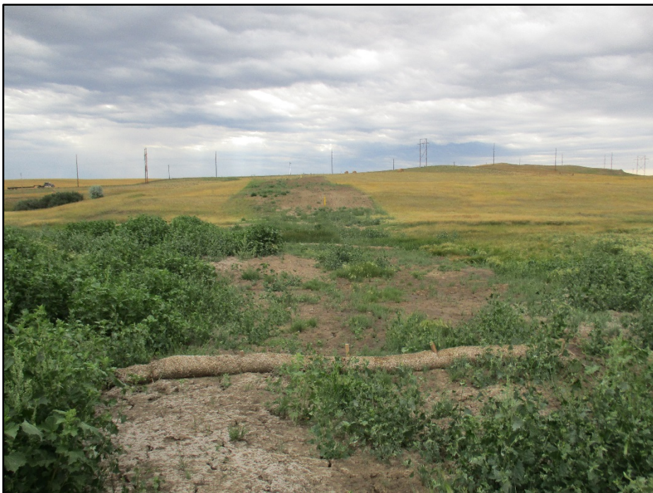
Photo 14. (GPS Point near #529) – View near wetland area. Straw wattles were observed. Area is poorly vegetated, with weeds and some native plants along the lower portion of the wetland. Poor vegetation most likely due to drought conditions. Direction: East.
