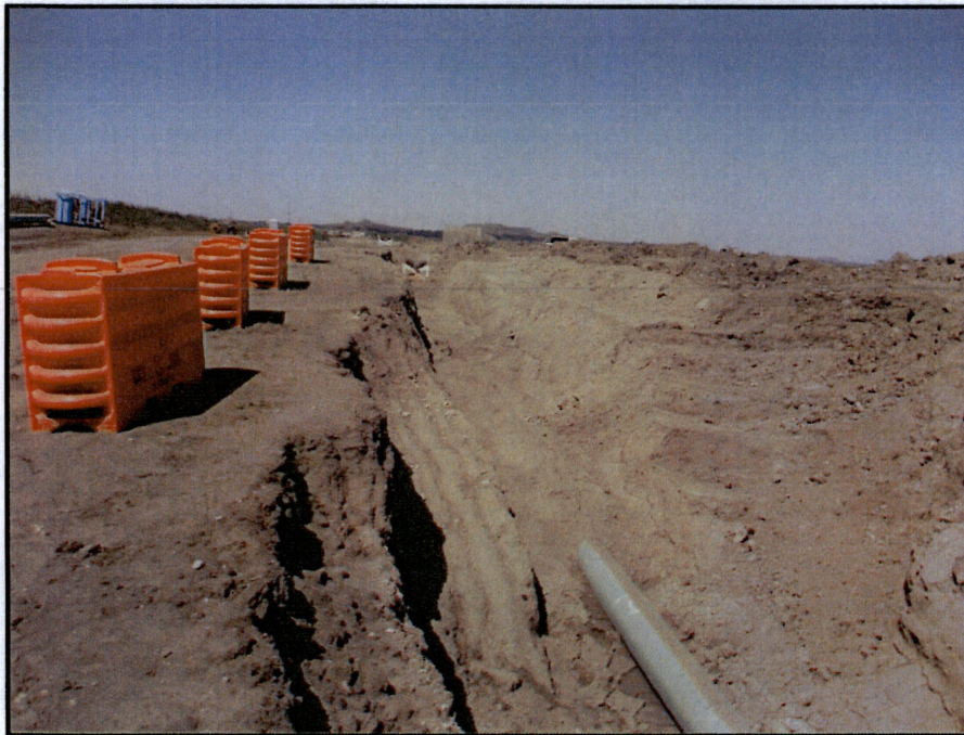
Photo 10. (GPS Point #450) - Open trench with partially covered pipe in trench. Orange safety blockades to the left of photo. White and black pipe rollers (visible in trench in far distance of photo) were used to guide the bore pipe into bore hole. Direction: West
