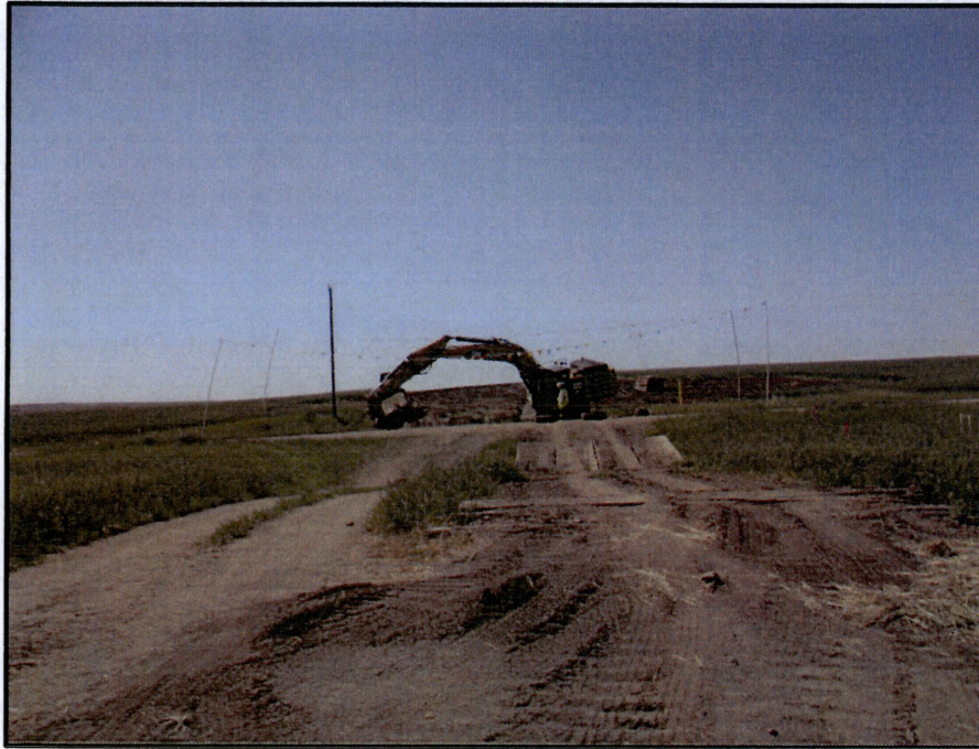
Photo 5. (GPS Point #447) – Excavator removing mats from road ditch (far side of the road), which was used for access to the ROW. Most of the topsoil had been replaced in this area. Direction: South
