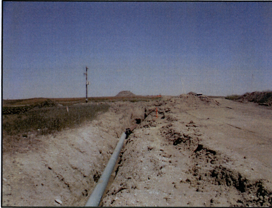
Photo 13. (GPS Point #444) - Area near rural water line break. Open trench to the left of photo. No standing safety fence observed. Environmental inspector thought they hit the rural water line while they were doing boring activities. Direction: North
