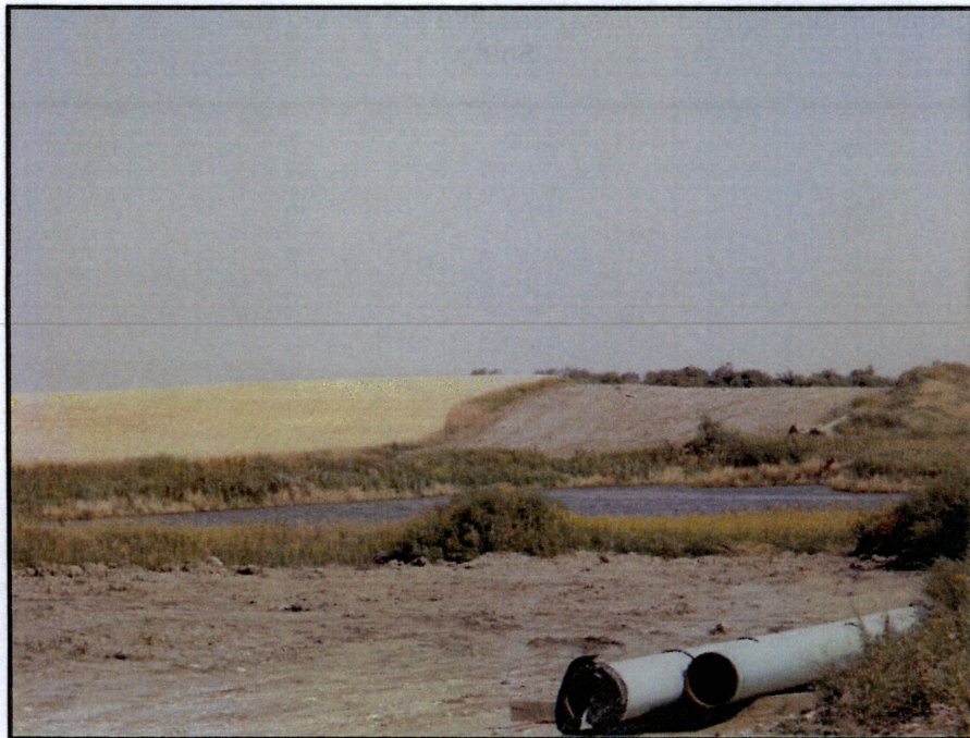
Photo 22. (GPS Point #485) - Pipeline ROW goes down the hill in the distance and wetland was bored under. No erosion control devices observed. Direction: North
