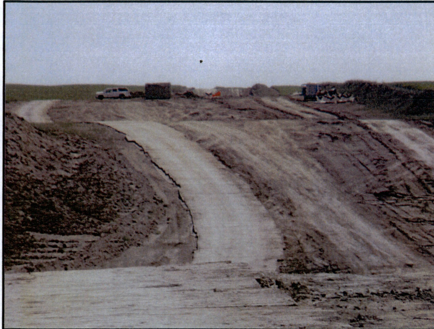
Photo 9. (GPS Point #449) – ROW going up to Lake Sakakawea bore area. The bore contractor wanted mats placed on ROW up to bore area. Mats are observed on the left side of the ROW. Direction: East
