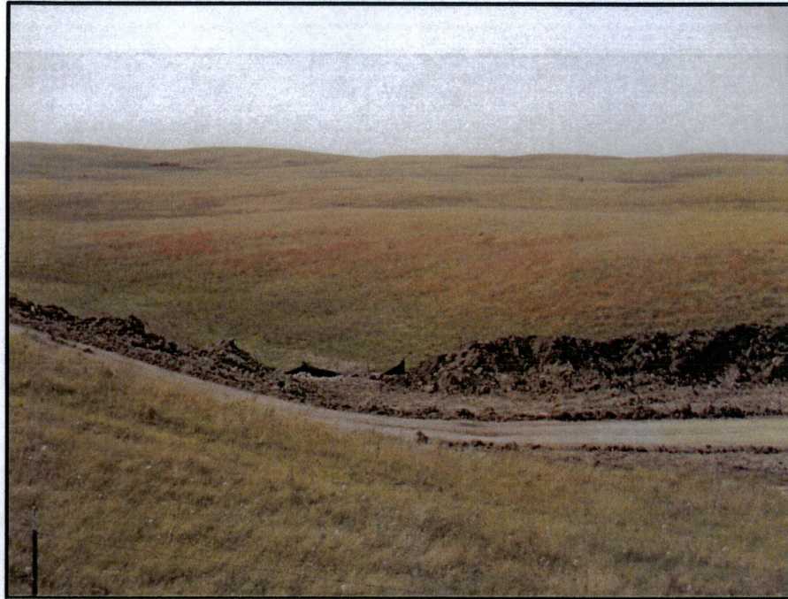
Photo 21. (GPS Point #484) - Silt fence in drainage area, needs maintenance. Direction: South
