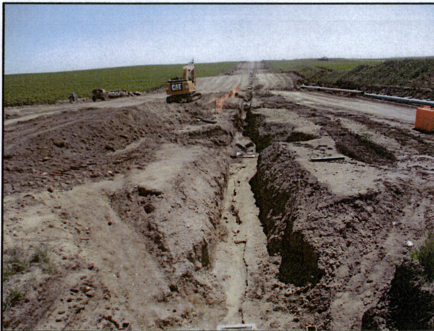
Photo 12. (GPS Point #450) - Open trench with few orange blockades ending to the right of photo, and only partial orange fence to the left of trench. White and black pipe rollers in trench were used to guide bore pipe. Photo taken from bridge shown in photo #11. Direction: East
