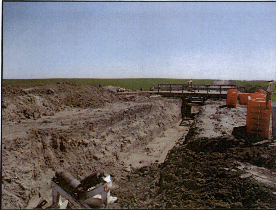
Photo 11. (GPS Point #450) - Open trench with orange blockades to the right of photo, trench spoil to the left. White and black pipe rollers in foreground were used to guide bore pipe. Bridge was used for a vehicle crossing to get to the bore area. Direction: East
