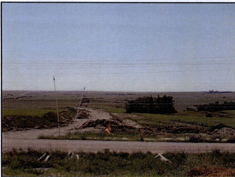
Photo 14. (GPS Point #444) - Area near rural water line break. Extended ROW for bore area. Topsoil pile to the left of photo on left side of ROW with vegetation growing on it. Direction: South
