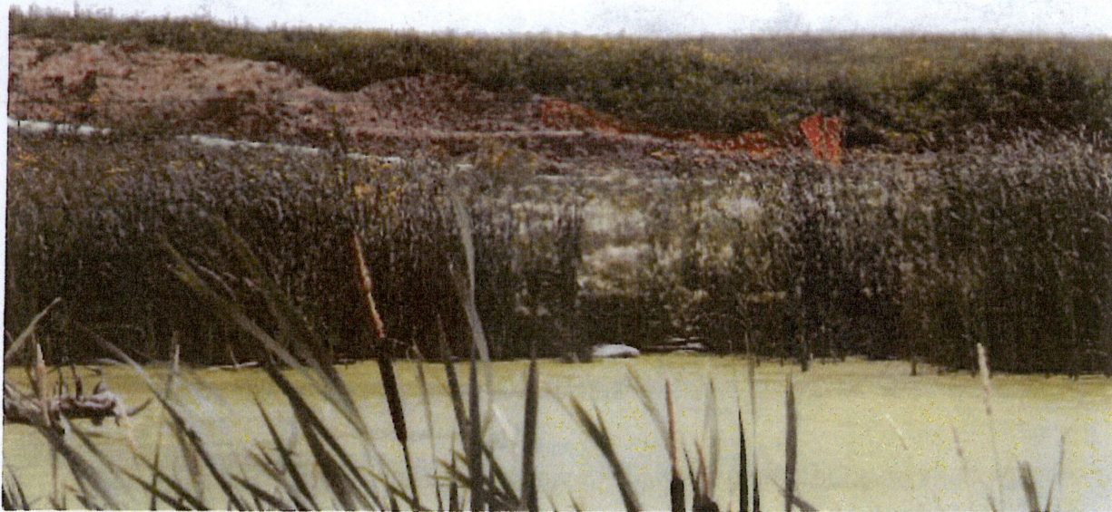
The next two photos, taken at a location east of 87 th Avenue on an unnamed road in Mountrail County, show an area where silt fence was installed but then evidently run over and neglected.
