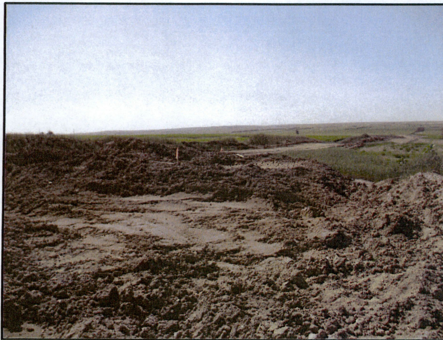
Photo 15. (GPS Point #444) - Area near rural water line break. Looks like subsoil had been pushed around, there was some ponded water in back of photo. Direction: South
