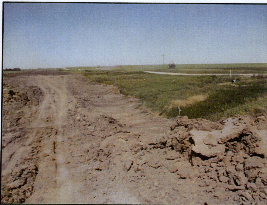
Photo 4. (GPS Point #446) - Drainage area intersected by ROW. Pipe trenched and backfilled along the edge of the ROW. The drainage area appeared to be a potential wetland. Notice the vegetation change. However, the environmental inspector stated it was not a wetland. No erosion control devices were observed. The PSC was informed of this site the day after the inspection.
