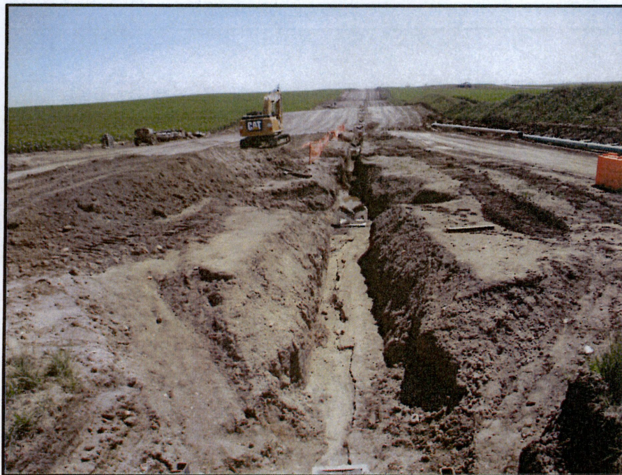
Photo 12. (GPS Point #450) - Open trench with few orange blockades ending to the right of photo, and only partial orange fence to the left of trench. White and black pipe rollers in trench were used to guide bore pipe. Photo taken from bridge shown in photo #11. Direction: East
