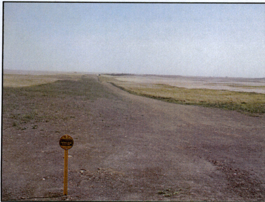
Photo 24. (GPS Point #490) - Pipeline ROW has vegetation growing. Looks like the right side of the ROW, where no vegetation is growing, has been/or is being used as a travel lane. Direction: East
