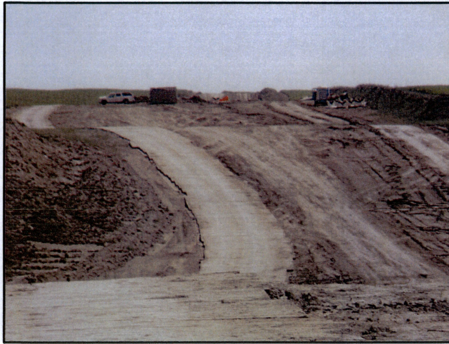
Photo 9. (GPS Point #449) – ROW going up to Lake Sakakawea bore area. The bore contractor wanted mats placed on ROW up to bore area. Mats are observed on the left side of the ROW. Direction: East
