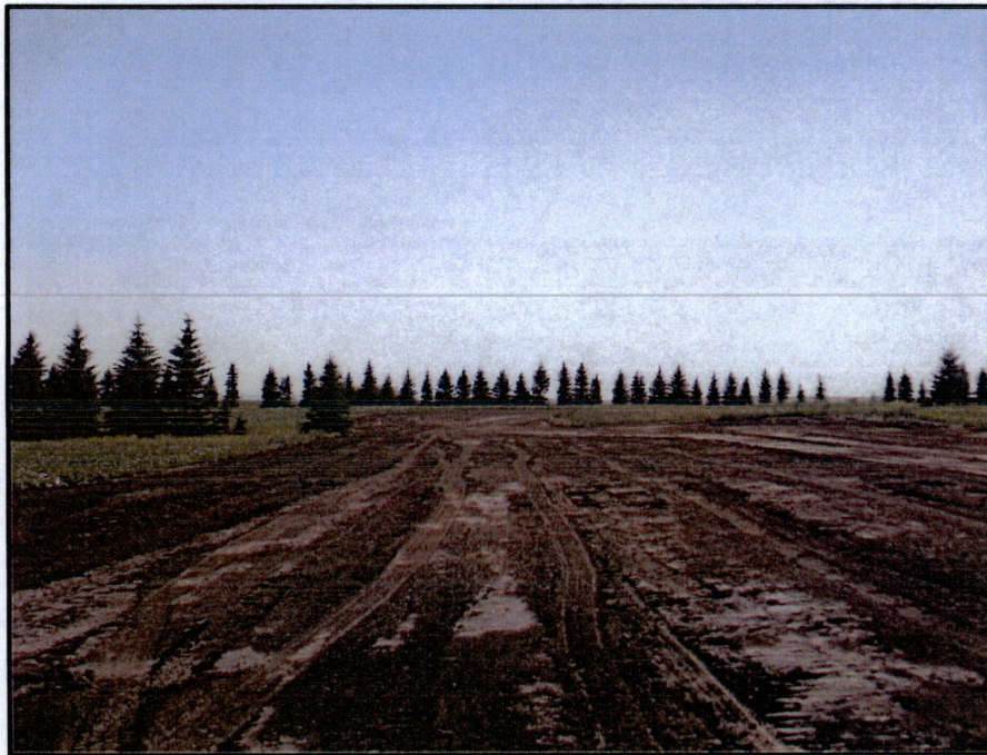
Photo 6. (GPS Point #448) – ROW necked down to 50 ft width through tree rows. Unknown if or how many trees were taken out in this area. Topsoil replaced back on the ROW. Direction: East.
