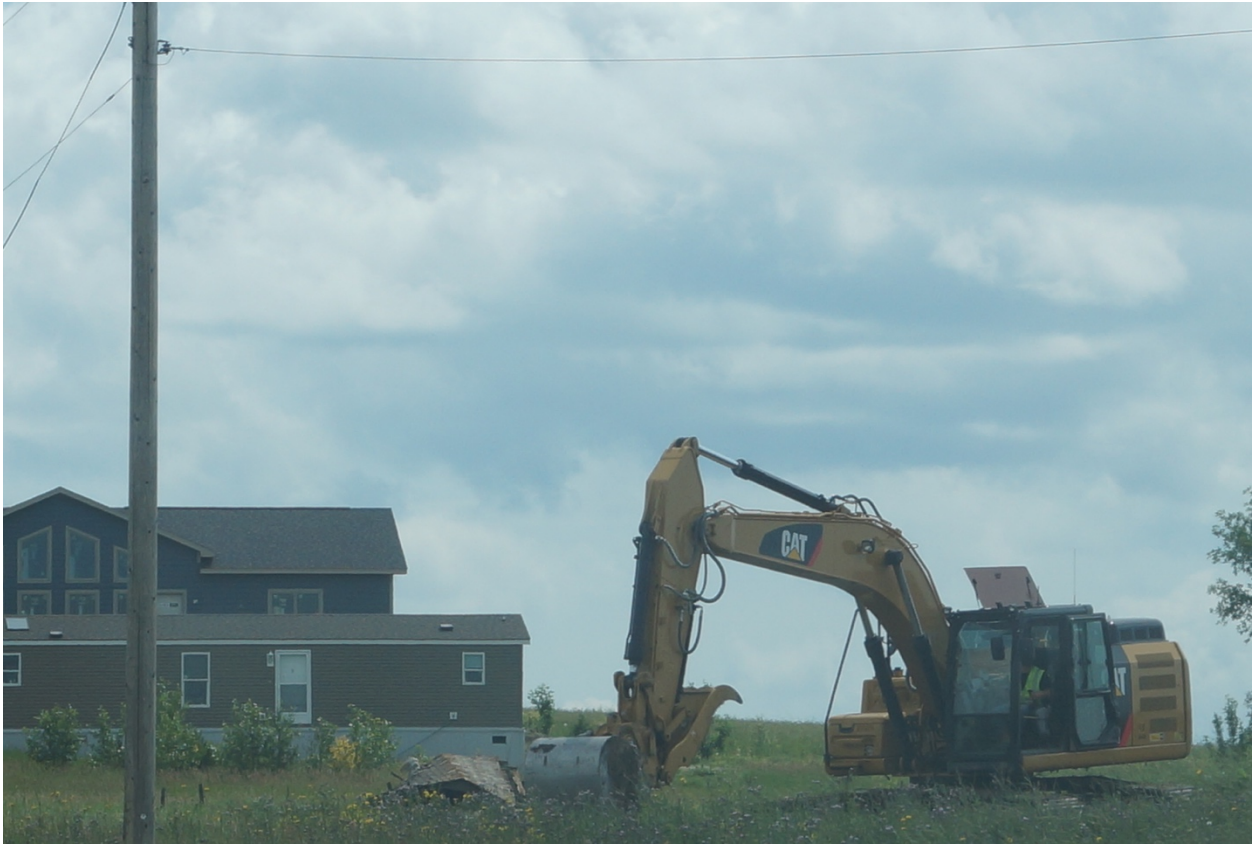
Photo of Sacagawea Pipeline construction near 53 rd Street NE east of Highway 8 in Mountrail County on July 14, 2016
