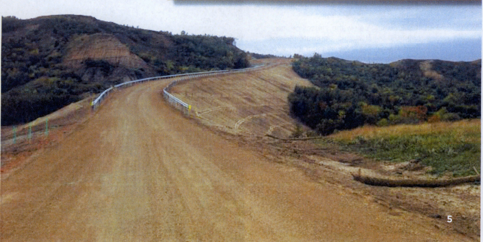
Example of construction and reclamation of an access road during and after construction.
