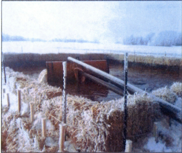
Hydrostatic Test Water Discharge Structure
