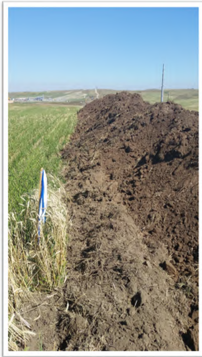
Figure 7. View from western pipeline right of way edge looking north. Topsoil stockpiled along western edge of right of way.
