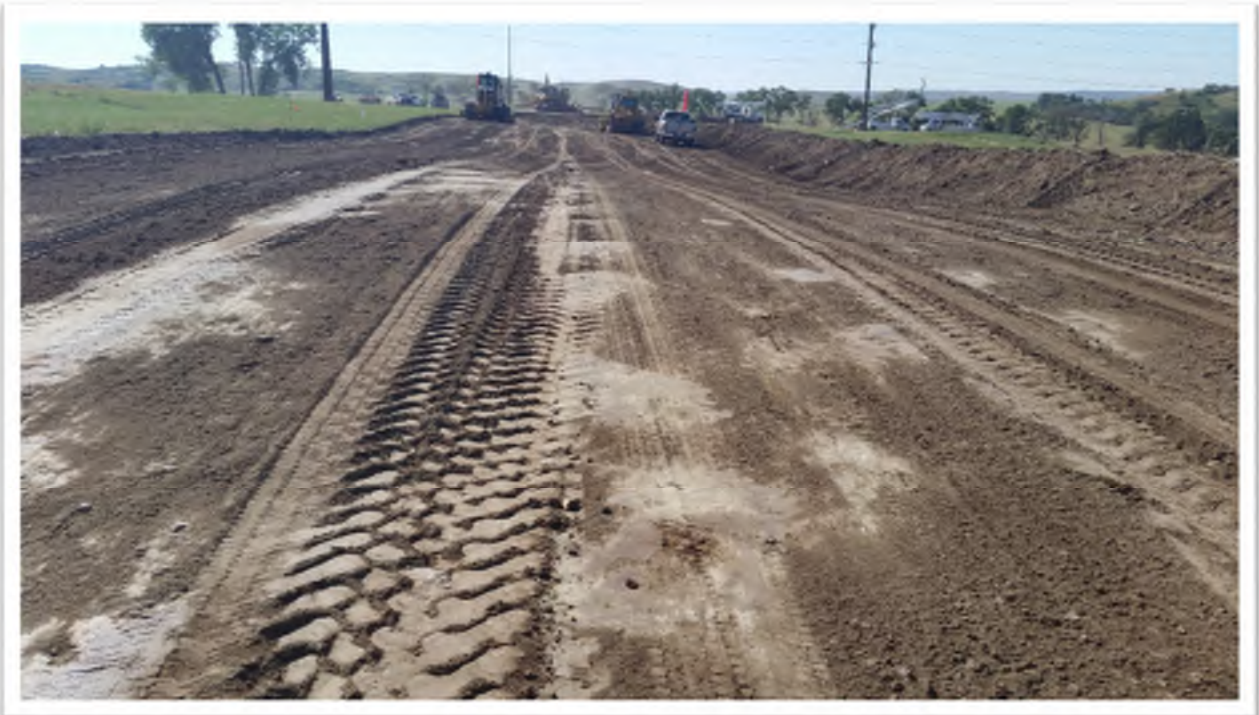
Figure 6. View from pipeline right of way looking south. Topsoil stockpiled along western edge of right of way.
