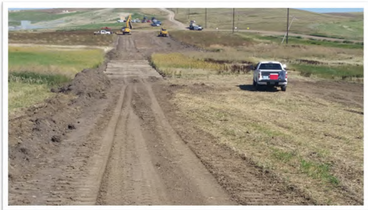
Figure 2. View looking north at WET1. Construction matting across WET1, topsoil on right side of image will remain in place since this segment is to be directionally drilled.
