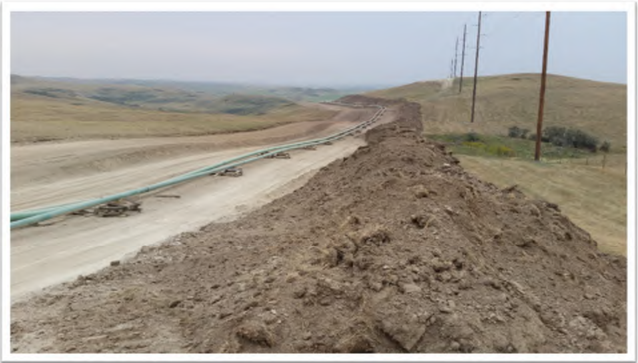
Figure 7. View from western pipeline right of way edge looking south. Topsoil stockpiled along western edge of right of way.
