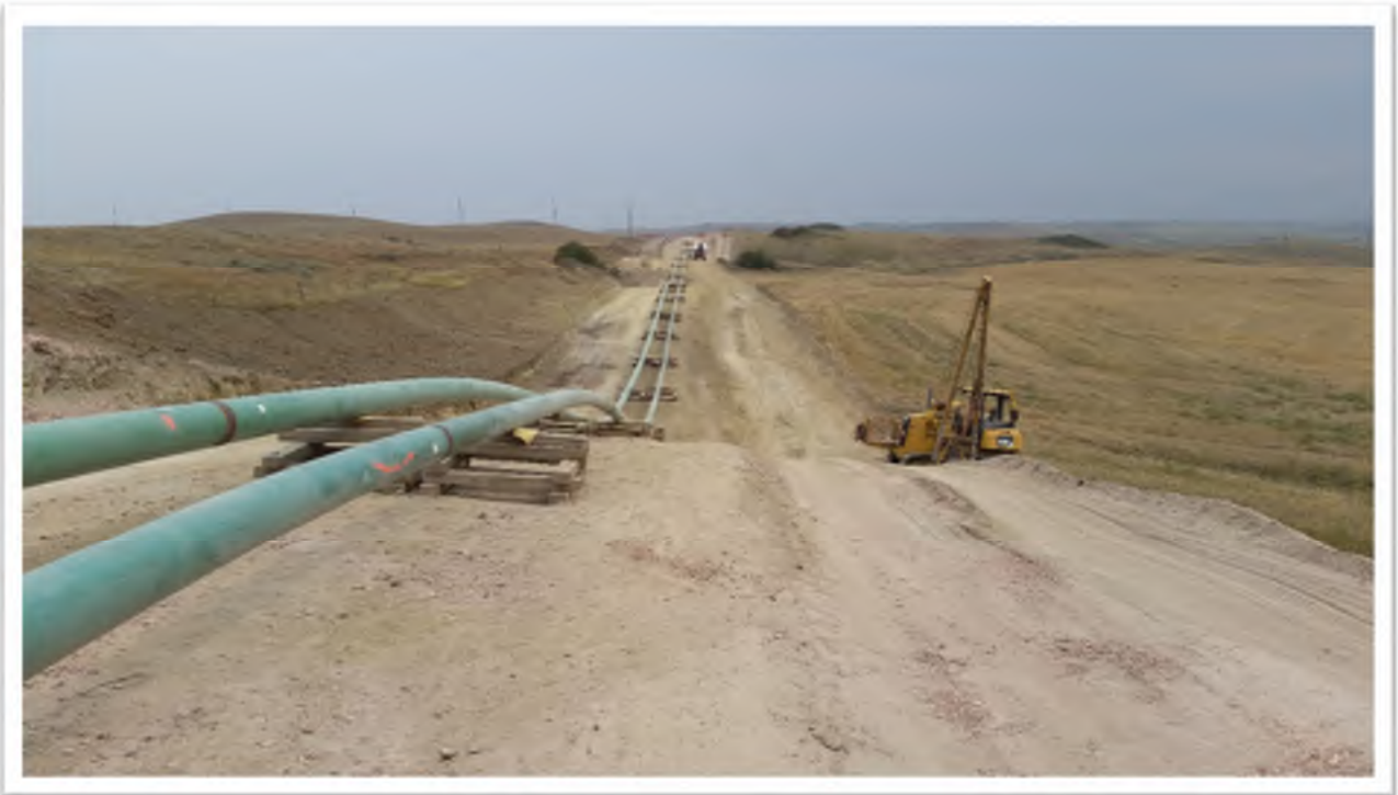
Figure 9. View from pipeline right of way looking east at pipeline string operations. Topsoil stockpiled along northern edge of right of way.
