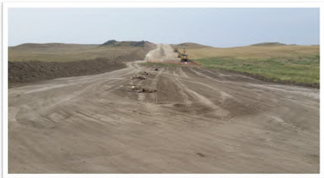
Figure 10. View from end of pipeline route near NGL plant looking east. Topsoil stockpiled along northern edge of right of way.
