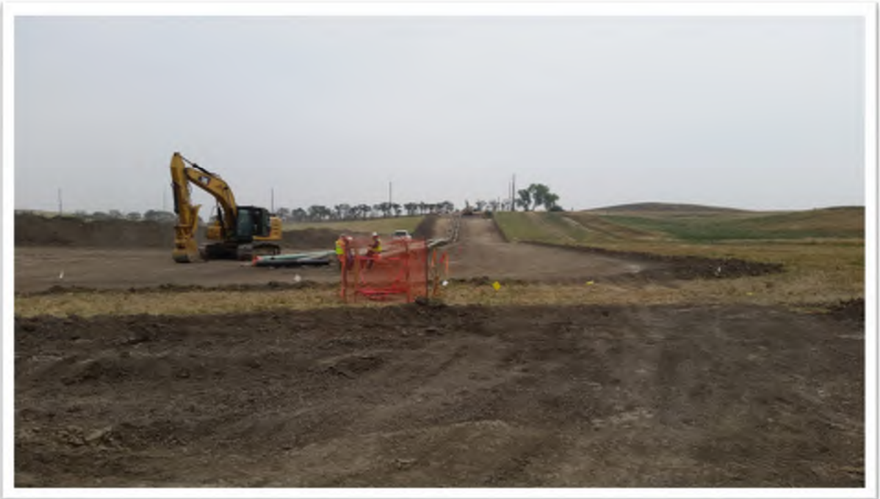
Figure 5. View from pipeline right of way looking north. Topsoil stockpiled along western edge of right of way.
