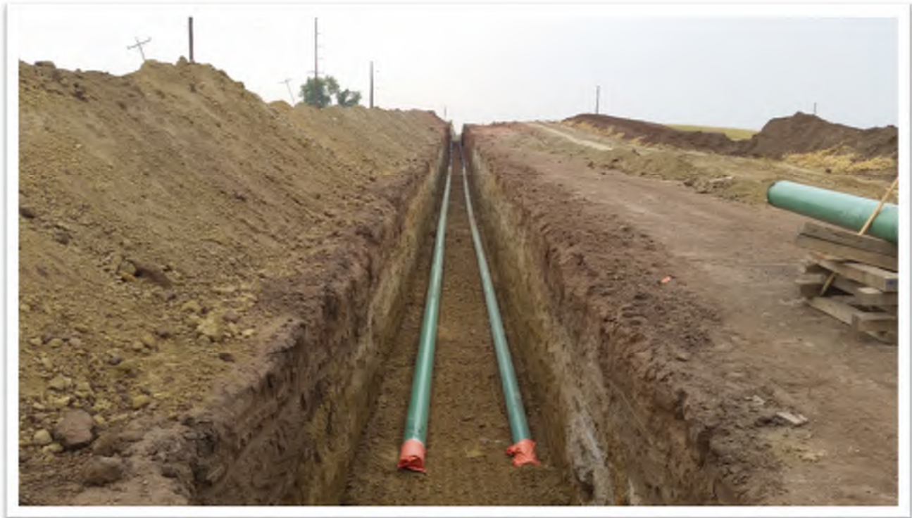
Figure 3. View of installed 10" and 8" pipelines looking south. Two feet of separation between pipelines and 7.5' depth of cover.
