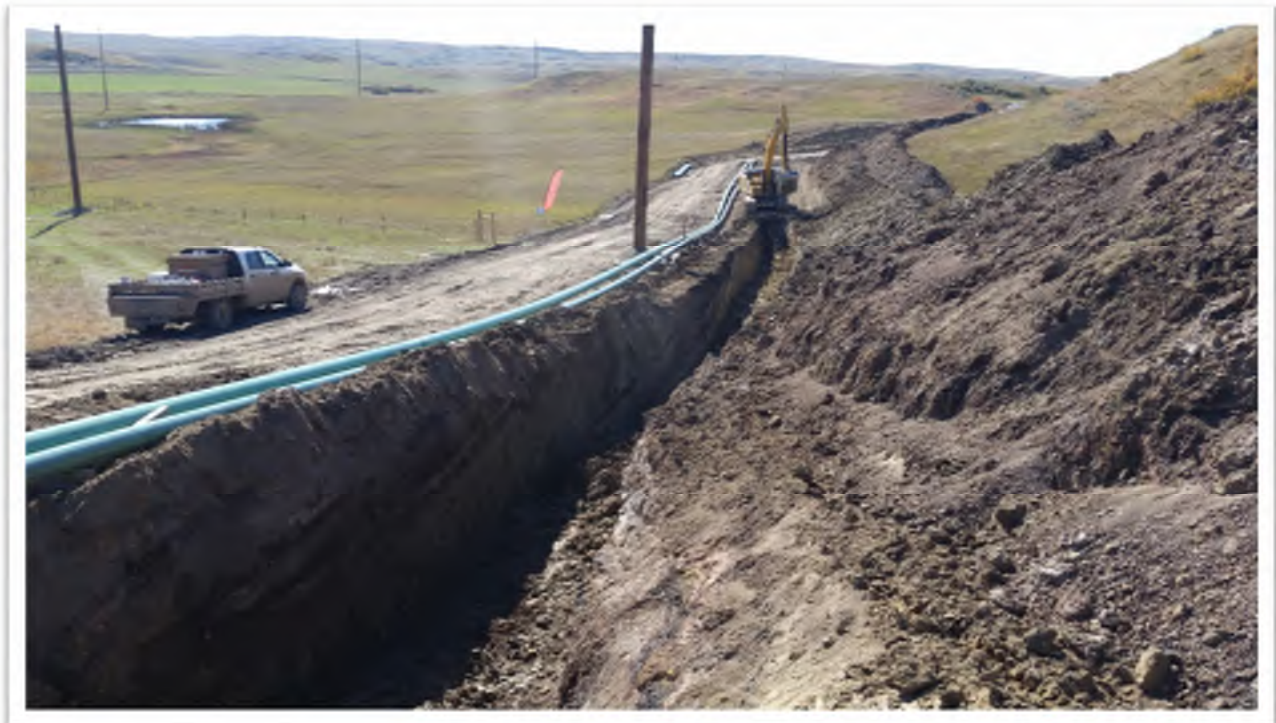
Figure 6. View of tie-in location where subgrade and topsoil spoil piles are being stored without separation.
