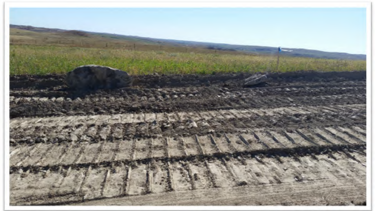
Figure 4. Boulders encountered during earthwork operations.
