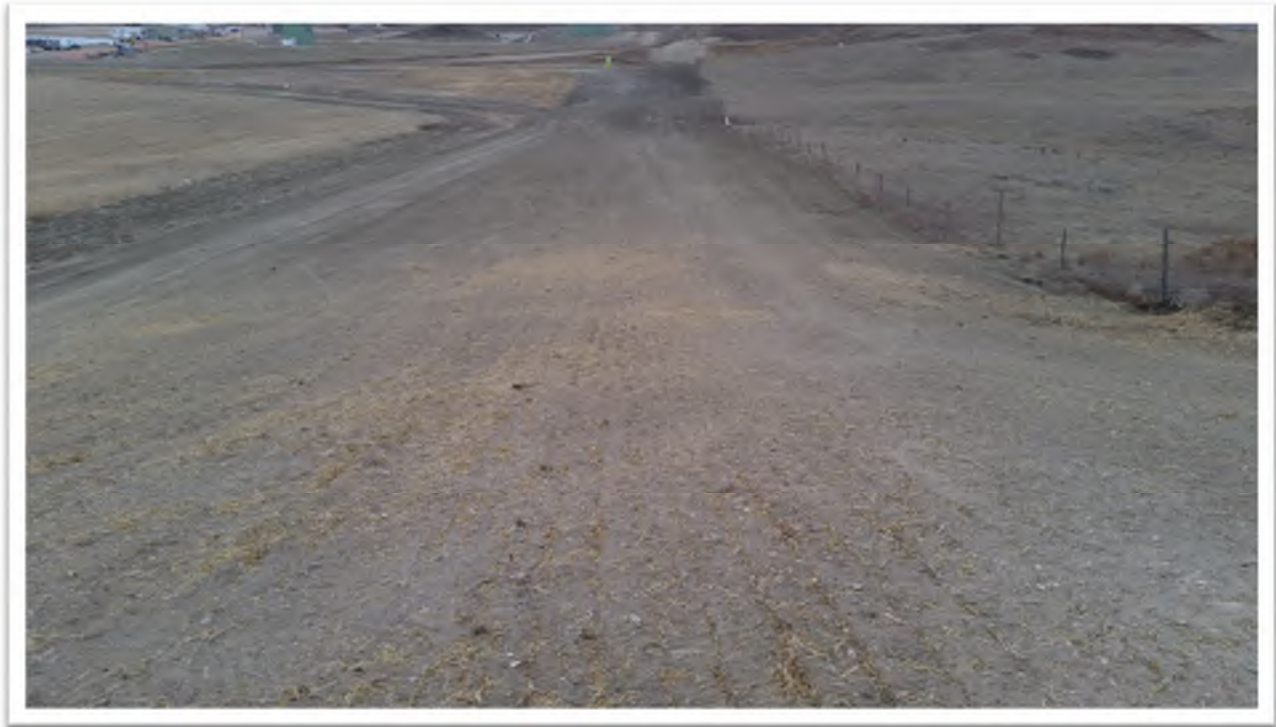
Figure 7. View of agricultural land topsoil blended back into original contours looking west.
