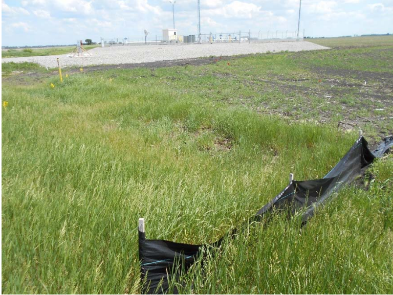
Photo 16: Fargo Terminal silt fencing.
