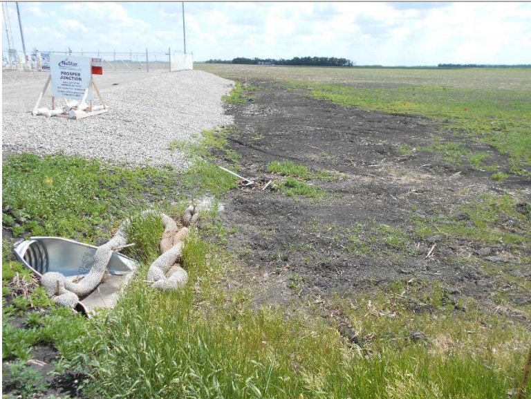
Photo 12/13: Pipeline corridor at Fargo Terminal at the intersection of 32 nd St SE and 166 th Avenue SE. Facing south. Erosion control features can be seen in the foreground near the newly installed culvert.
