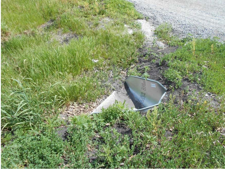
Photo 14: Culvert at Fargo Terminal. No erosion / sedimentation issues, or bare ground observed.
