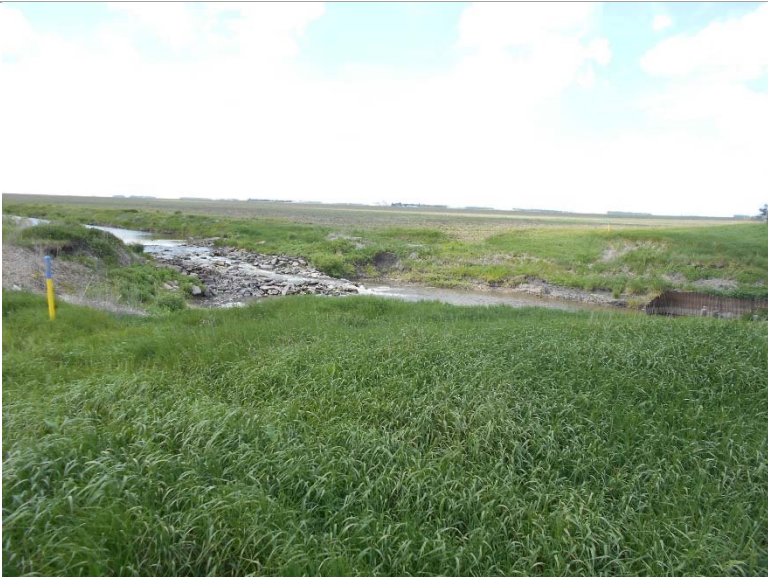
Photo 22 / 23: Project Corridor at Maple River crossing. Horizontal Directional Drilling was used to span the river.
