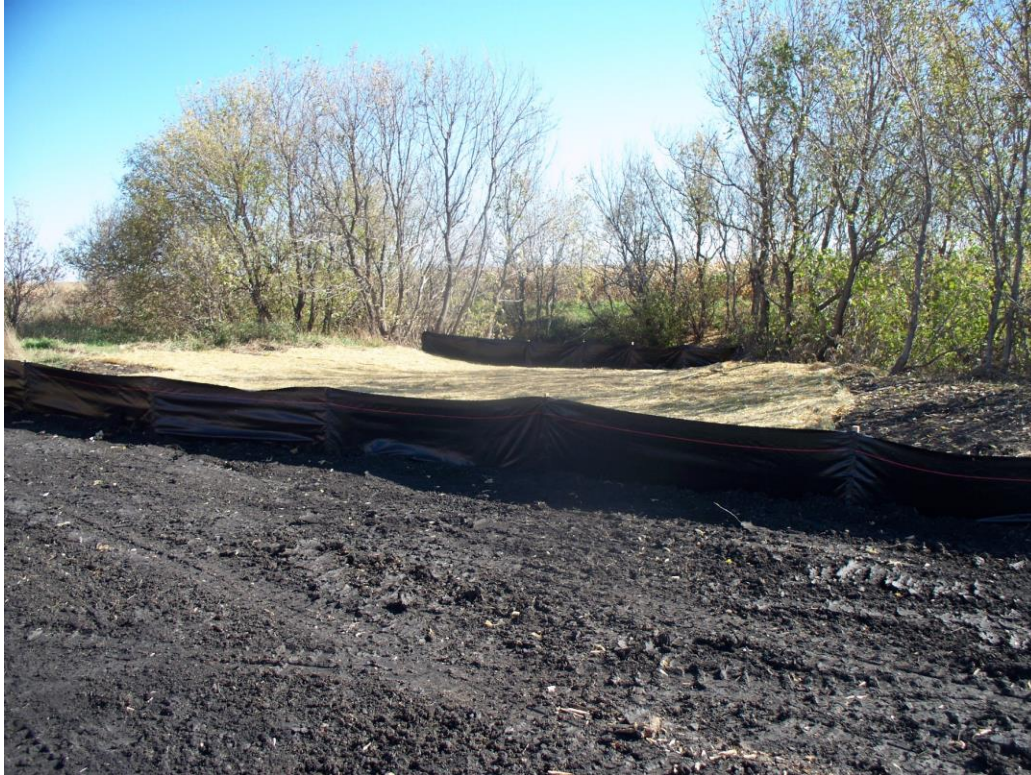
Silt fence and erosion control blanket installed near tributary to the Sheyenne River
