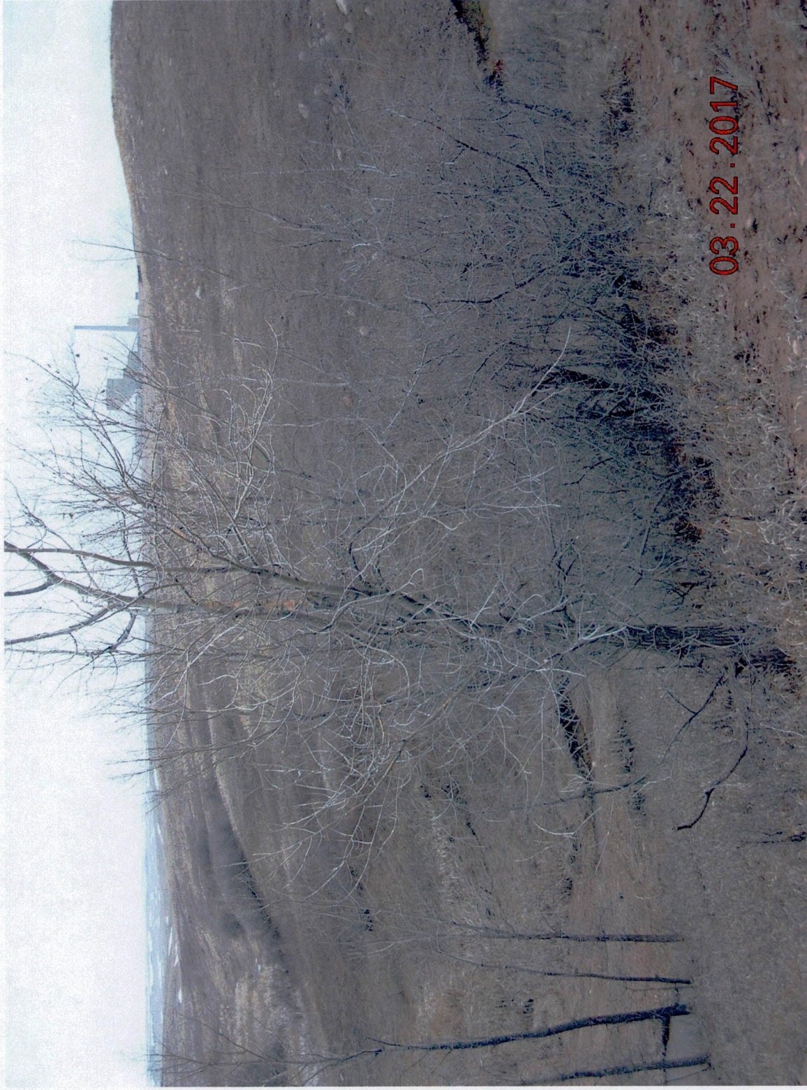
Figure 14b. Erosional gully in foreground and siltation in intermittent stream on left - facing northeast with Coyote Station in background - rotate north (left) with following Figure 14c or east (right) with preceding Figure 14a.
