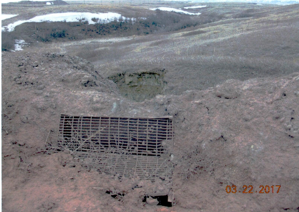
Figure 12. Uncontrolled haul road runoff flow over or through the north haul road berm at the drainage grate location - facing north with headward extent of erosional gully in background - see Figure 9 for location.
