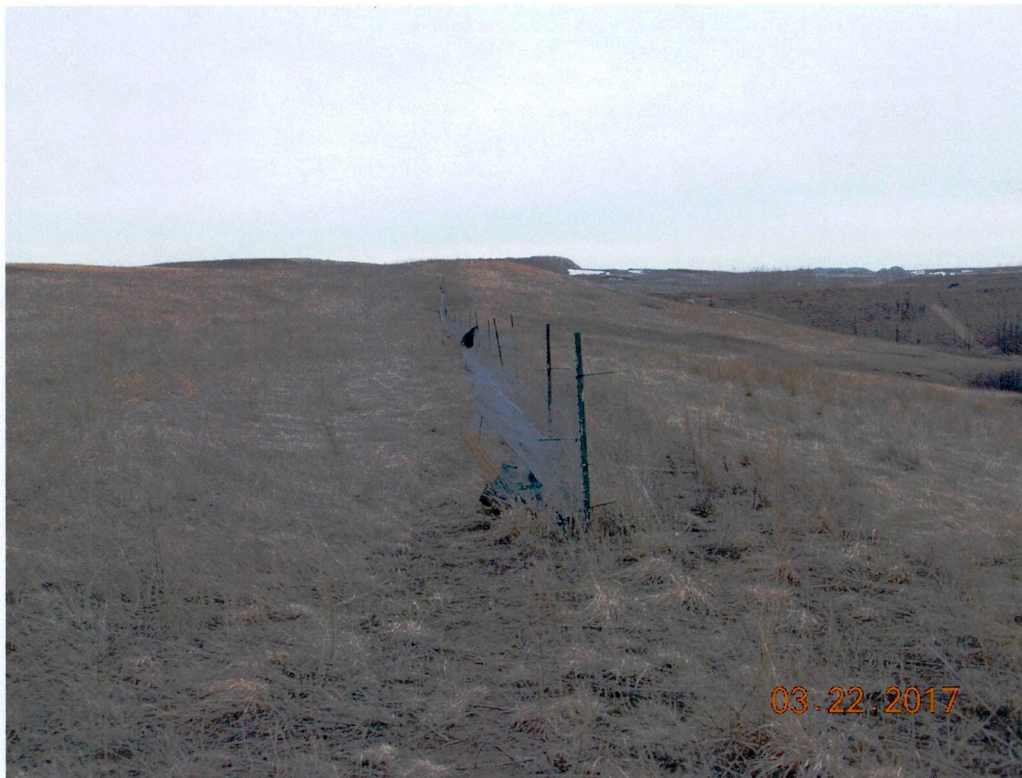
Figure 6. Silt fence installed at the mining disturbance boundary along the east bank of the undisturbed intermittent streambank in the SW¼ of Section 15 for grade approval areas Gold2-2011 and Gold1-2009 - facing south - see Figure 1 for location.
