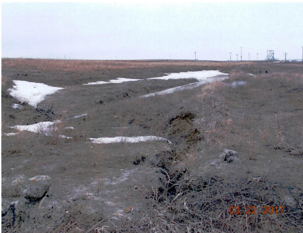
Figure 2. Special Variance Zone #7 spoil stockpile sump overflow to an adjoining linear sump to the north that was apparently installed to detain runoff from reclaimed land - facing north - see Figures 1 and 8 for location.
