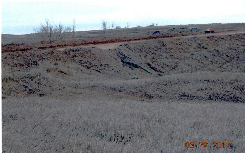
Figure 13. Uncontrolled haul road runoff flow over or through the north haul road berm at the drainage grate location as viewed from the intermittent stream's east bank - facing southwest with DWC pickup truck parked on south haul road shoulder.
