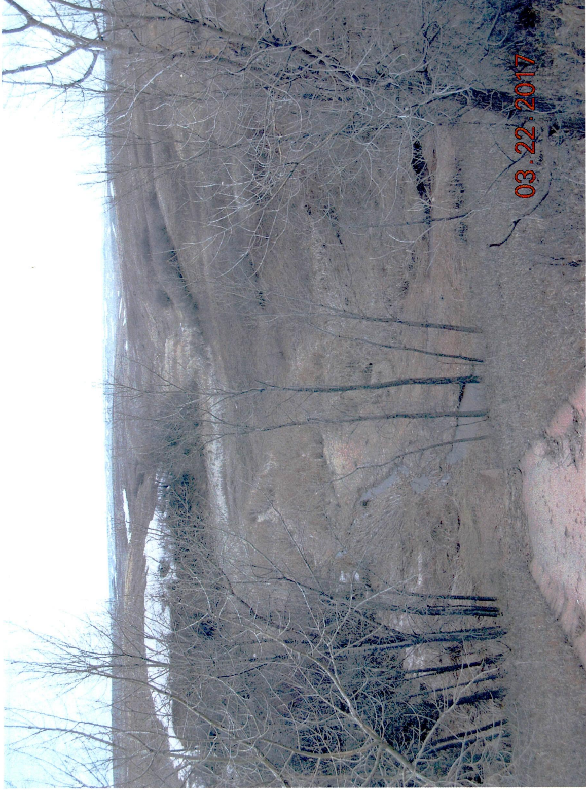
Figure 14c. Intermittent stream siltation in center - facing north with obsolete concrete drainage channel in foreground - rotate northeast (right) with preceding Figure 14b.
