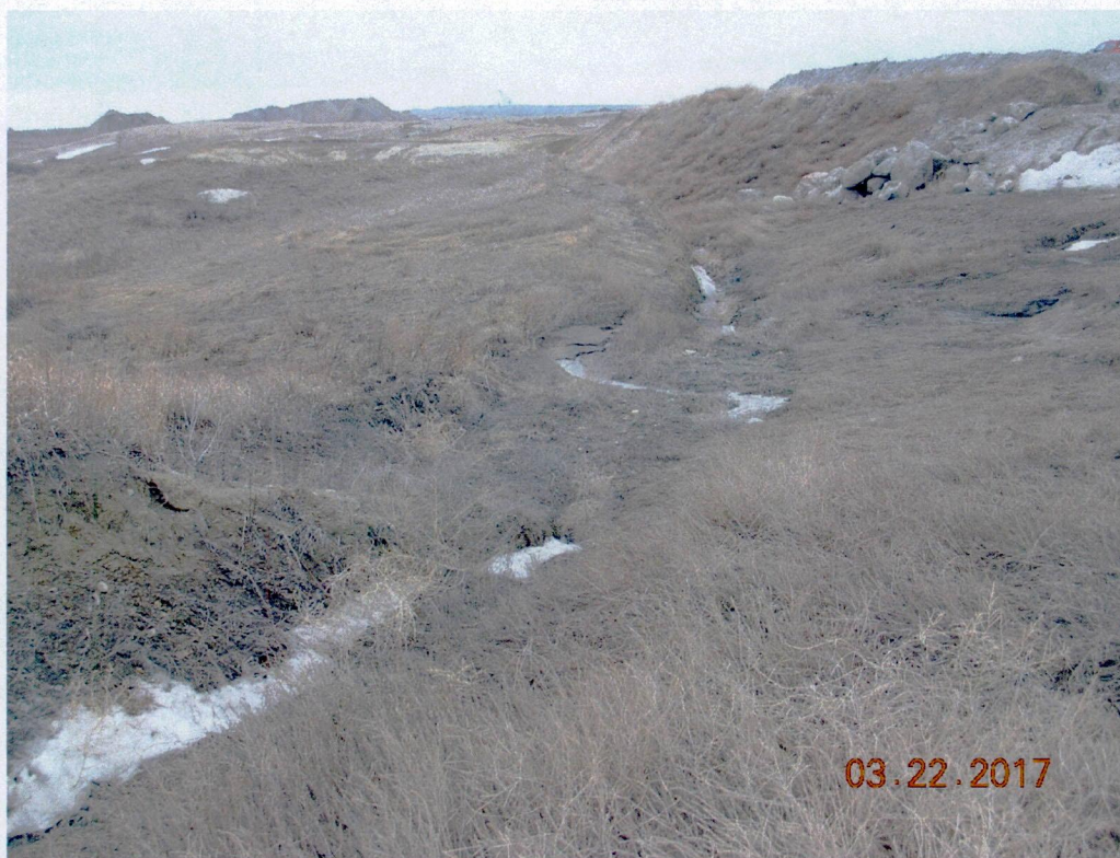
Figure 4. Sediment accumulated in Diversion 99E-B about 150 feet east of Sump 99E where sediment laden runoff is at risk of overtopping the diversion and causing sediment deposition in the undisturbed intermittent stream buffer zone to the south - facing west with Sump 99E in background - see Figure 1 for location.
