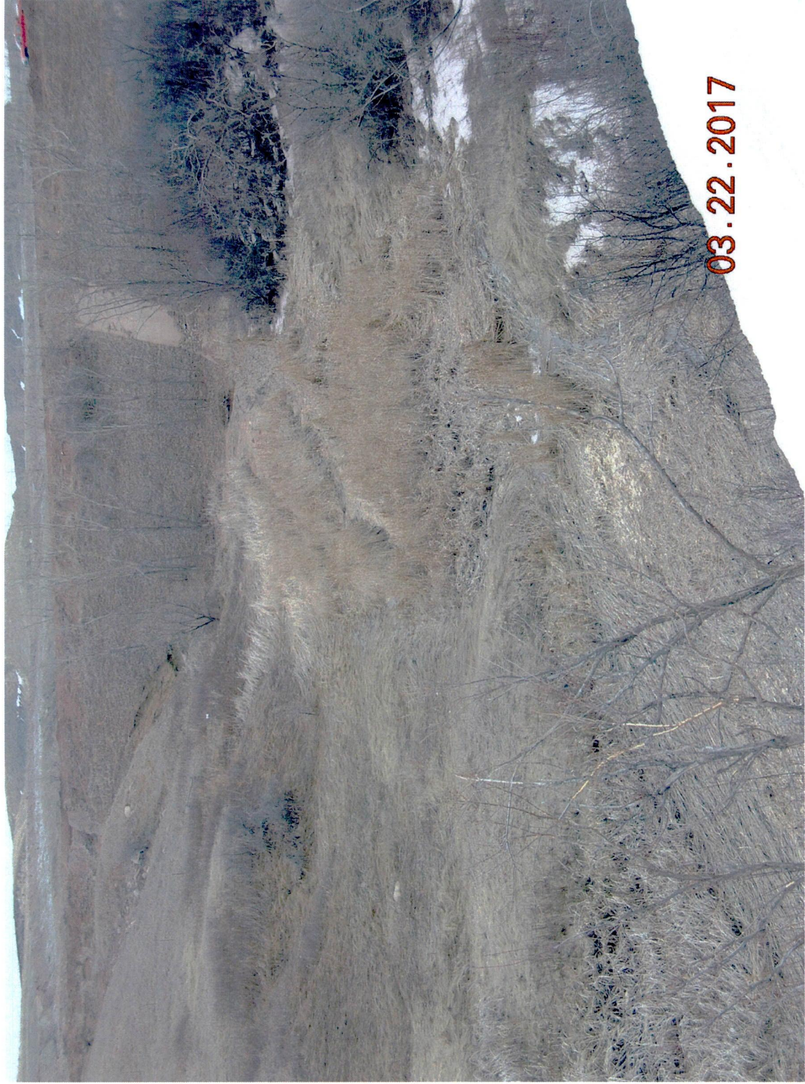
Figure 15. Overview of haul road runoff erosional gully (left background), siltation in intermittent stream (center foreground), and obsolete concrete drainage channel (center background) as viewed from the intermittent stream's west bank about 600 feet north of the haul road - facing south-southeast with DWC pickup truck parked on south haul road shoulder.
