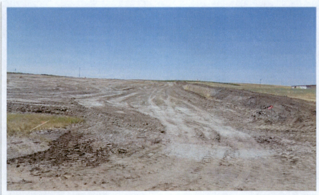
Figure 2. View from northcentral portion of the construction site, looking west. Topsoil removal progress.
