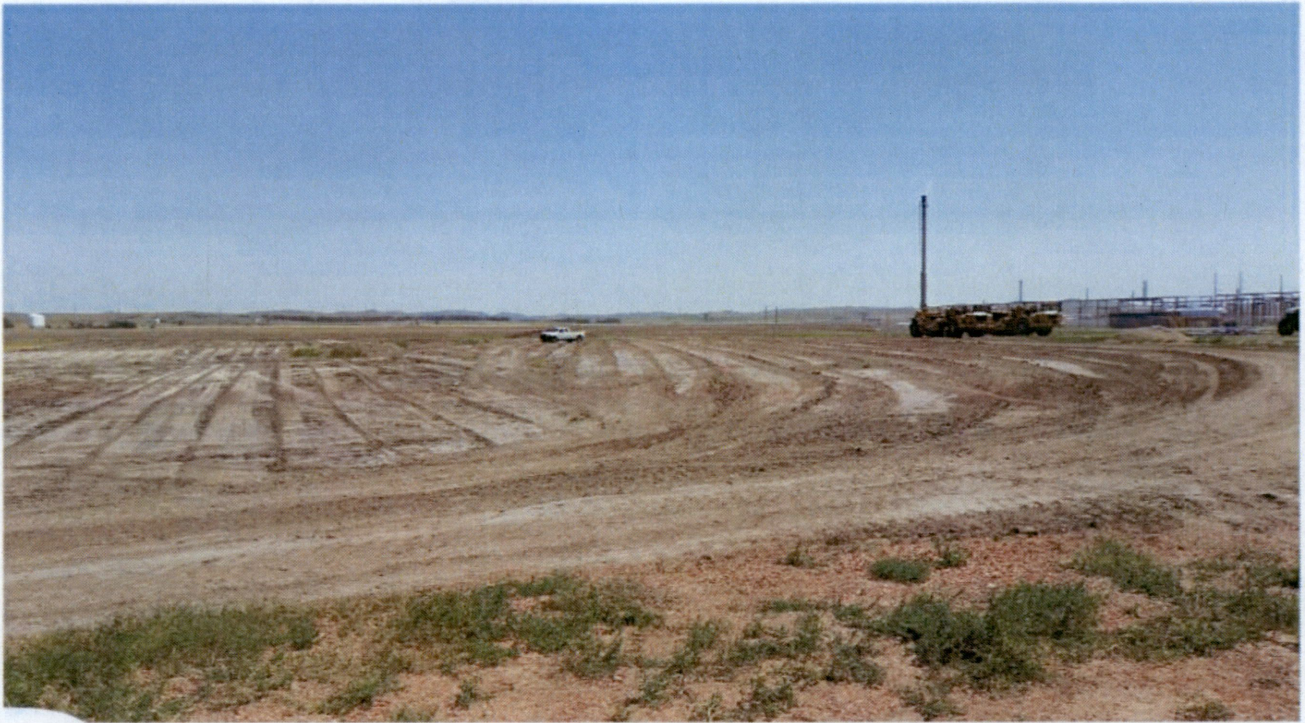
Figure 1. View from northcentral portion of the construction site, looking east. Topsoil scrapers on the right and drainage swale to the left.
