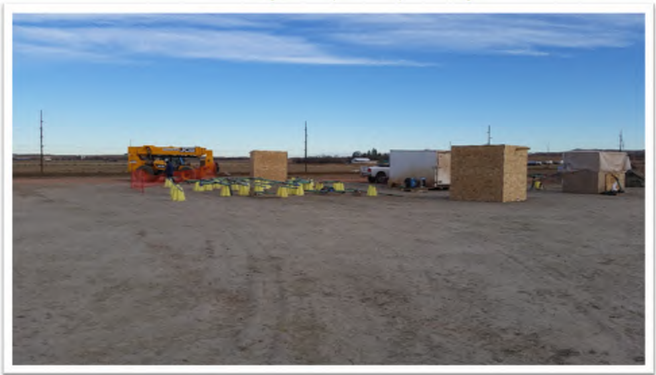
Figure 3. View from northeast portion of construction site, looking northeast. Future buried pipeline being assembled above grade.
