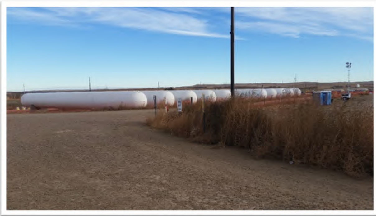
Figure 5. View from northwest portion of construction site, looking northeast. NGL storage tanks installed.
