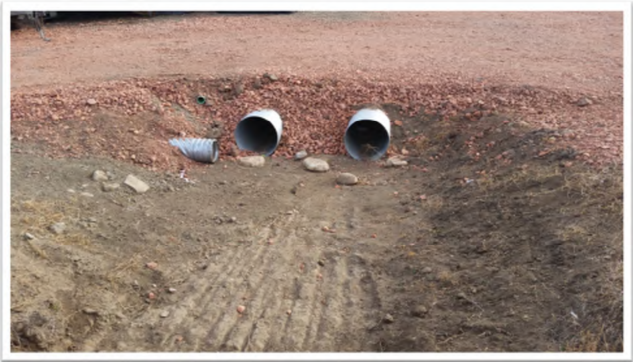
Figure 7. View from western portion of construction site, looking east. Storm water structures installed.
