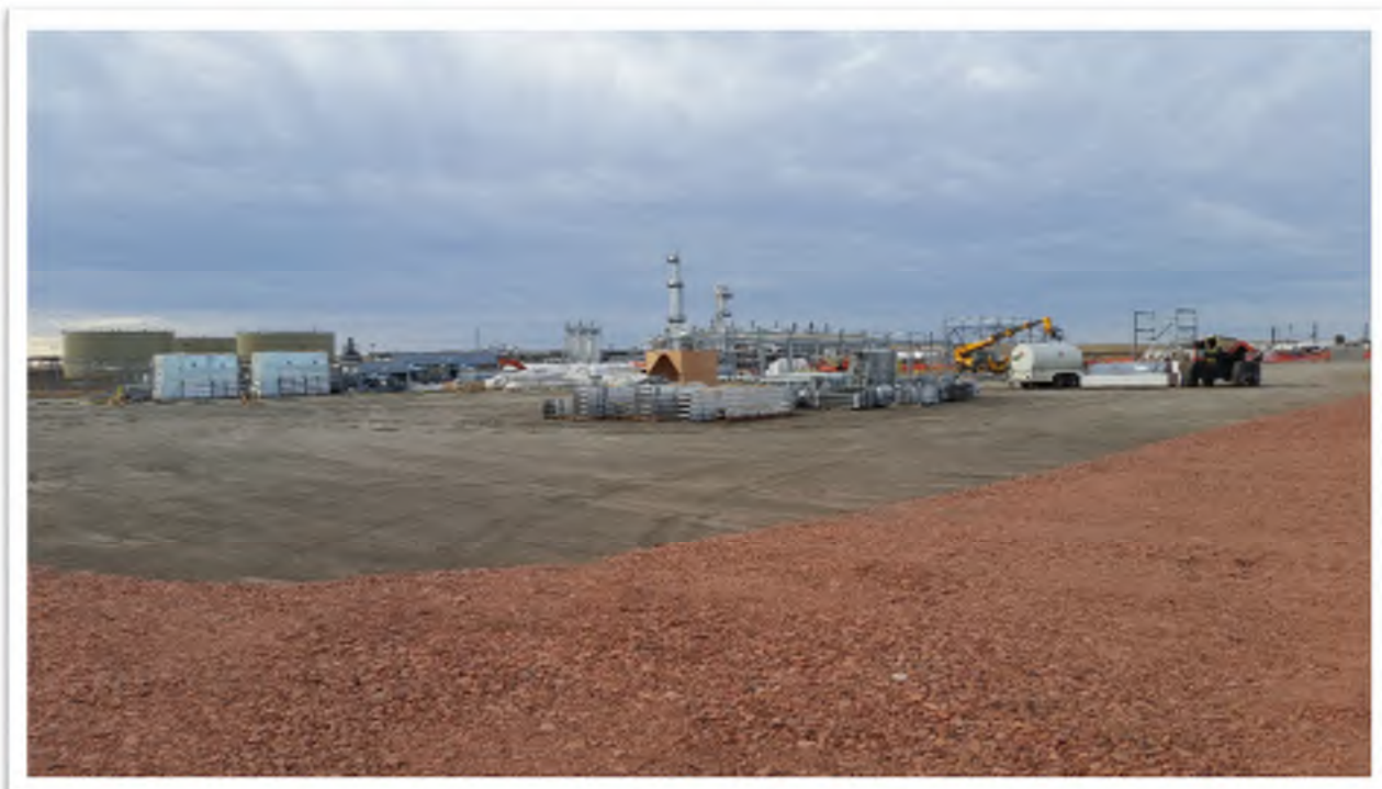
Figure 2. View from northeast portion of construction site, looking southwest. Stabilized Scoria road and site grading shown.
