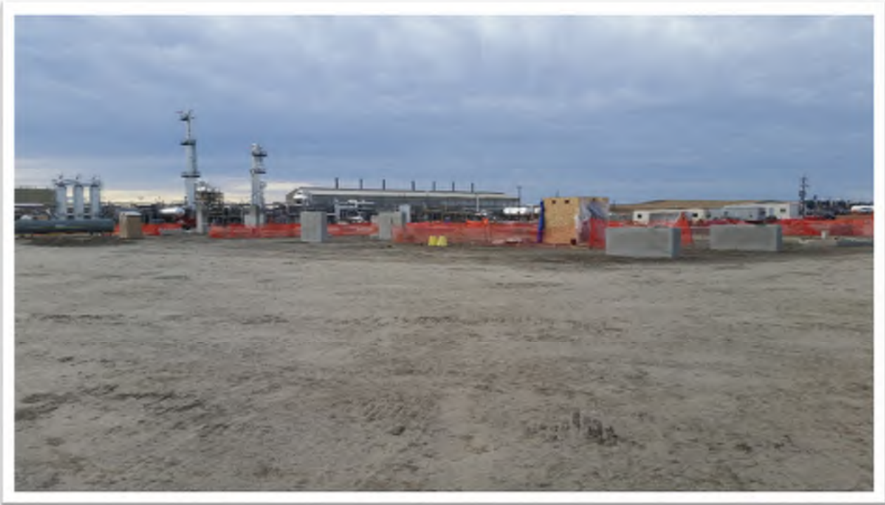
Figure 1. View from northeast portion of construction site, looking southwest. Poured equipment foundations and site grading shown.
