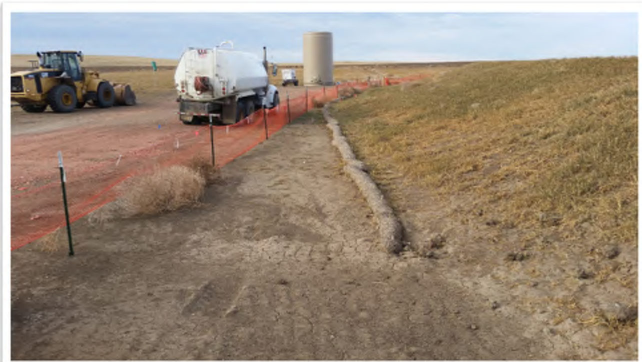
Figure 6. View from western portion of construction site, looking west. Erosion control measures shown.
