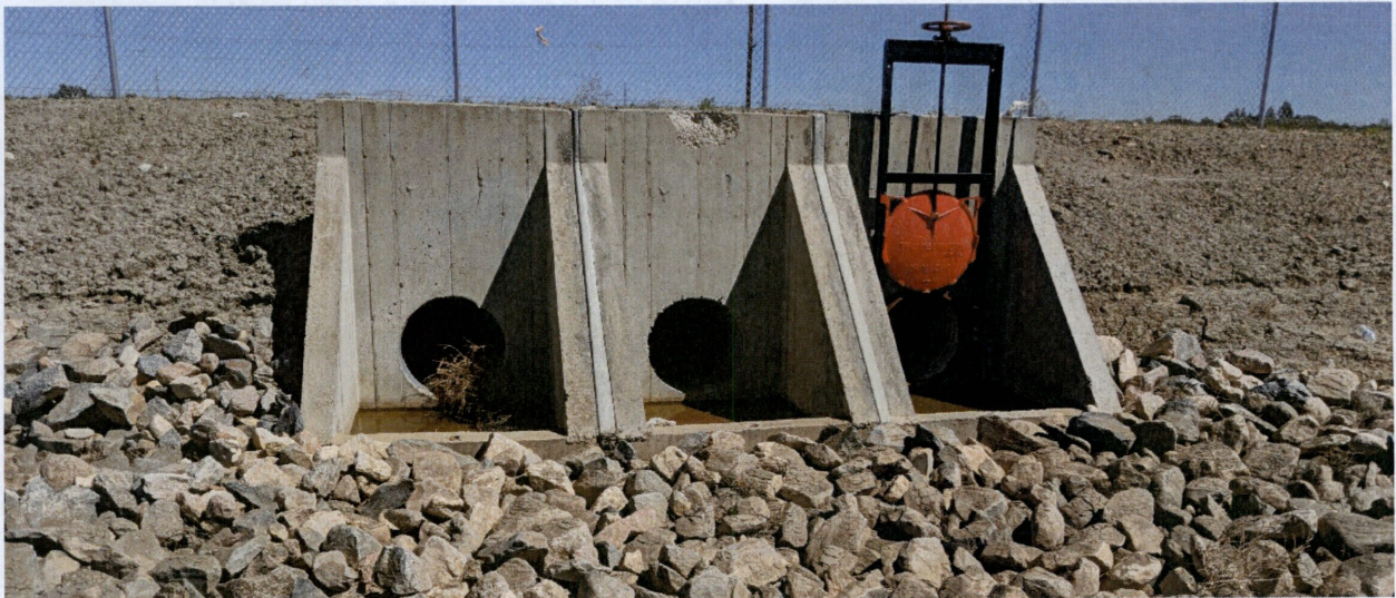
Figure 2. View from northeast portion of construction site, looking north at storm water control infrastructure.
