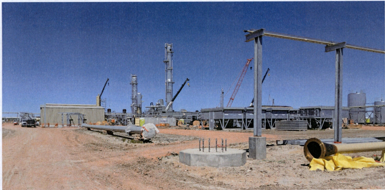
Figure 6. View from eastern portion of construction site, looking west at electrical and flare construction progress.
