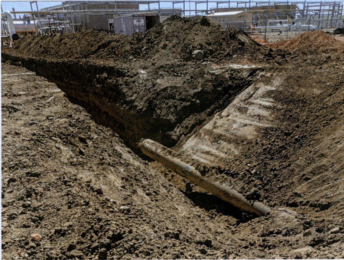
Figure 1. View from western portion of construction site, looking southeast at gas pipeline construction.
