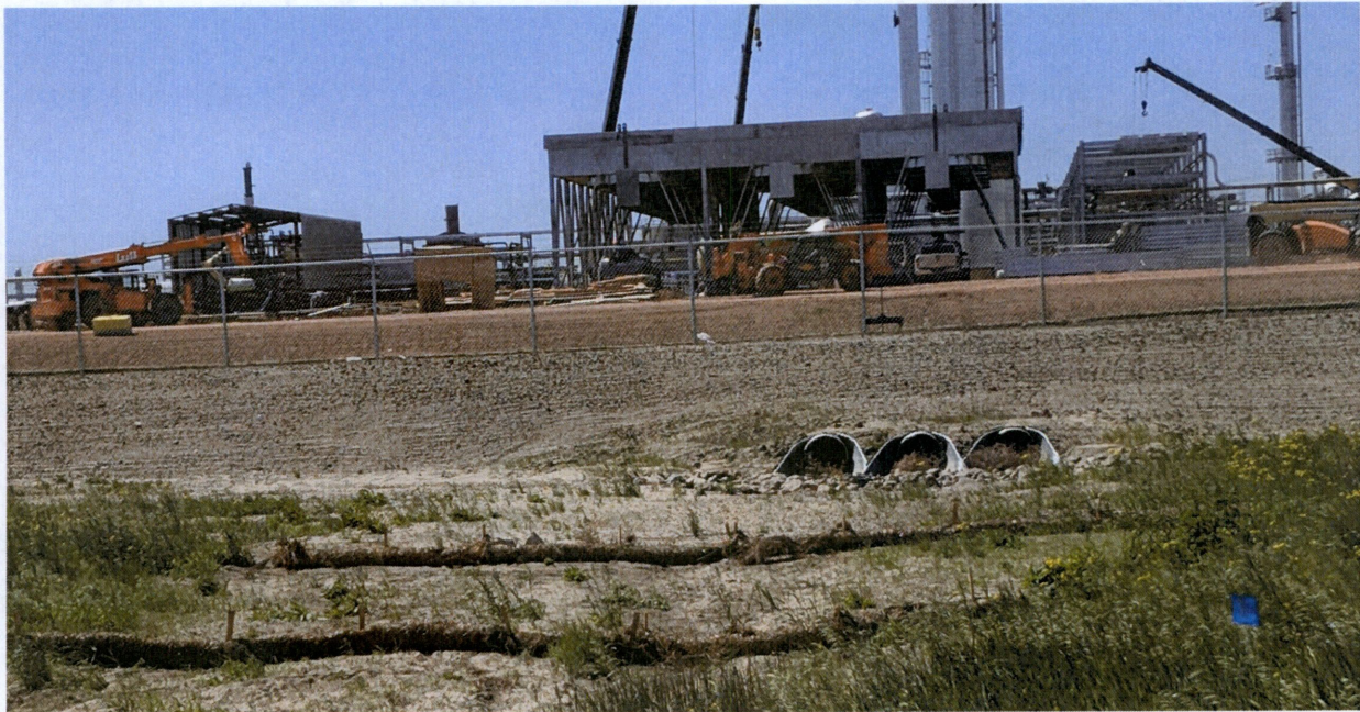
Figure 3. View from northeast portion of construction site, looking south at storm water control outlet and erosion control measures.
