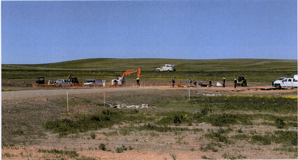
Figure 5. View from western portion of construction site, looking west at new location and construction progress of control room.
