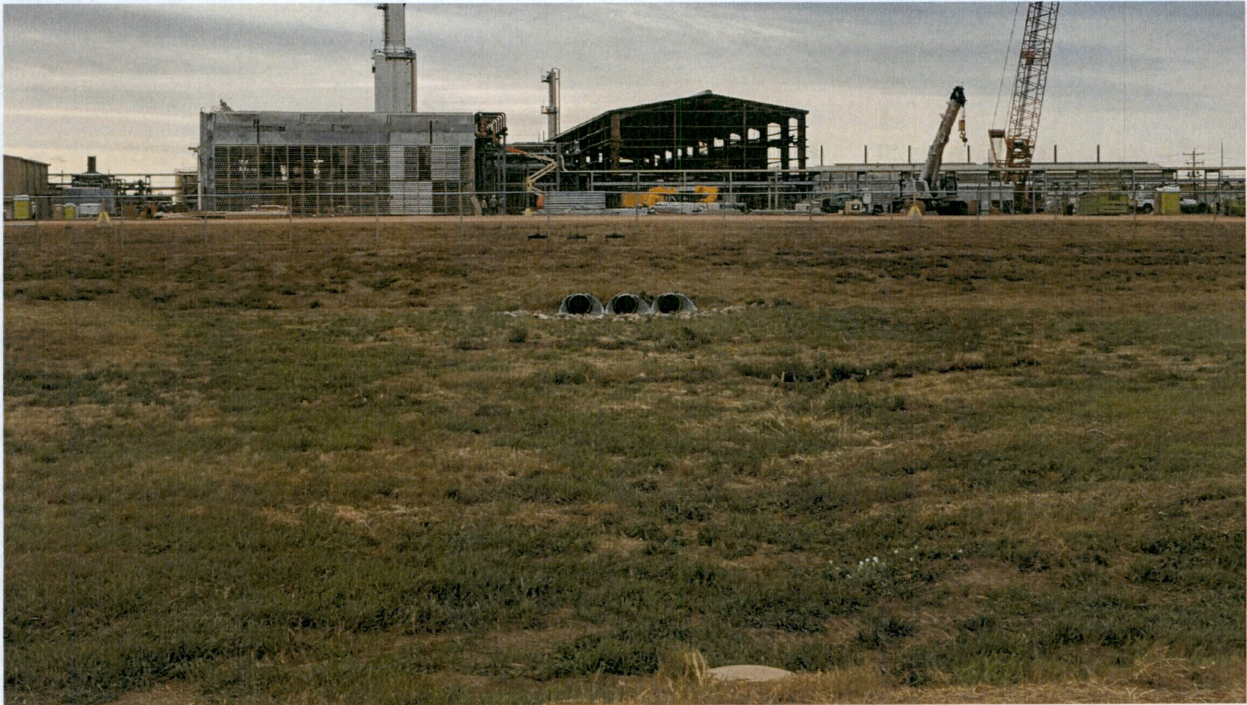
Figure 5. View from northeastern portion of construction site, looking south at storm water outlet revegetation progress.
