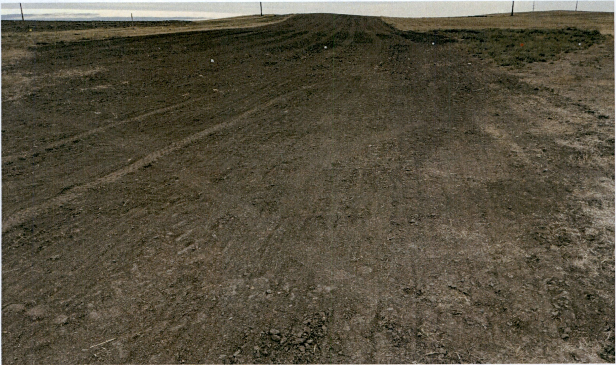
Figure 3. View from western portion of construction site, looking south at seeded gas pipeline right-of-way.
