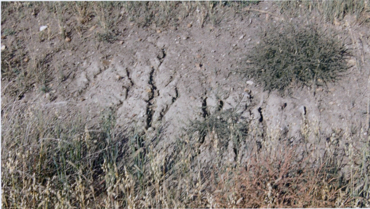
Figure 4. View looking west with good vegetation above the ditch, but some minor soil erosion occurring in the ditch.
