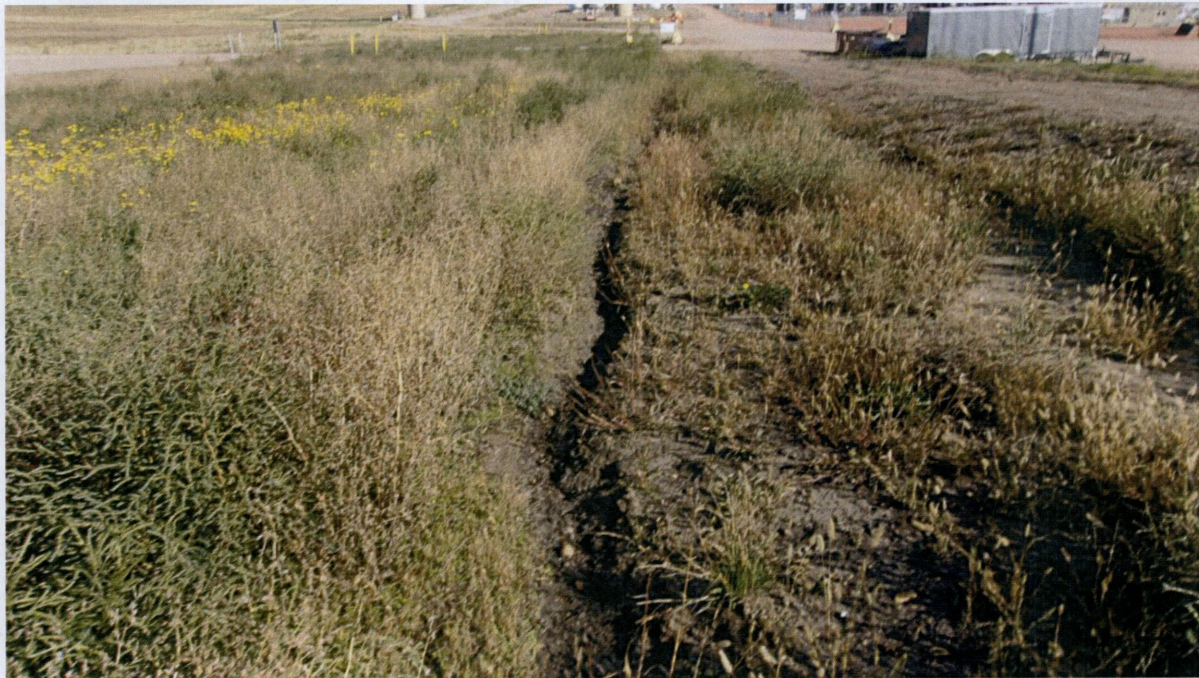
Figure 7. View looking north at an area of erosion along the west side of the truck turnaround access road.
