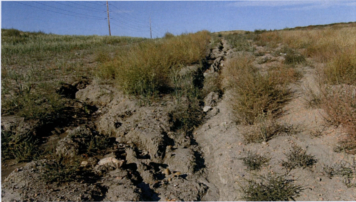
Figure 6. View looking west at an area of significant erosion which starts at the truck turnaround area.
