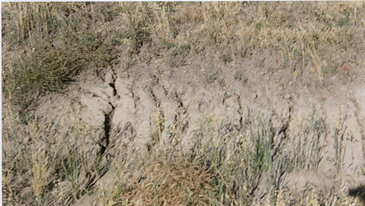
Figure 3. View looking west at the new road ditch with minor soil erosion that is occurring in the road ditch only.
