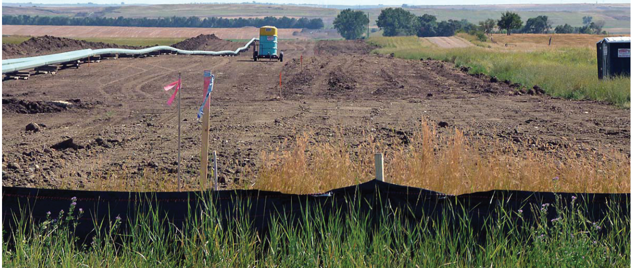
Figure 17. Pipeline construction in corridor of proposed pipeline in August 2011. View is to E. Stake marks proposed pipeline, which continues to the E, into the distance. This is at north terminus of proposed pipeline, at an oil and gas facility. Road to right is 56 th Street NW. Pipeline corridors like this were common throughout the survey area during the 2012 surveys.
