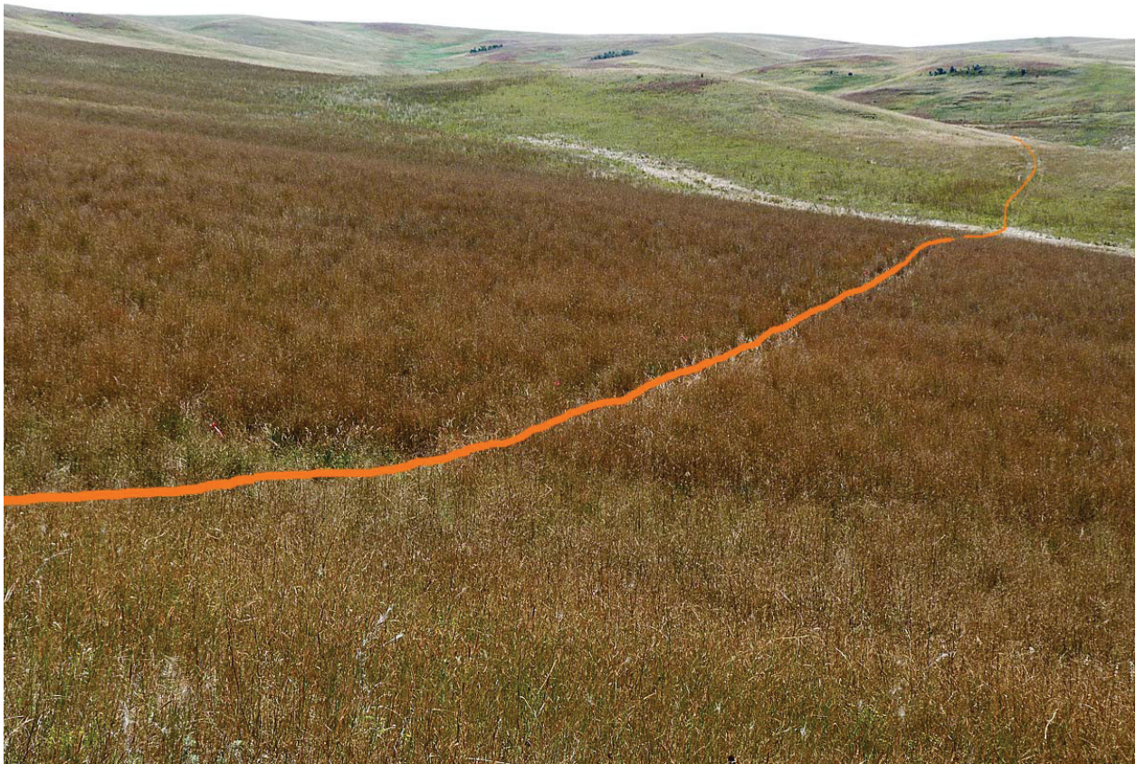
Figure 15. Rust-colored yellow sweetclover dominates this reclaimed grassland. Other clover patches can be seen in distance. Orange line marks proposed pipeline route, an alternate route. View is to SE from Waypoint 149, in T151N, R101W, S21.
