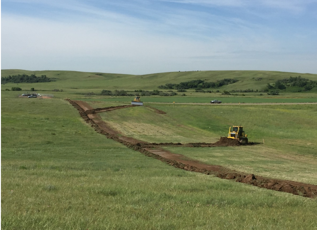
Photo 1. Facing: South. Location: 47.80797, -103.170188. Start of topsoil stripping by Jones Contractors on the North Segment. You can see where the dozer scraped a line in the ground for the topsoil pile to be placed, to stay in the ROW.
