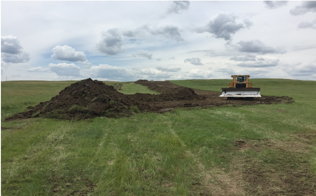
Photo 6. Facing: South. Location: 47.150877, -103.214334. West half of ROW stripped. Final topsoil stockpile location on east end of ROW.
