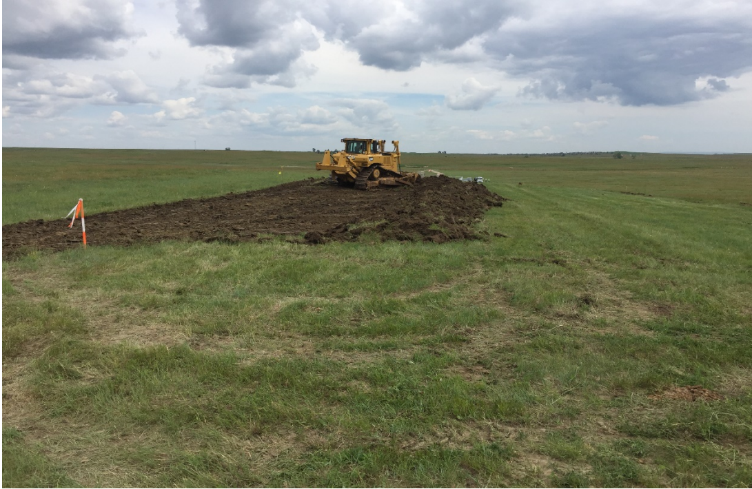
Photo 5. Facing: North. Location: 47.149225, -103.21515. Start of topsoil stripping on South Segment. West half of ROW stripped first.
