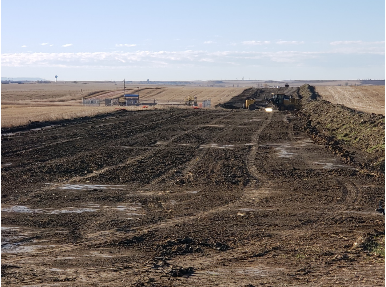
Photo 11. Facing: South. Location: 46.94859, -103.21168. Topsoil stripping on South Segment. Grader making last pass to level ROW.
