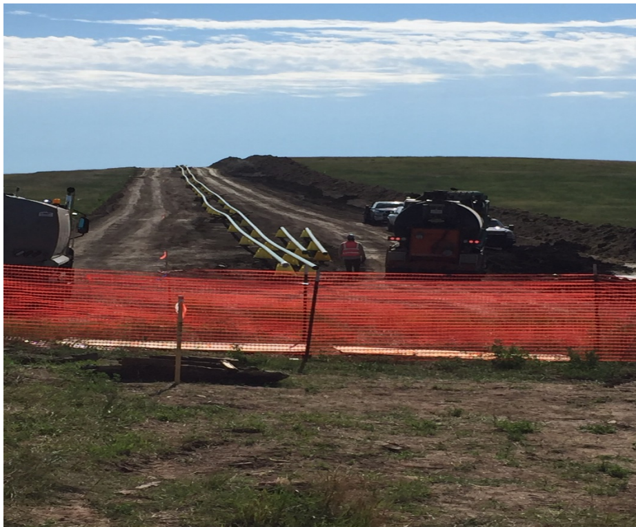
Photo 8. Facing: East. Location: 46.8596, -103.23127. Two stockpile mounds visible at hilltop at the Transfer Segment. Topsoil on outside (right) with the subsoil pile touching.
