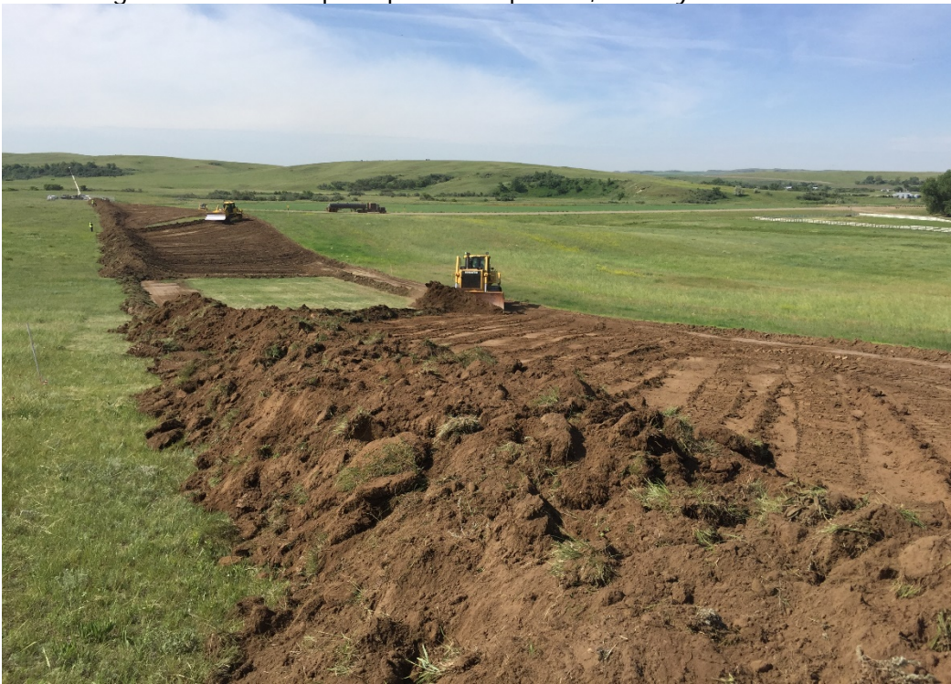
Photo 2. Facing: South. Location: 47.80799, -103.170348. Start of topsoil stripping. Topsoil stockpile being created. Spotters ensuring stockpile remain in ROW.
