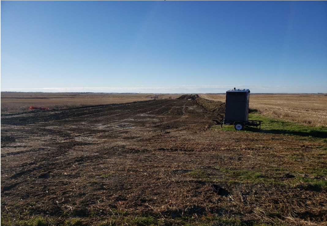
Photo 10. Facing: South. Location: 46.94859, -103.21168. Topsoil stripping on the South Segment. Stockpile stored on west side of ROW.
