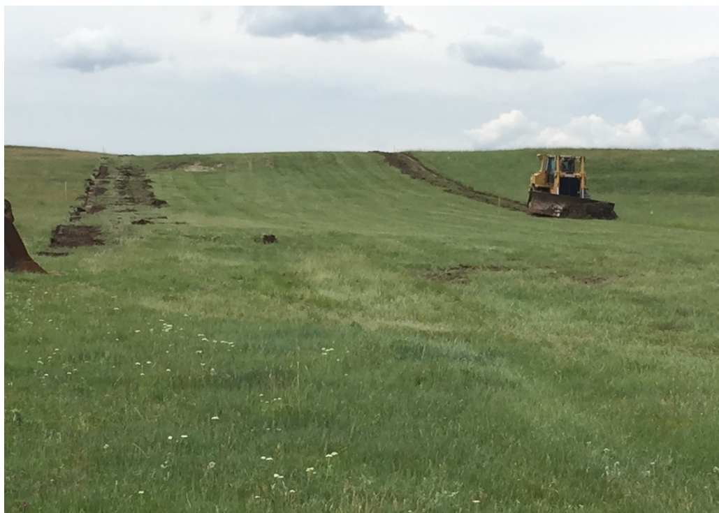
Photo 4. Facing: South. Location: 47.151114, -103.214176. Dozer marking edge of ROW for start of topsoil stripping by Jomax on the South Segment.
