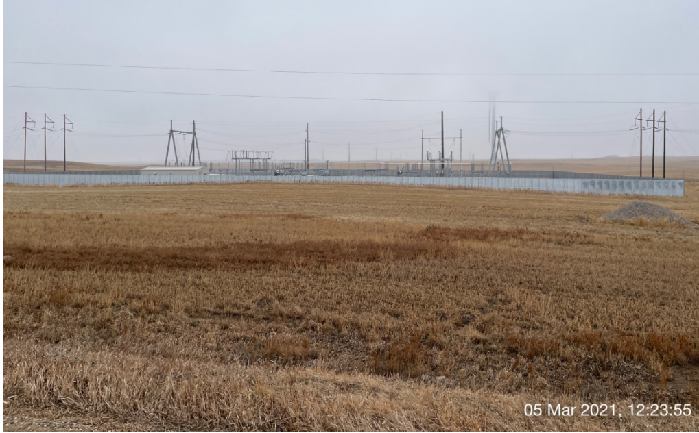
Photo #8: Existing MDU Heskett-Wishek 230 kV Transmission Line
