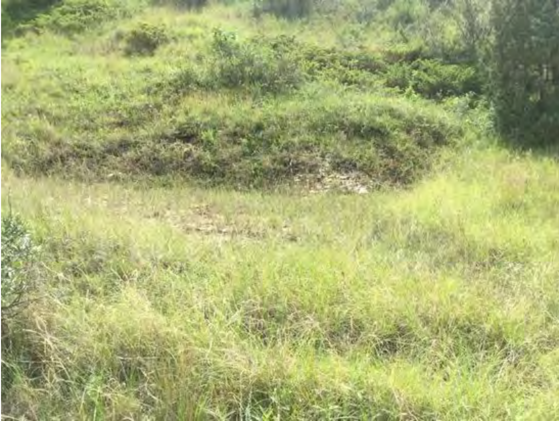
Photo Type: Slope movement evidence | Photo Bearing: 224 degrees Photo Description: Slump near the toe of the slope.
