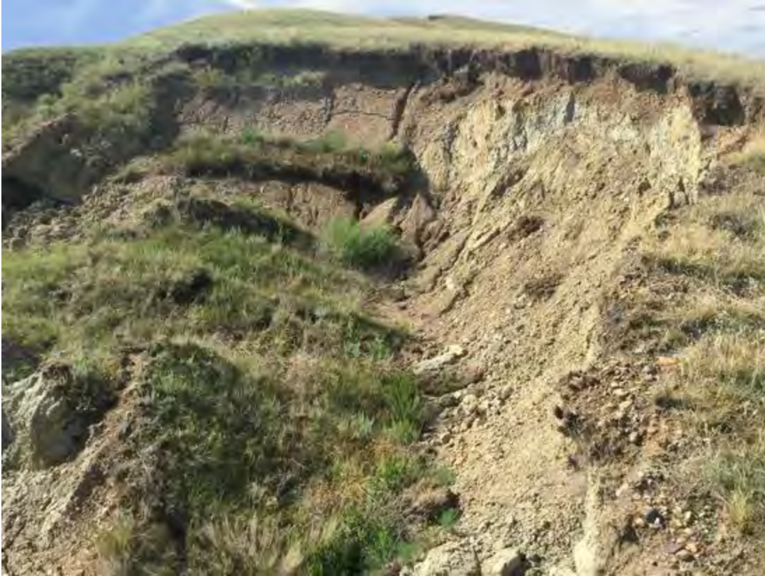
Photo Type: Slope movement evidence | Photo Bearing: 322 degrees Photo Description: Large slide mass between existing pipeline.
