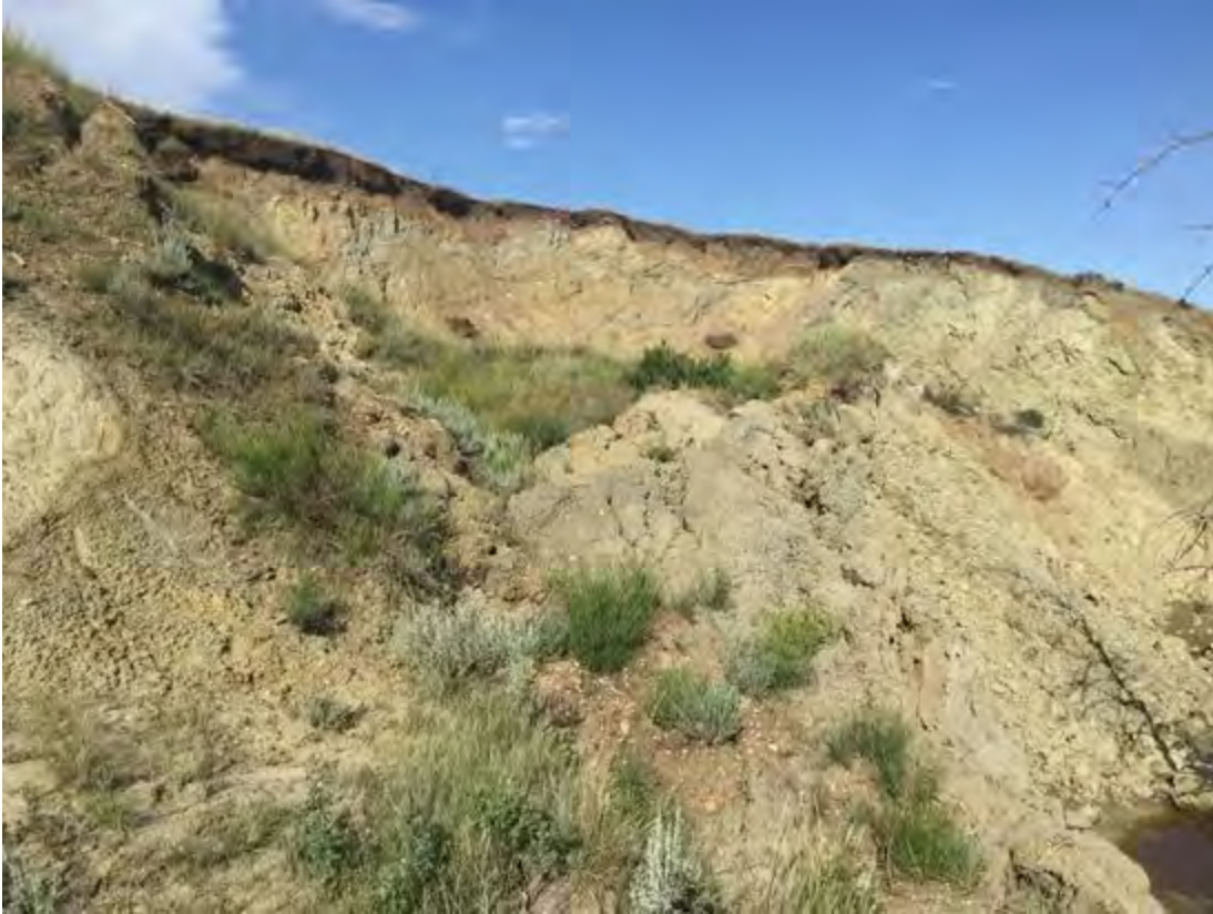
Photo Type: Slope movement evidence | Photo Bearing: 61 degrees Photo Description: Looking upslope at slide mass.
