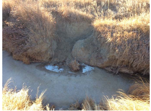
Photo 8: Erosion at waterbody crossing. (Section 4, T147N, R101W)
