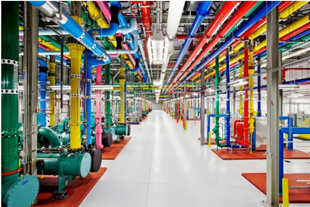
Figure 6 7 A Central Cooling Plant in Google's Douglas County, Georgia Data Center Campus
