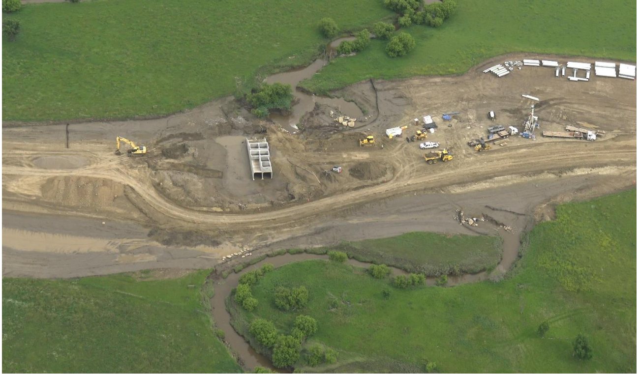
Figure 1- Coyote Creek at access road crossing site taken during June 25, 2015 flyover inspection
