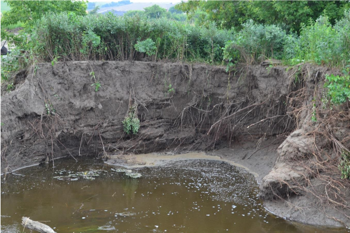
Figure 4- Closer view of bank erosion feature located across from the 60-inch culvert
