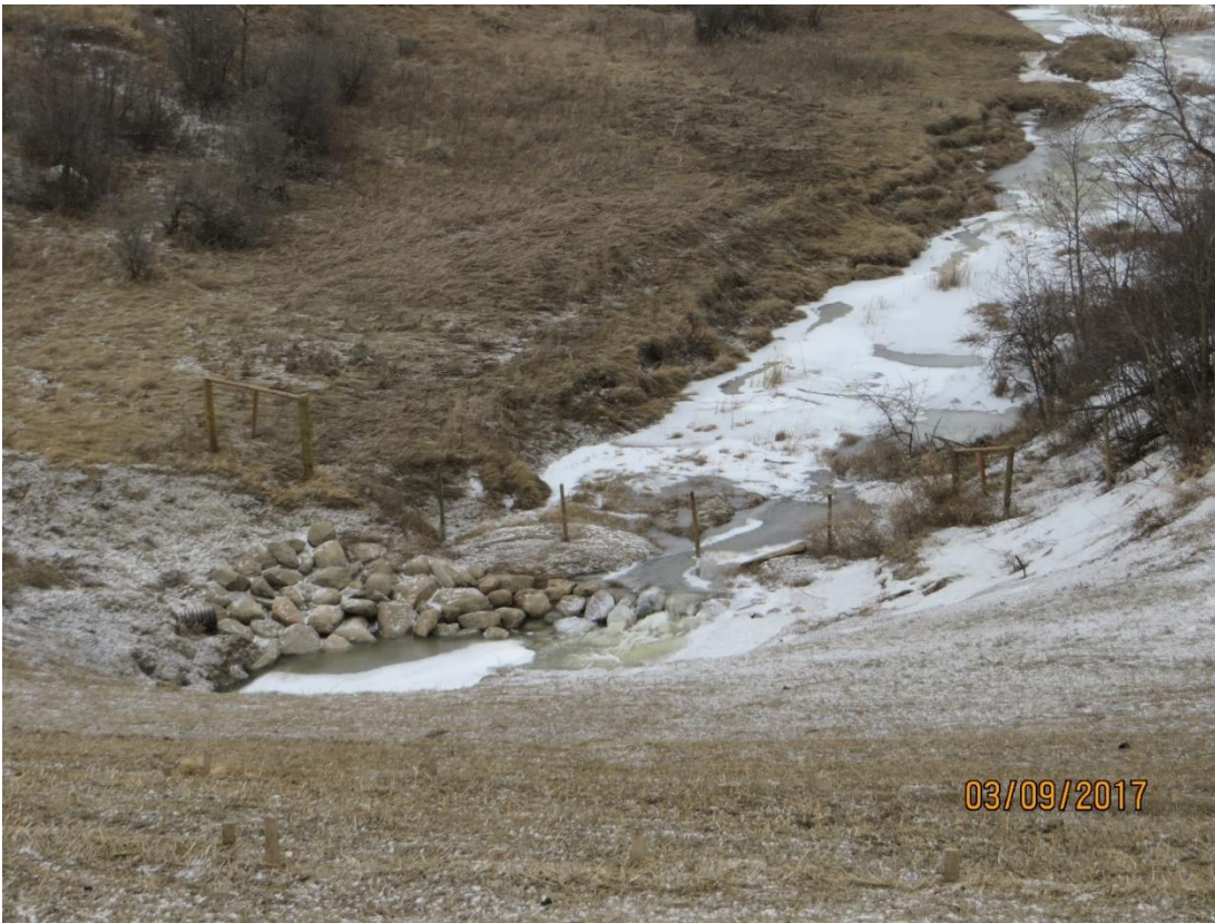
Figure 1. DWC discharge through Section 18 drainage
