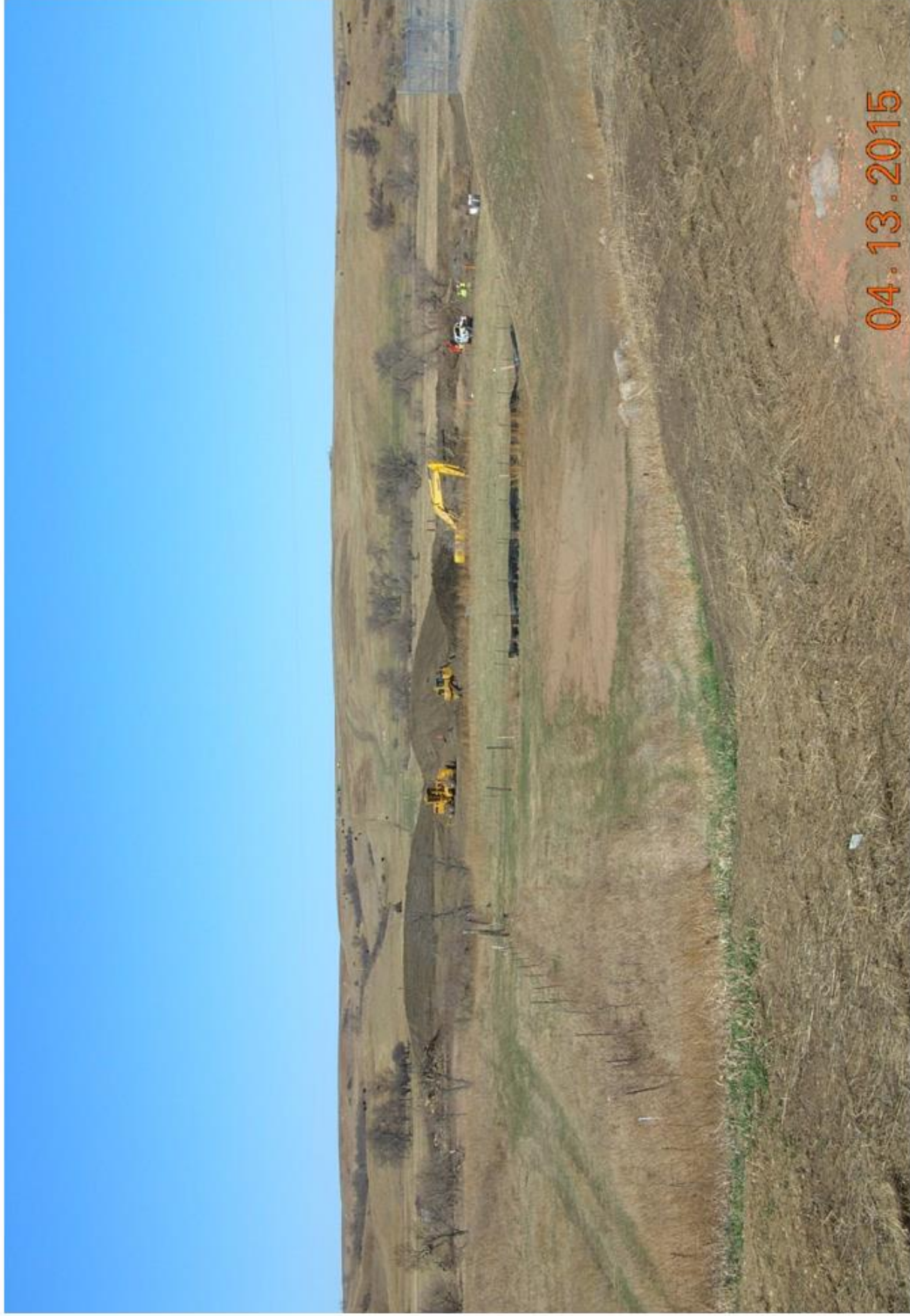
Figure 3. SPGM removal for a four-acre segment of the Shop Access Road on both sides of Coyote Creek with a temporary topsoil stockpile in left background and a temporary subsoil stockpile in middle background – facing west with fence line in center-west marking the section line common to Section 30 on right (north) and Section 31 on left (south) – photograph taken south of large white hoop building pictured in right background in Figure 1
