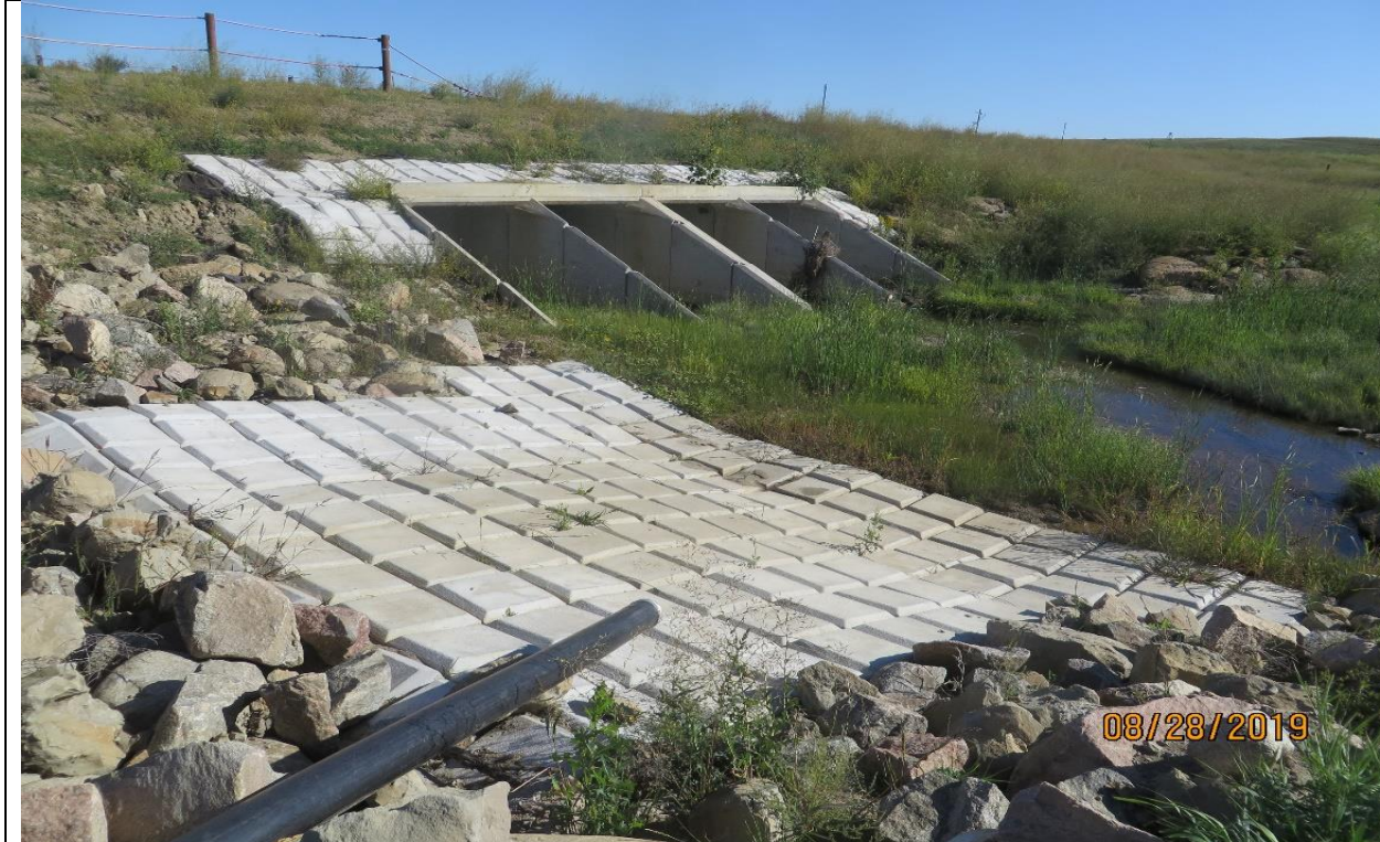
Figure 4: Delta adjacent to west box culvert, south side of the haul road in Sections 30 and 31
