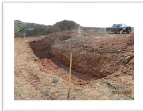
Figure 1. Newly constructed sump between existing sumps No. 1 and 2 View is toward the east
