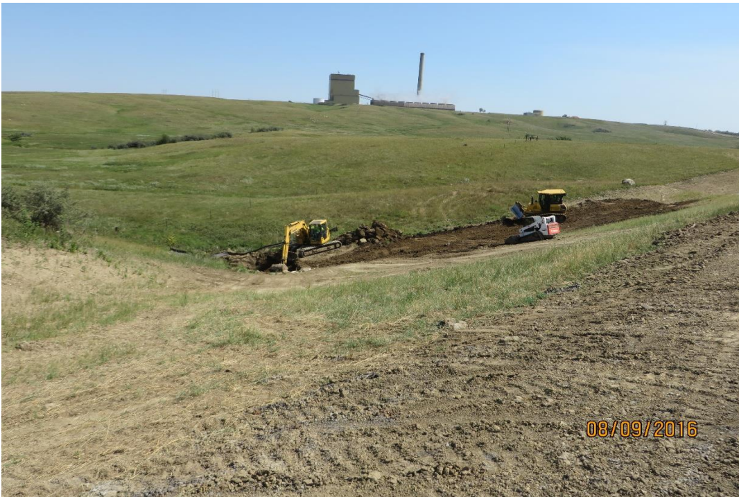
Figure 1. Sump clean-out at Discharge Point No. 6
