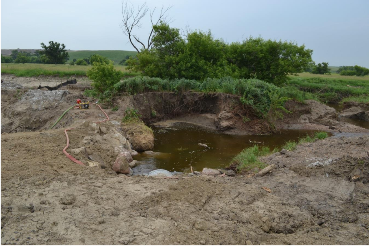
Figure 3- Erosion to stream bank, center. Channel plug and box culvert site to the left.
