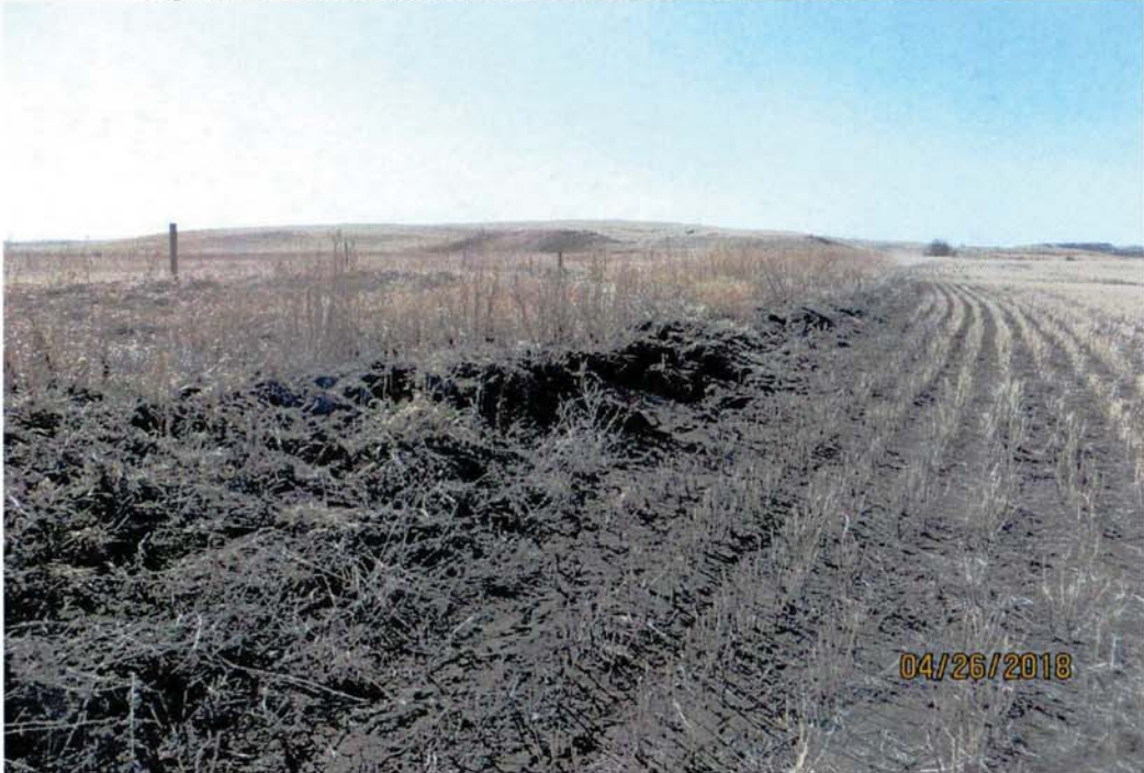
Figure 5: Soil sloughing on the west side of the diversion berm.
