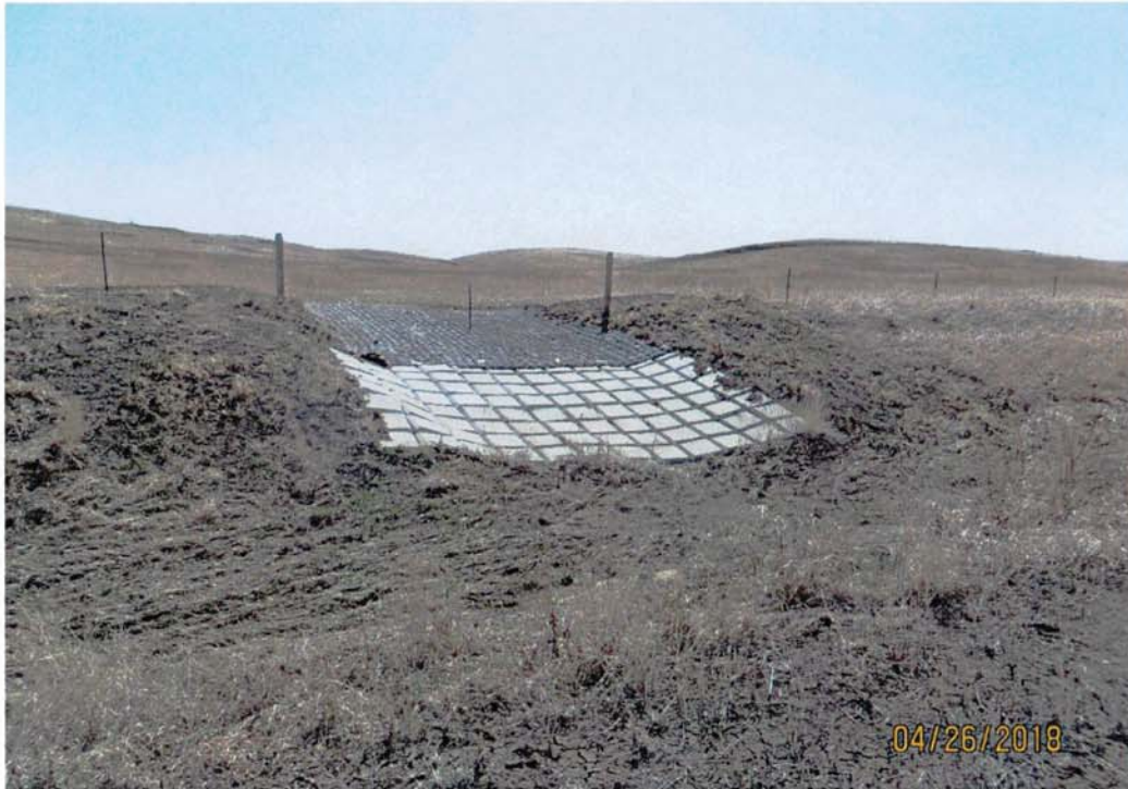
Figure 6. Concrete flex matting at the inlet where water enters the diversion from the NE¼ of Section 34.
