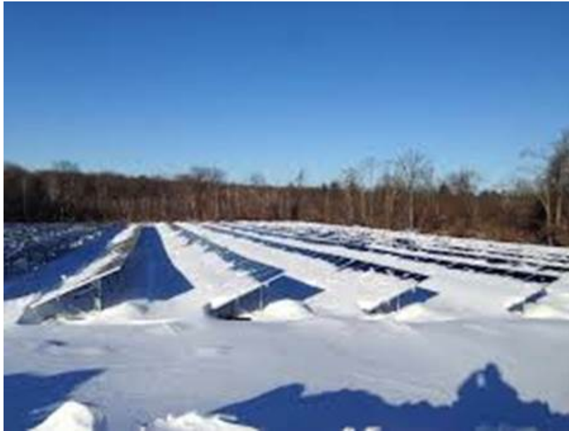
Figure 7: Snow Impacting a Large Solar Installation
