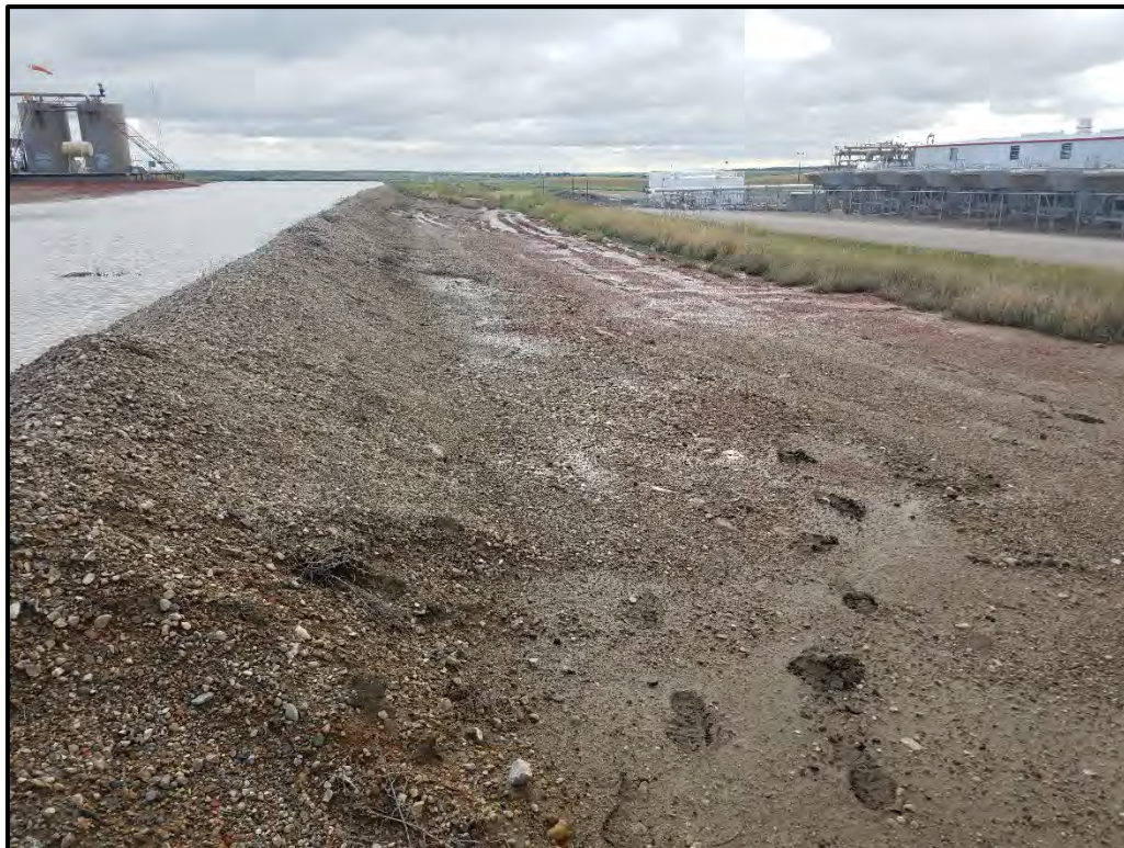
Photograph 2. View looking east from the Facility entrance. Nearly 2 inches of rain fell the night before the survey, resulting in the ponding of water on the pad.
