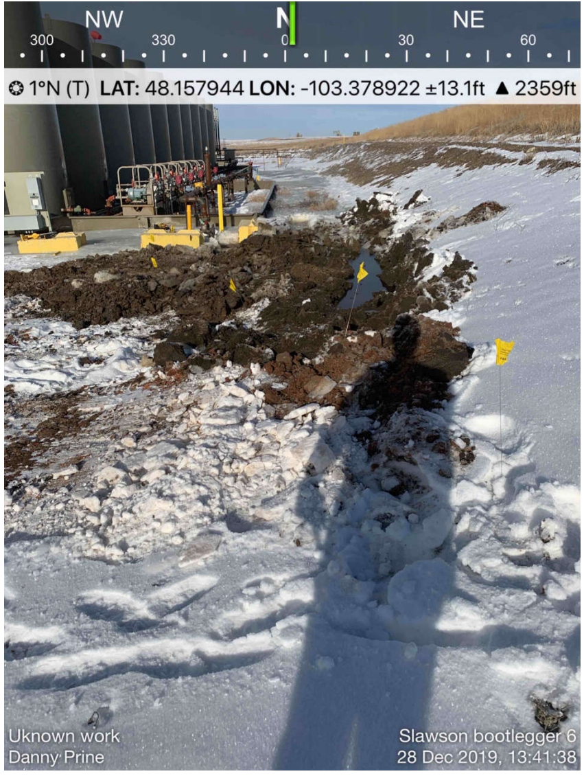
This picture again illustrates the ruts made from when the backhoe fell through the ice and struggled to back out.
