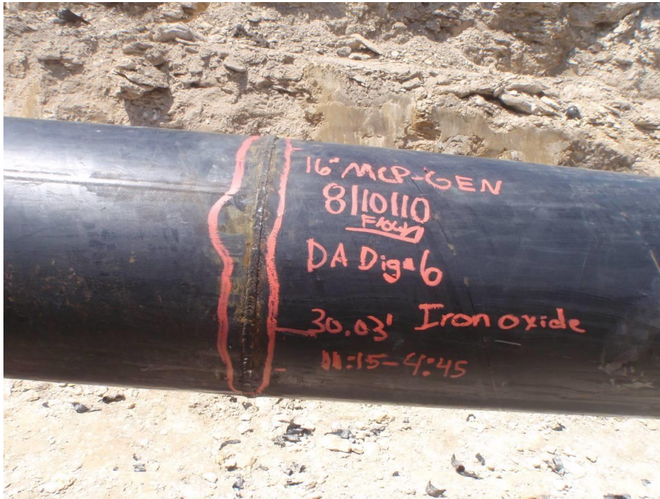
Figure K-4. Example Corrosion Deposit Photograph
