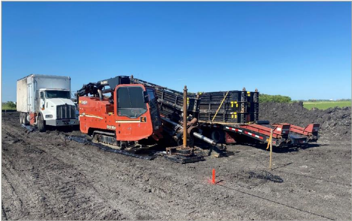
Ditch Witch JT100 Mach 1 HDD Rig and drilling fluid mixing system for HDD at Drain 14
