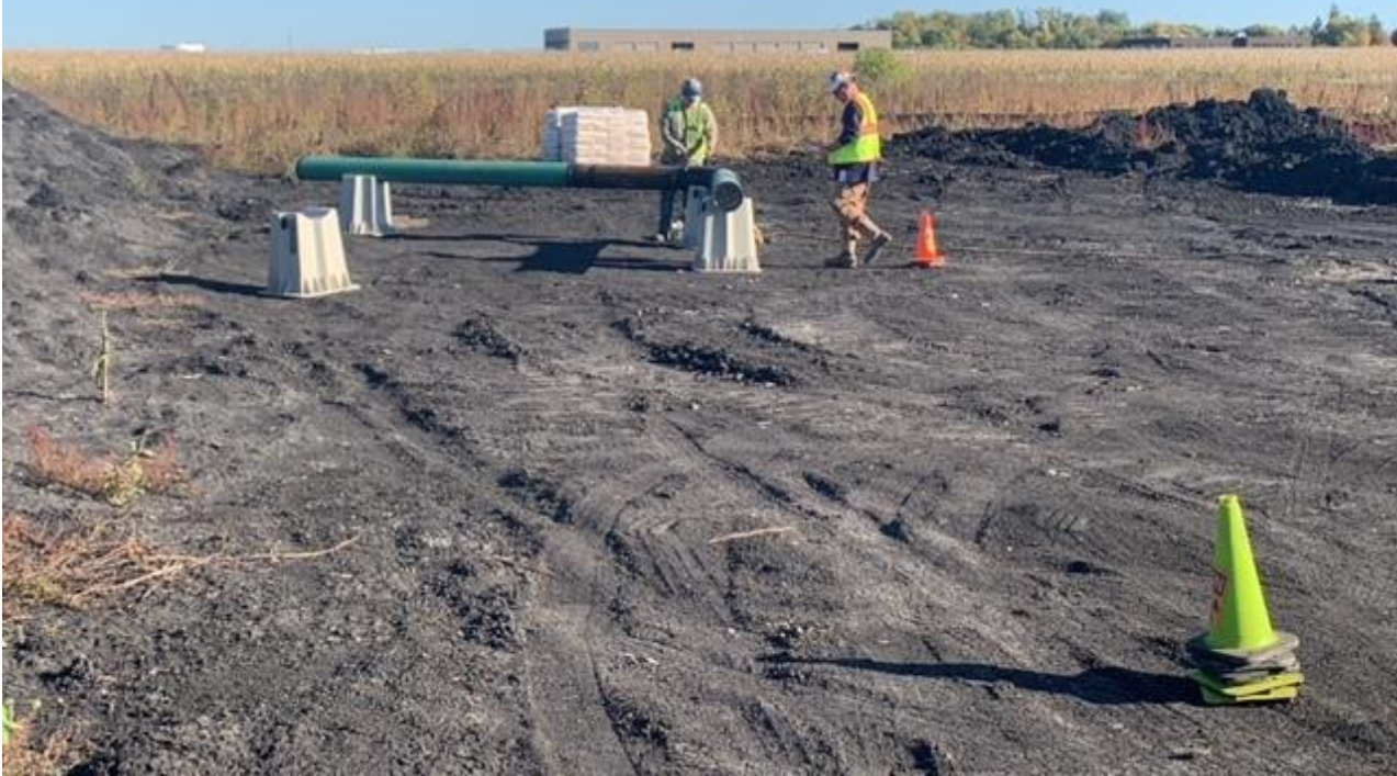
Fabrication of tie-in piping for the westerly end of the relocation project.
