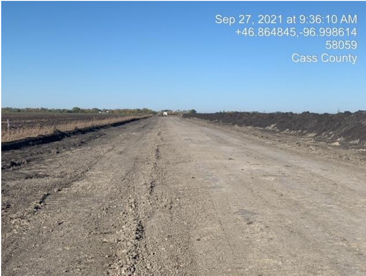
Beginning rough backfill of sub-soil in area where pipeline has been fabricated and installed.
